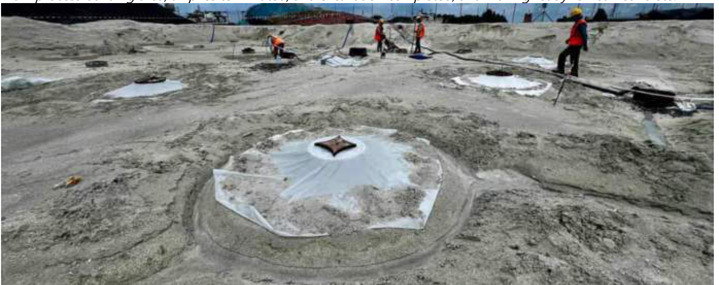
Photo 09 24/10/23 11:17hrs. Main process building area, all piles terminated, and excavation completed, and making ready for lean concrete.
