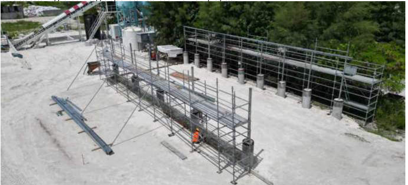
Photo 12 06/11/23 11:19hrs. Concrete batching plant and support facilities installation work is in progress.
