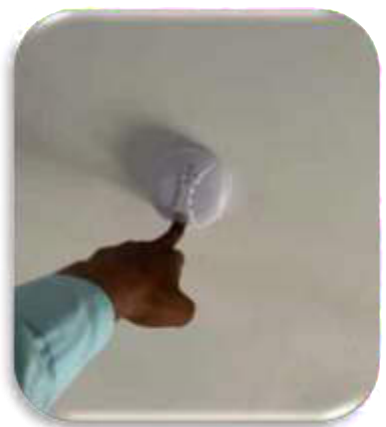
Smoke Detector Inspection
