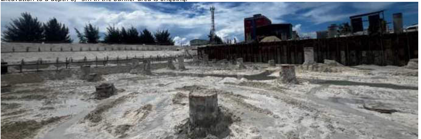
Photo 03 06/11/23 10:49hrs. Excavation to a depth of -5m in the bunker area is ongoing.
