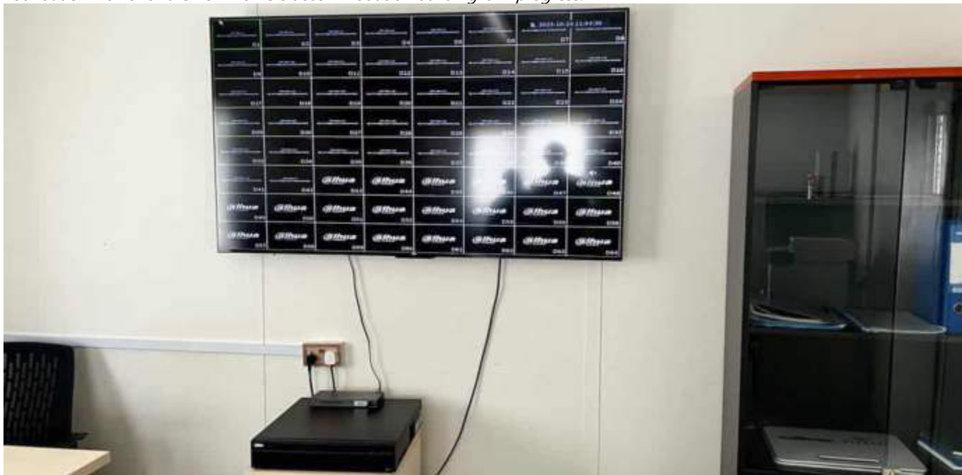
Photo 26 24/10/23 11:19hrs. The CCTV system monitors in the construction camp managers office is not operational at the moment of inspection, issue with the system should be rectified at the earliest. It is recommended to provide monitor for the security guards in the guard.
