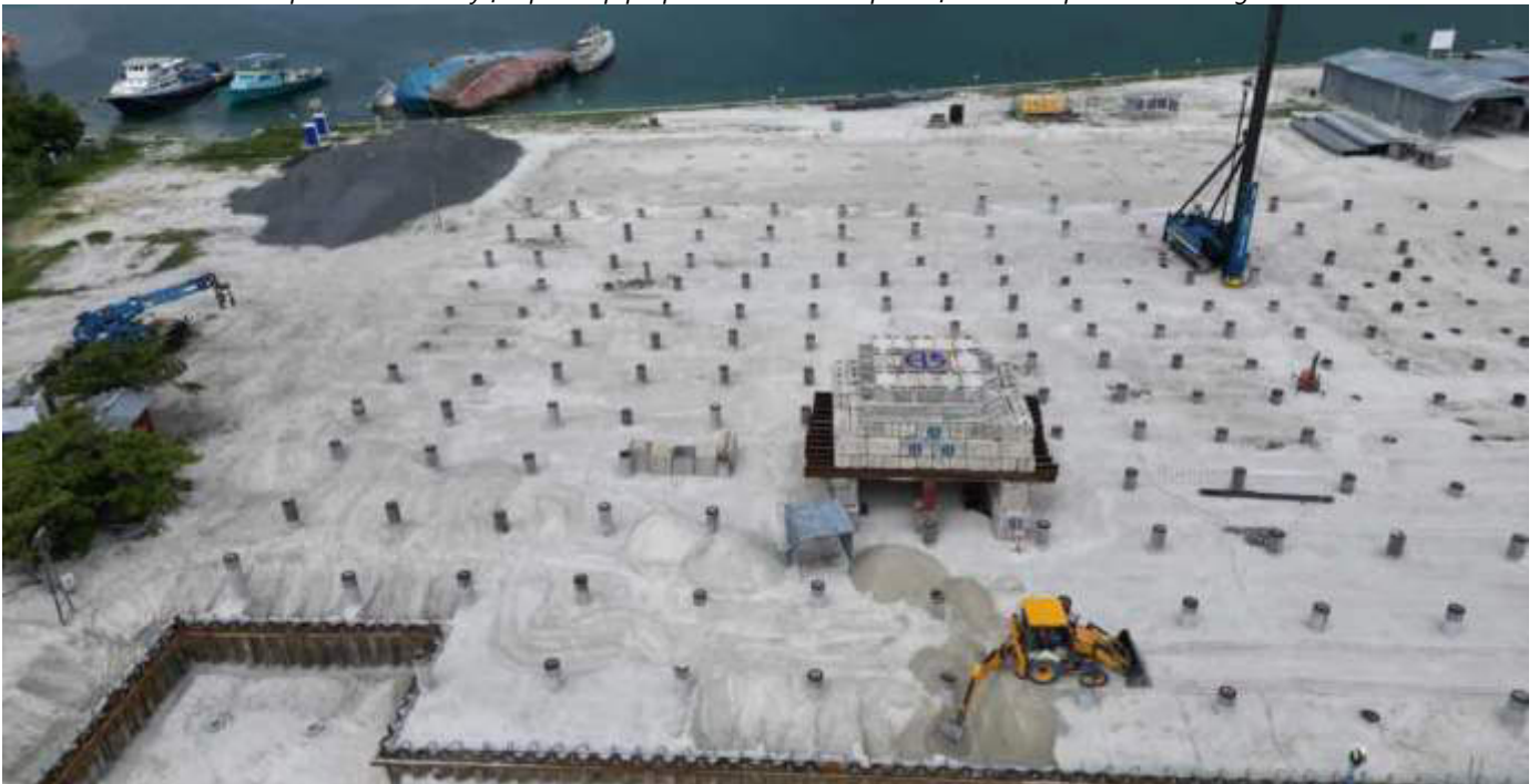
Photo 14 06/11/23 11:19hrs. Static load test being carried out on select piles in the main process building area.
