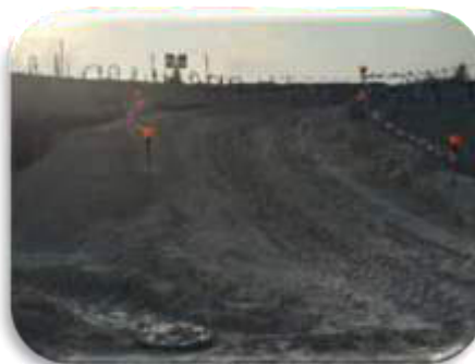
Excavation at the bunker area provided the necessary warning flickering lights and control of entry
