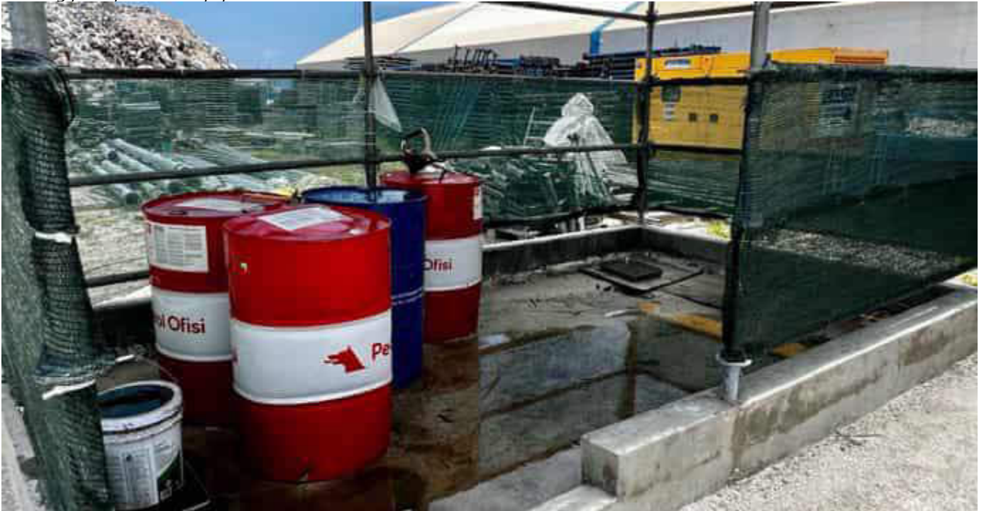
Photo 23 12/10/23 11:36hrs. Fuel storage area, needs to be completed urgently, the containment volume should be checked and ensure proper fire fighting equipment is kept within reach.
