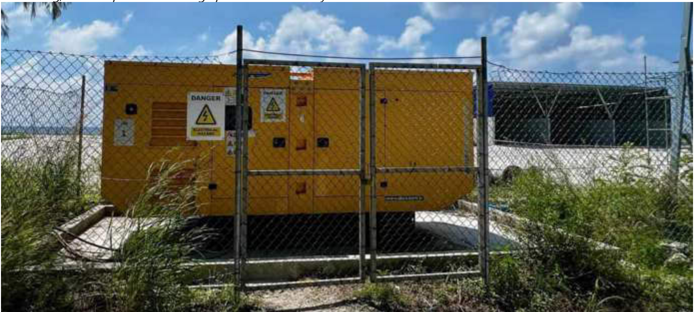
Photo 07 13/12/23 11:30hrs. Diesel genset in use, placed in an enclosure and signage in place. Operational permits have been obtained from URA.
