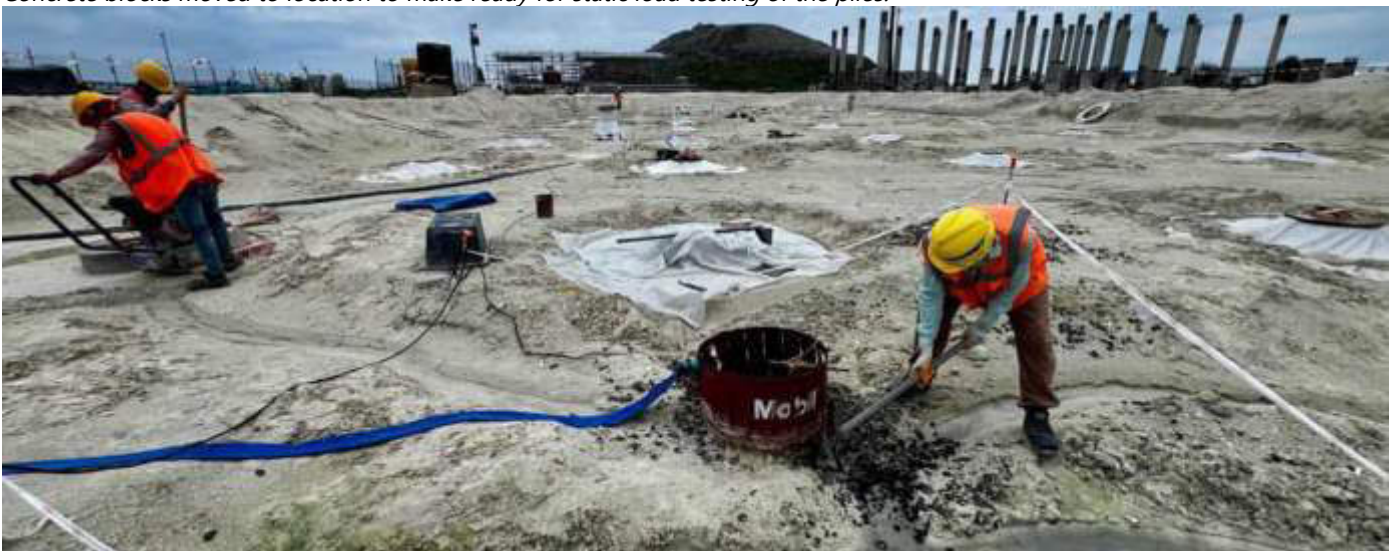
Photo 08 24/10/23 12:10hrs. Main process building area, all piles terminated, and excavation completed, and making ready for lean concrete.
