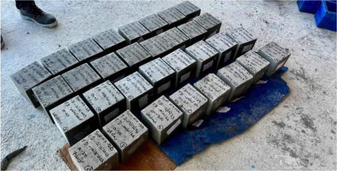
Photo 08 13/11/23 11:47hrs. Concrete batching plant is operational and trial mix test cubes cast and being tested on site by the ELS concrete testing lab.
