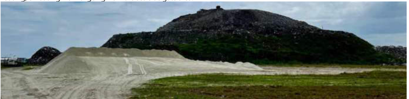
Photo 12 24/10/23 11:19hrs. Excavated soil from the site is stored in the laydown area within the site boundary.
