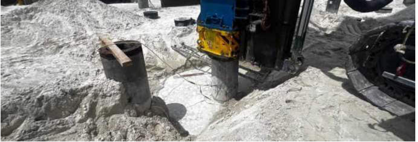
Photo 04 06/11/23 10:50hrs. PDA test being conducted on select piles in the main process building area.
