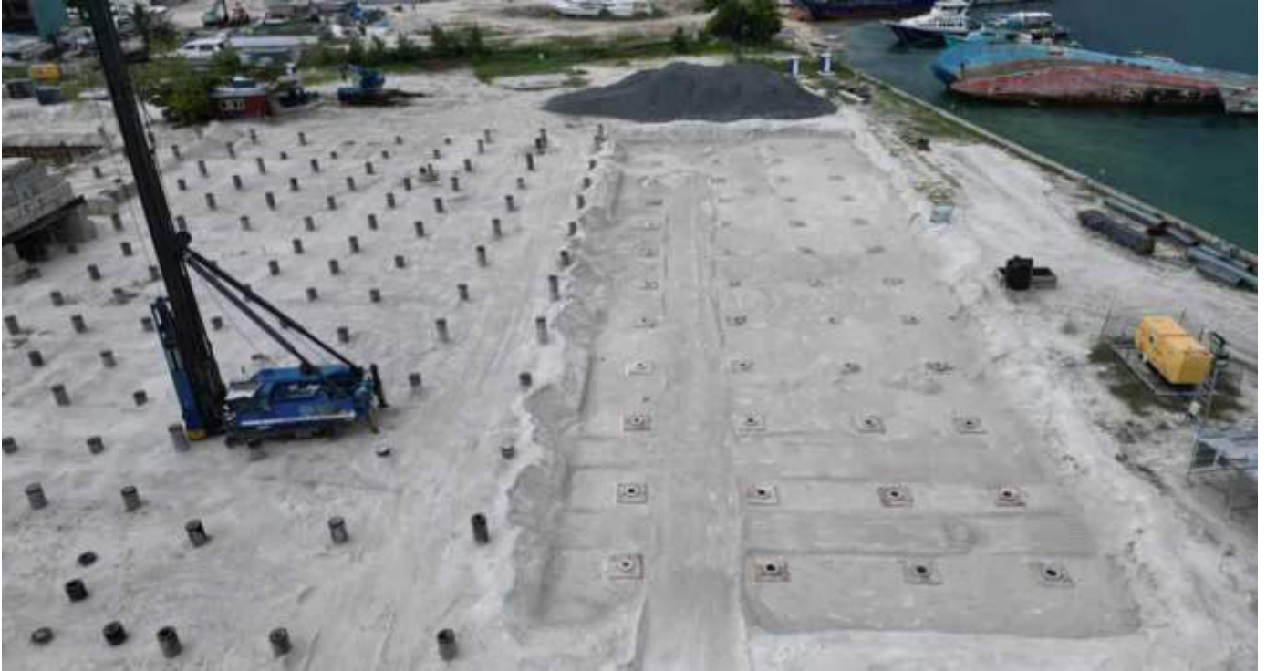
Photo 13 06/11/23 11:19hrs. Lean concrete works completed and ready for pile cap preparation works in part of the main process building.
