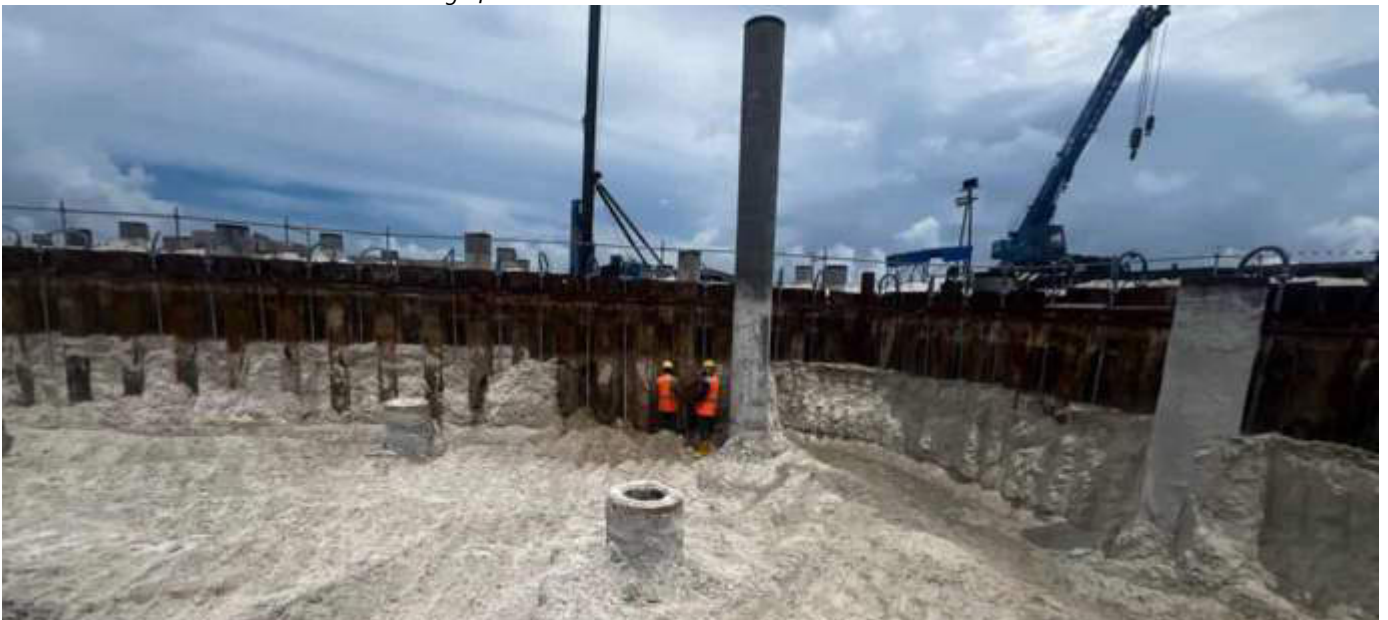
Photo 02 by 06/11/23 10:48hrs. Excavation to a depth of -5m in the bunker area is ongoing.
