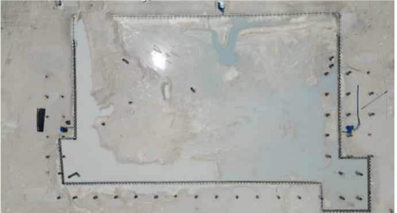
Photo 07 12/10/23 11:00hrs. Bunker area has been sheet piled and the wellpoint dewatering system installed, excavation has started.
