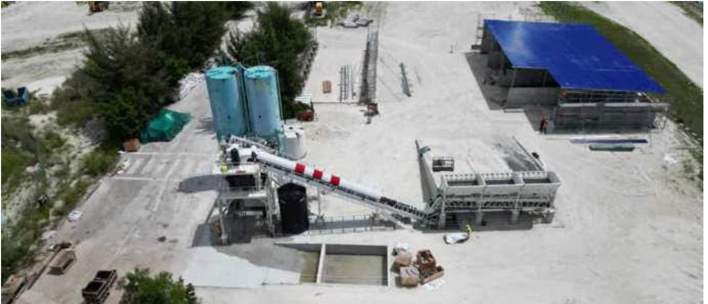
Photo 11 06/11/23 11:19hrs. Concrete batching plant and support facilities installation work is in progress.
