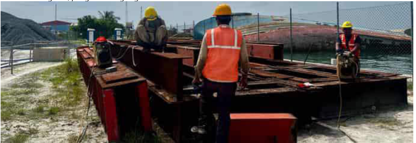
Photo 46 12/10/23 12:08hrs. Fabrication of the framing to be used for static load testing of the spun piles ongoing.
