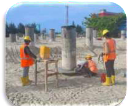
workers are all PPE (dust mask, hearing protection etc.) Compliance while cutting of spun pile
