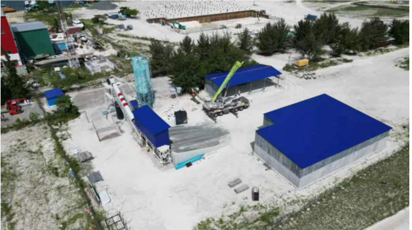
Photo 12 13/12/23 13:05hrs. Concrete batching plant is operational and support facilities installation work is in progress.
