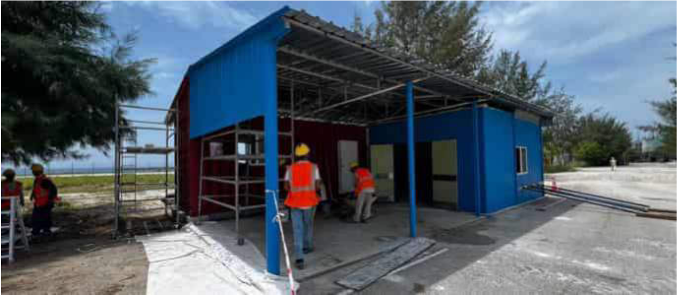
Photo 13 12/10/23 11:22hrs. Concrete testing lab under construction close to the batching plant setup within the site boundary.
