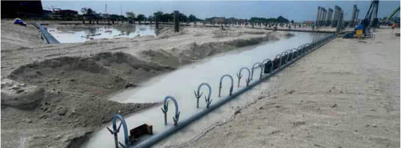
Photo 40 12/10/23 11:59hrs. Well point dewatering system installed in place around the bunker area and ready to be used.
