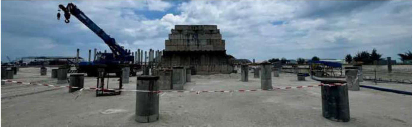
Photo 07 24/10/23 11:05hrs. Concrete blocks moved to location to make ready for static load testing of the piles.
