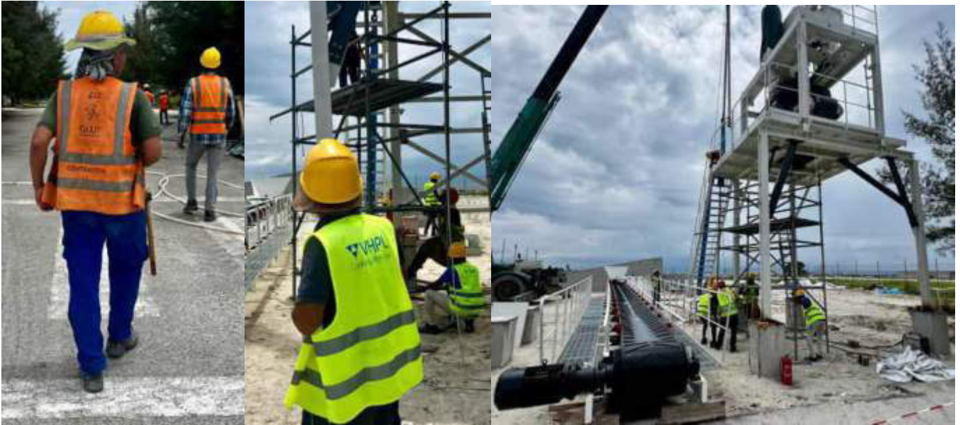
Photo 30 24/10/23 11:19hrs. Workers from GLUT and VHPL on site. All subcontractors should be approved by ER.
