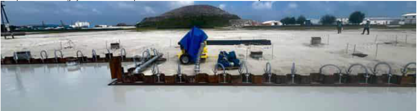
Photo 41 12/10/23 11:59hrs. Well point dewatering system installed in place around the bunker area and ready to be used.
