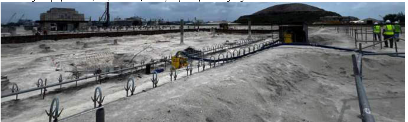
Photo 03 06/11/23 10:49hrs. Continous dewatering of the bunker area is ongoing, as excavation works continue.
