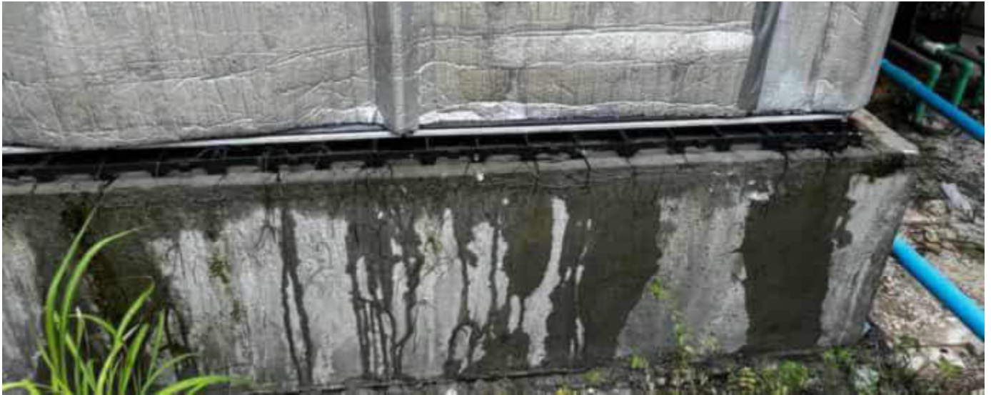
Photo 29 12/10/23 11:44hrs. The main storage tank still leaks at several places, and this issue has not been rectified after several months.
