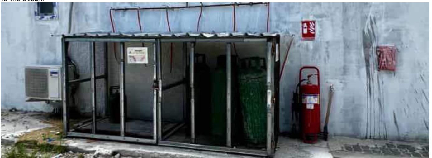
Photo 33 12/10/23 11:49hrs. Cooking gas storage kept locked and fire fighting equipment on hand.
