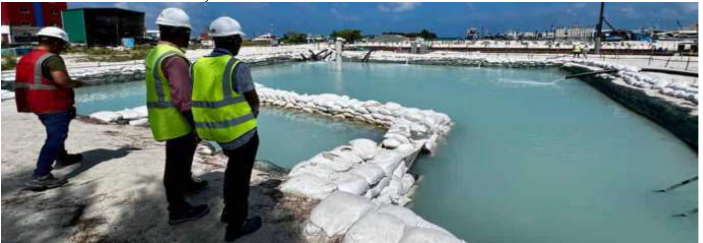
Photo 06 13/12/23 11:25hrs. Sedimentation pond for the dewatering activities. Kept clean and any floating debris is removed regularly. Life buoys placed and a guard is always posted. Dewatering will continue until foundation works have been completed. Regularly dewatering water quality monitoring, and EPA permits are being updated on a monthly basis.
