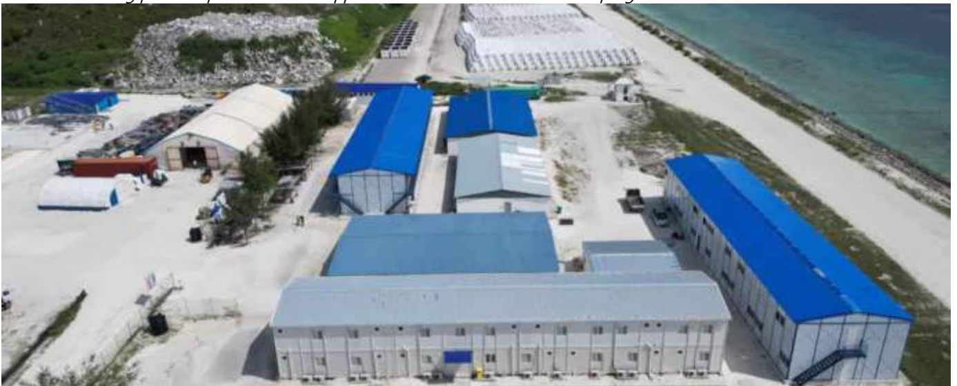
Photo 13 13/12/23 13:09hrs. Workers camp on site (Right) a new workers accommodation block and a staff accommodation block is almost complete.
