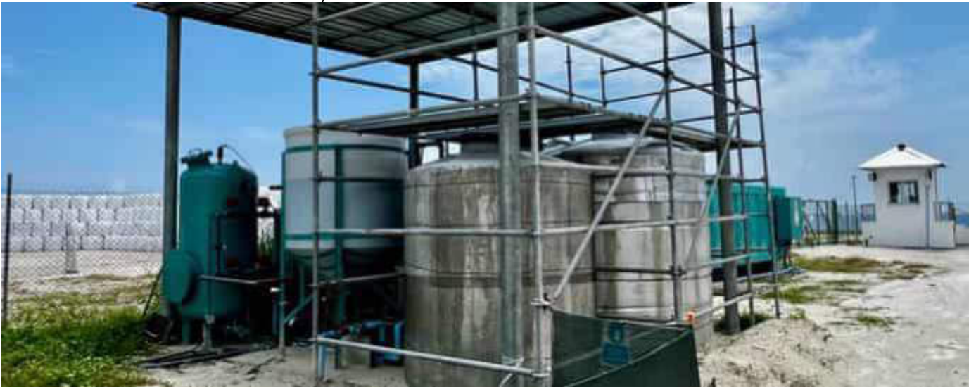
Photo 32 12/10/23 11:48hrs. Waste water treatment plant is operational and in use. Periodic testing is done to ensure the water is safe enough to be pumped to the ocean.
