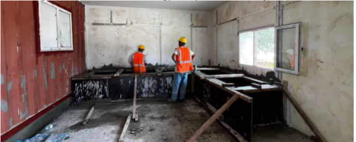
Photo 14 12/10/23 11:23hrs. Concrete testing lab under construction close to the batching plant setup within the site boundary.
