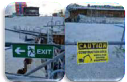
Appropriate mandatory signage placed at the worksite
