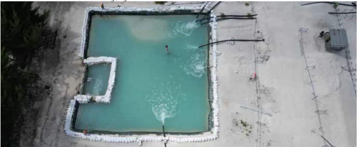
Photo 17 06/11/23 13:26hrs. Dewatering works is ongoing and the sedimentation tank kept with guard rails, silt traps, and guard in place and all surface debris is removed before the outfall.
