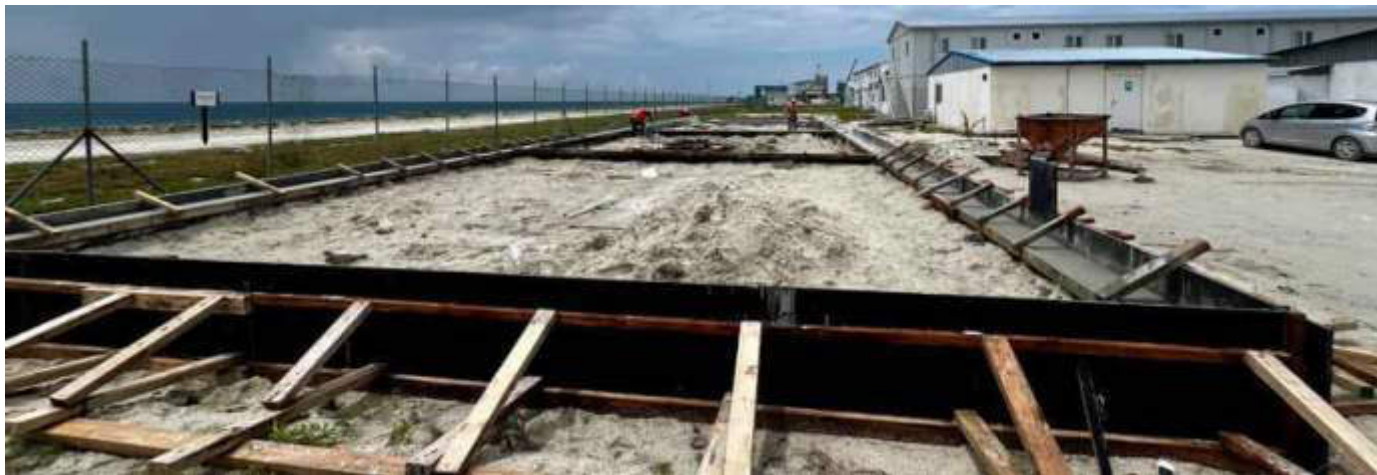
Photo 25 24/10/23 11:19hrs. Foundation works for the new workers accommodation building is in progress.
