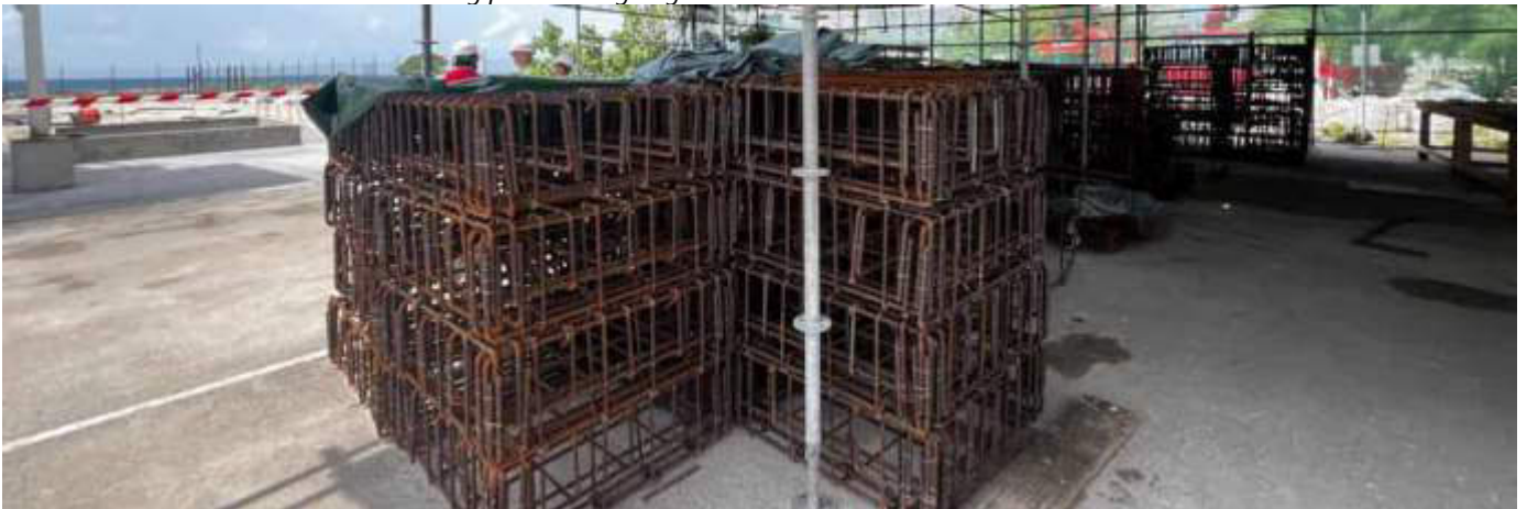
Photo 02 by 06/11/23 10:48hrs. Barbending and preparation of reinforcement for the spun pile caps are ongoing.
