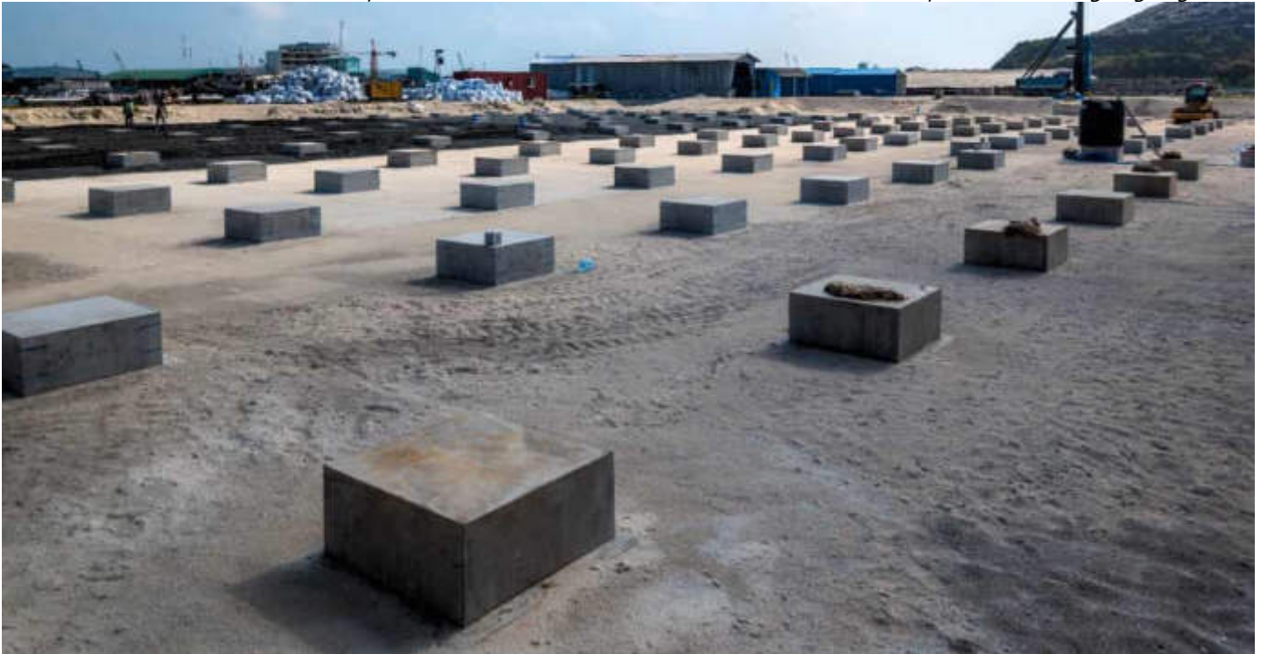
Photo 05 13/02/24 – Main process area, pile cap concrete works completed where possible and backfilling works in progress.
