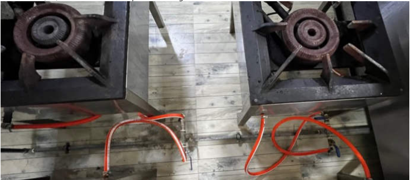
Photo 28 15/01/24 – Gas stoves are used in the kitchen and gas is piped from outside storage to the stoves.
