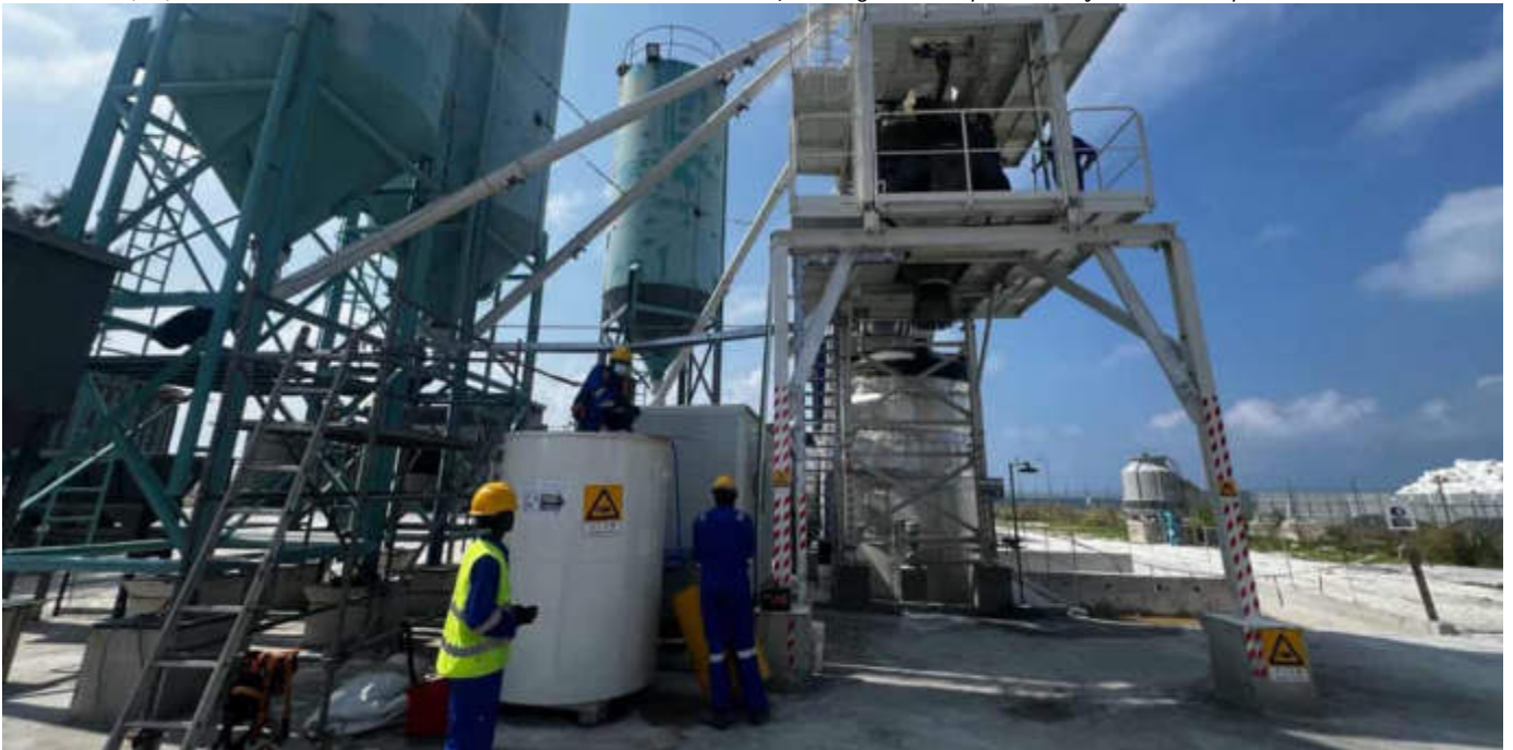
Photo 12 06/03/24 – Concrete batching plant is operational and operated by the subcontractor Villa Pvt. Ltd.
