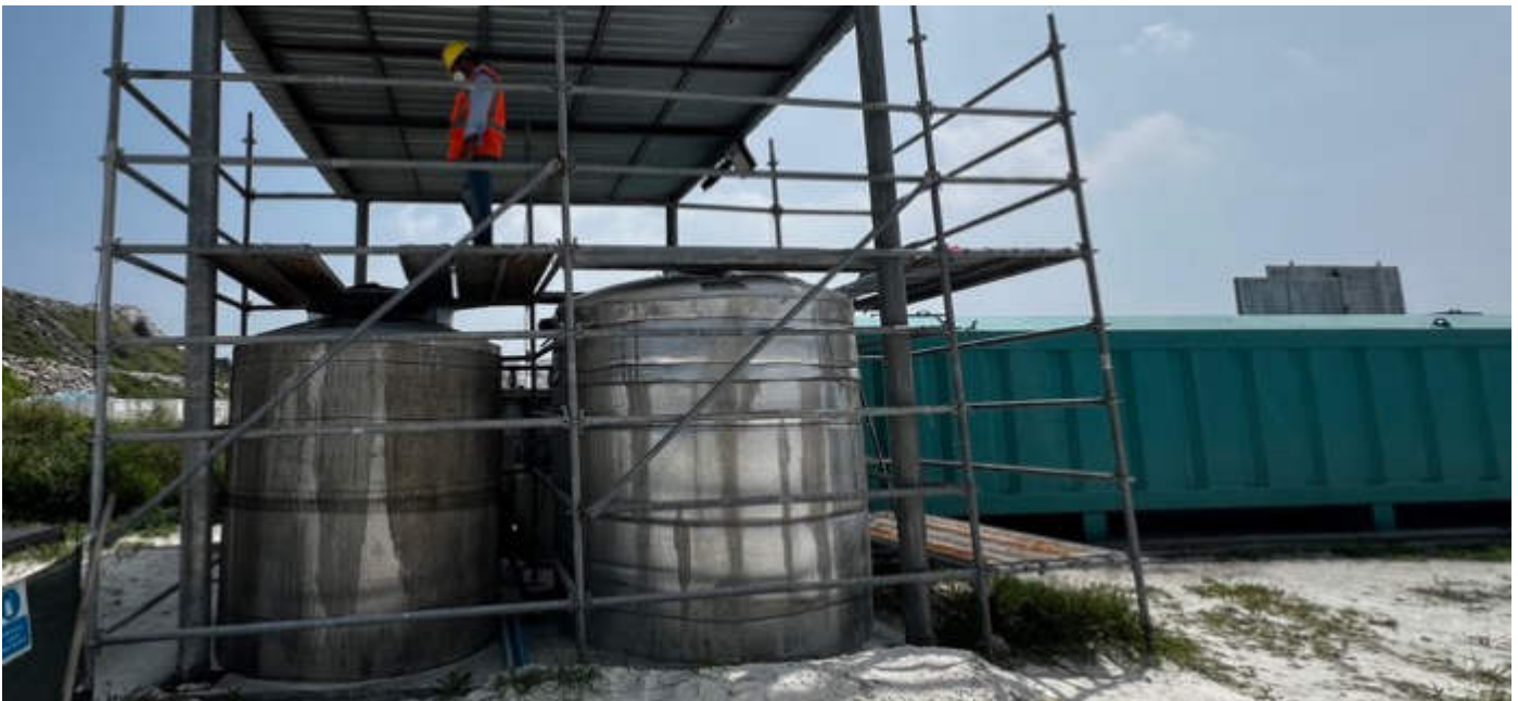
Photo 26 15/01/24 – Waste water treatment plant is operational and well maintained and monitored monthly.
