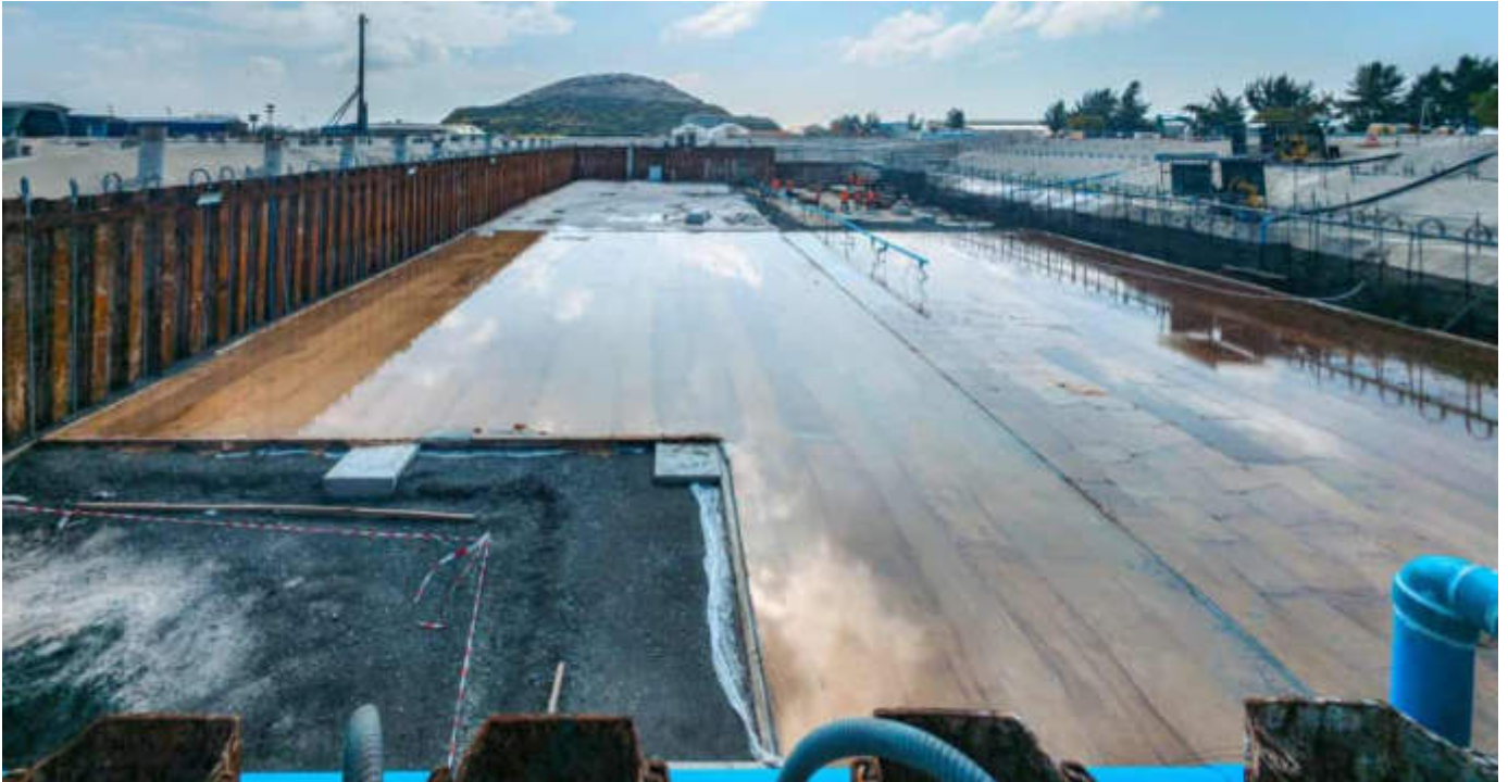
Photo 04 13/02/24 – Bunker area, part of the lean concrete for the foundation has been completed, and curing ongoing.
