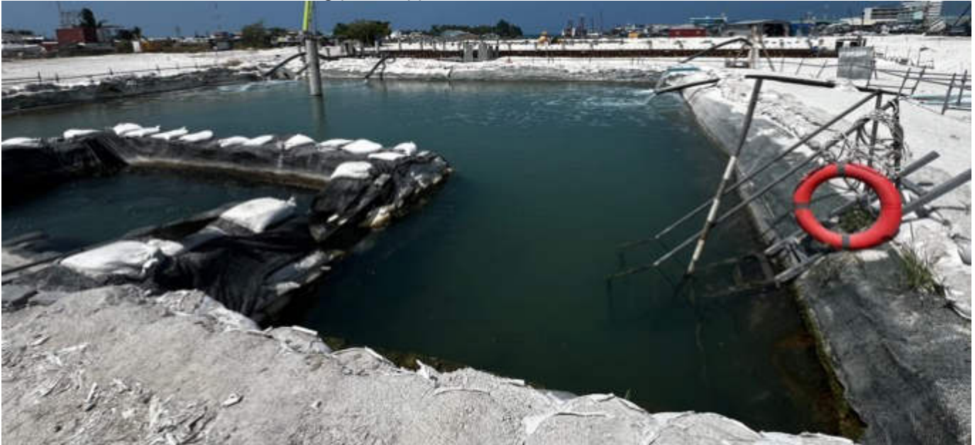
Photo 43 17/01/24 – Dewatering sedimentation pit is kept clean and guard placed at all times.
