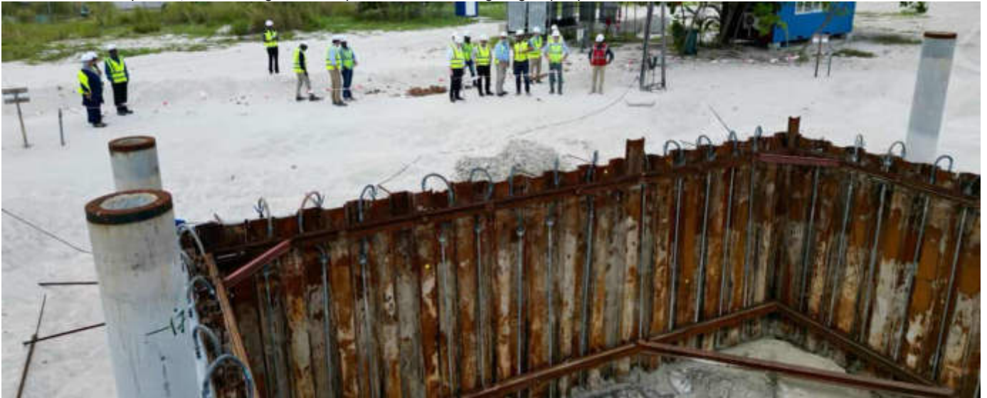
Photo 15 27/02/24 – DAB team members on site with the team members from DBO, EPC, PMU, PMDSC during the site walk about at the leachate pit area in the waste bunker area.
