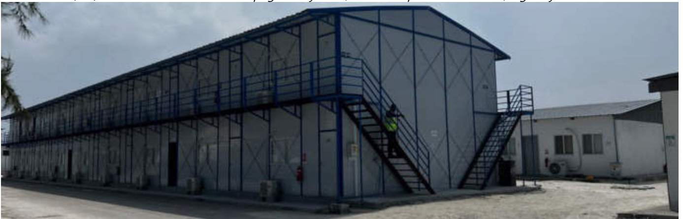
Photo 20 15/01/24 – Staff accommodation building is nearly completed, MNDF fire safety inspections carried out.
