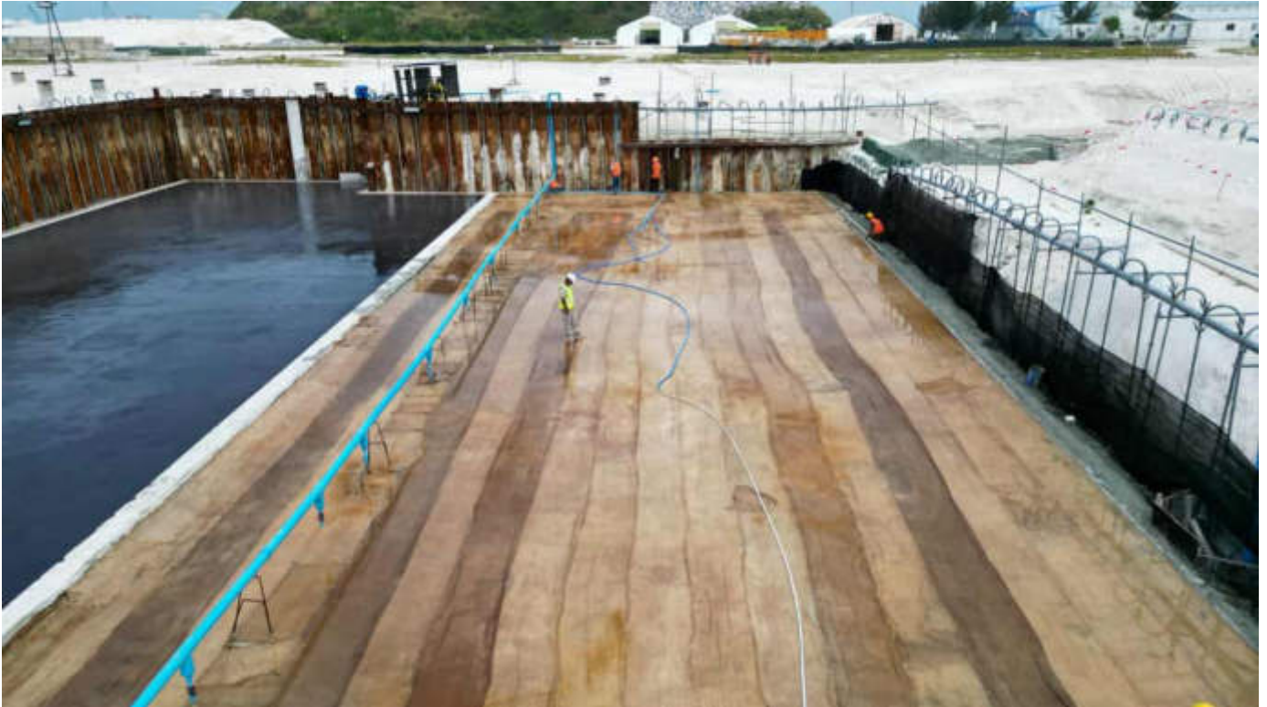
Photo 17 27/02/24 – Waste bunker area, lean concrete works completed, and curing ongoing (right side), waterproofing layer completed (left side)
