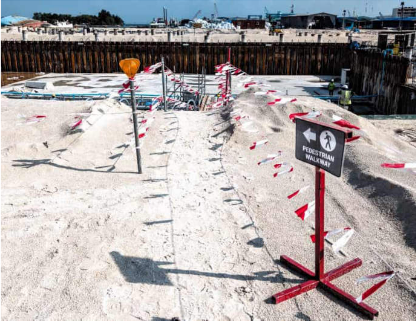
Photo 02 13/02/24 – Dedicated pedestrian walk way to access bunker area established for workers safety.
