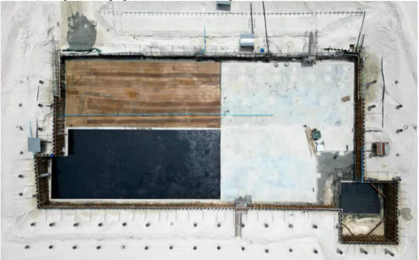
Photo 20 27/02/24 – Waste bunker area, sheet piling completed, excavation completed, continuous dewatering ongoing, spun pile installation completed, pile cap concrete works completed, backfilling and compaction completed, lean concrete work completed. Water proofing layer installation works in progress, leachate pit (bottom left corner) water proofing layer completed. Concrete works will start from the leachate pit.
