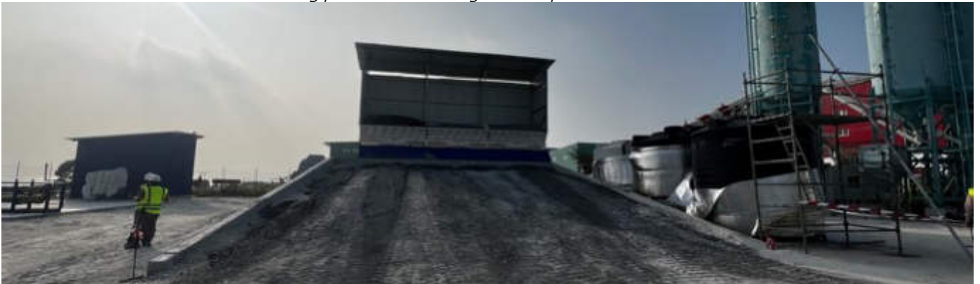
Photo 16 15/01/24 – Concrete batching plant material tipping area, kept covered from wind and rain.
