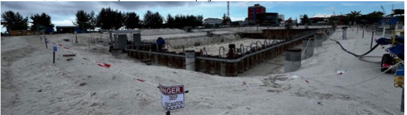
Photo 04 03/01/24 – Bunker area seen here, the safety tape and barrication around the excavation needs to be improved.
