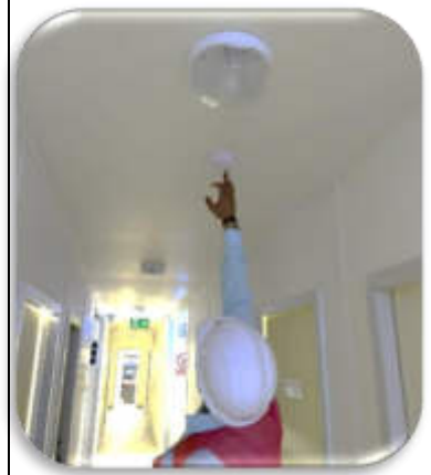
Smoke Detector Inspection
