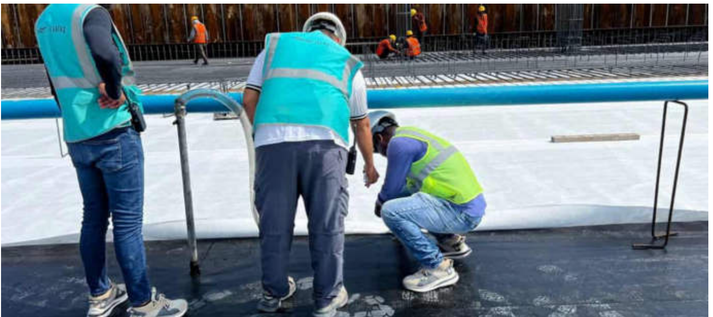
Photo 09 06/03/24 – Sathya from DBO conducting inspection of the geomembrane installation in the bunker area.
