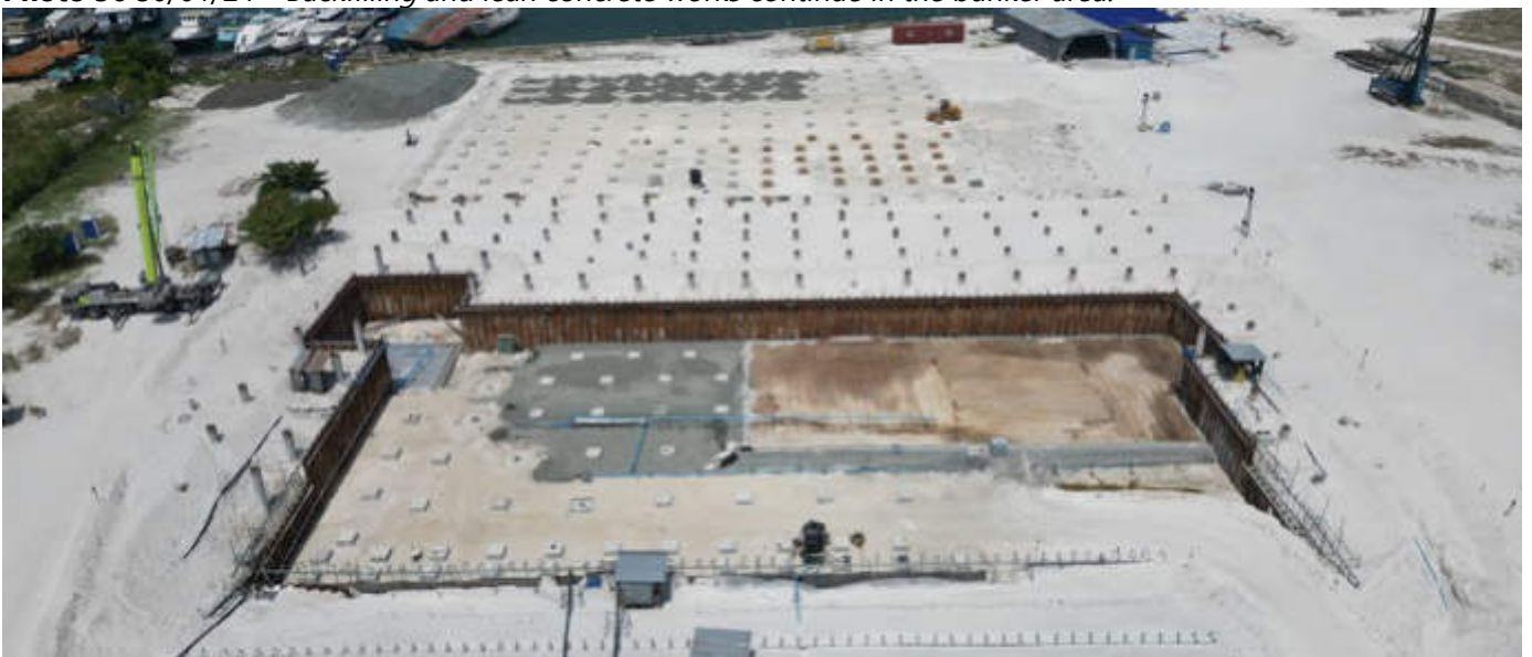
Photo 57 30/01/24 – Overall construction area view, backfilling and pile cap concrete works continue in the main process building area.
