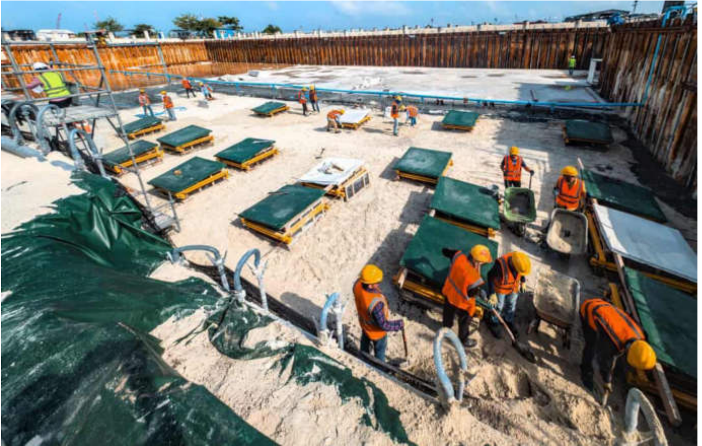
Photo 06 13/02/24 – Bunker area preparation for pile caps cast and curing on going for part of the bunker.
