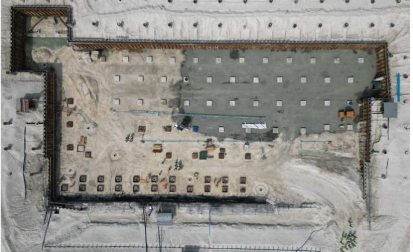
Photo 47 17/01/24 – Bunker area top view, backfilling work and pile cap concrete works in progress.
