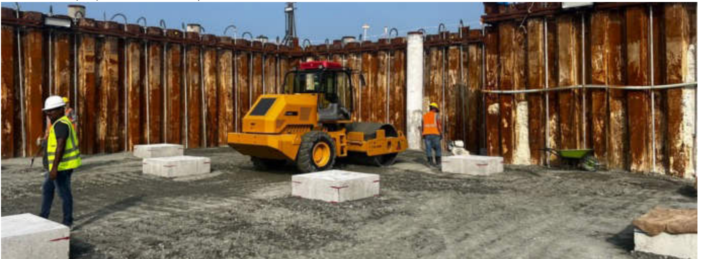
Photo 09 15/01/24 – Backfilling and compaction work on going in the bunker area where the pile cap concrete works have been completed.
