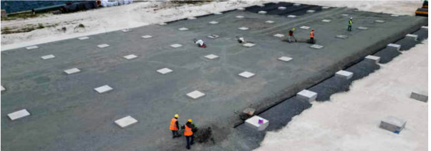
Photo 14 27/02/24 – Main process building area, spun pile installation completed, pile cap concrete works completed, excavation completed, backfilling and compaction works on going in preparation for lean concrete.
