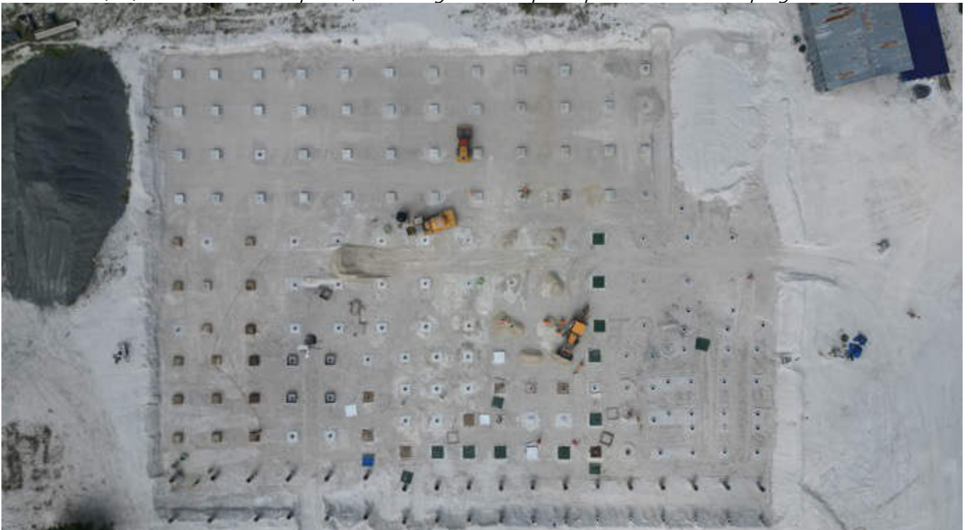
Photo 48 17/01/24 – Main process building area top view, backfilling work and pile cap concrete works in progress.
