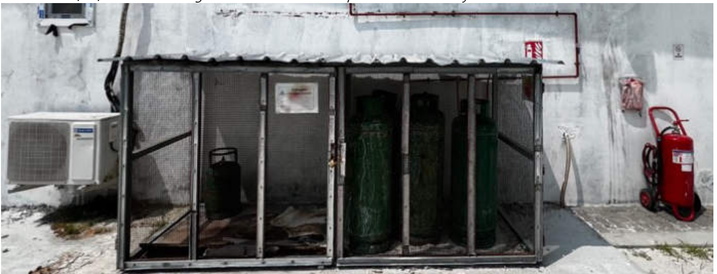
Photo 25 15/01/24 – Cooking gas storage area near the kitchen, the piping system has been re-routed and painted with valves made more accessible.
