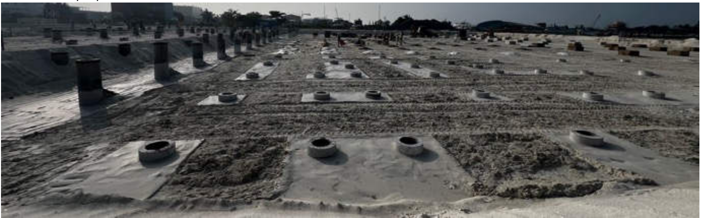
Photo 14 15/01/24 – Main process area, made ready for lean concrete of pile caps where the pile cutting has been completed.
