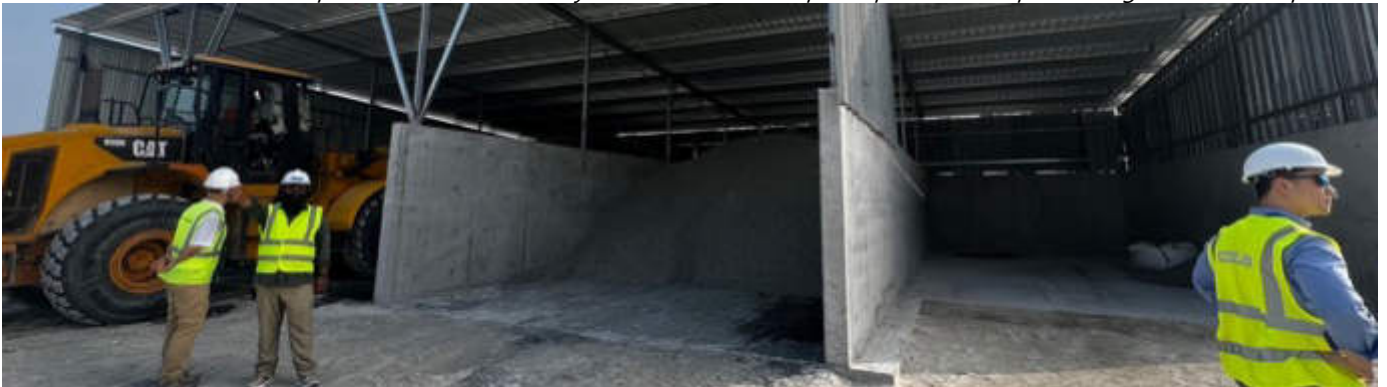
Photo 15 15/01/24 – Concrete batching plant material storage area, kept covered from wind and rain.
