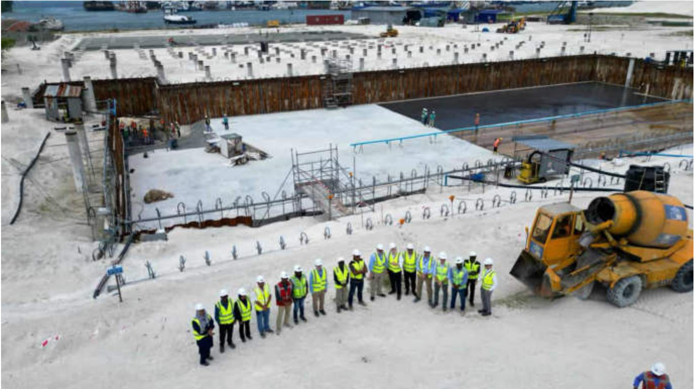
Photo 19 27/02/24 – DAB team members on site with the team members from DBO, EPC, PMU, PMDSC during the site walk about, showing the main ongoing construction area in the background.
