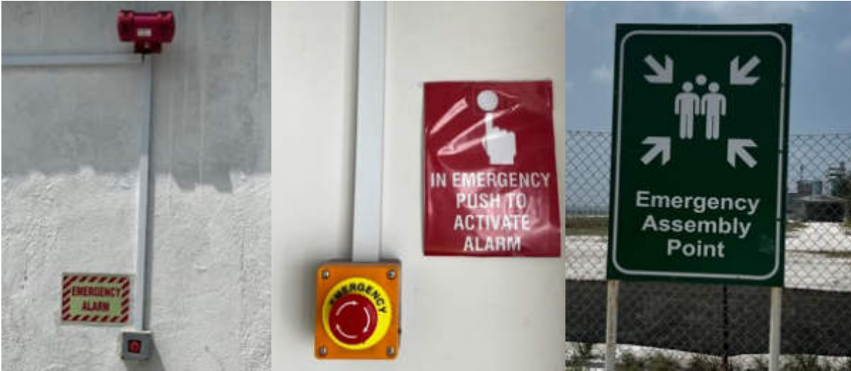
Photo 21 15/01/24 – Emergency alarm placed around the construction camp and clear assembly points established.
