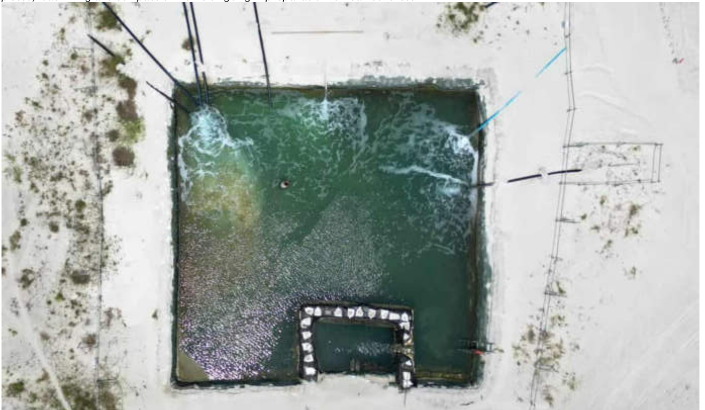
Photo 22 27/02/24 – Dewatering sedimentation pit, continuous dewatering will continue until bunker area concrete works have been completed. Water quality tests are done on a monthly basis to ensure that the environmental safeguards are complied.
