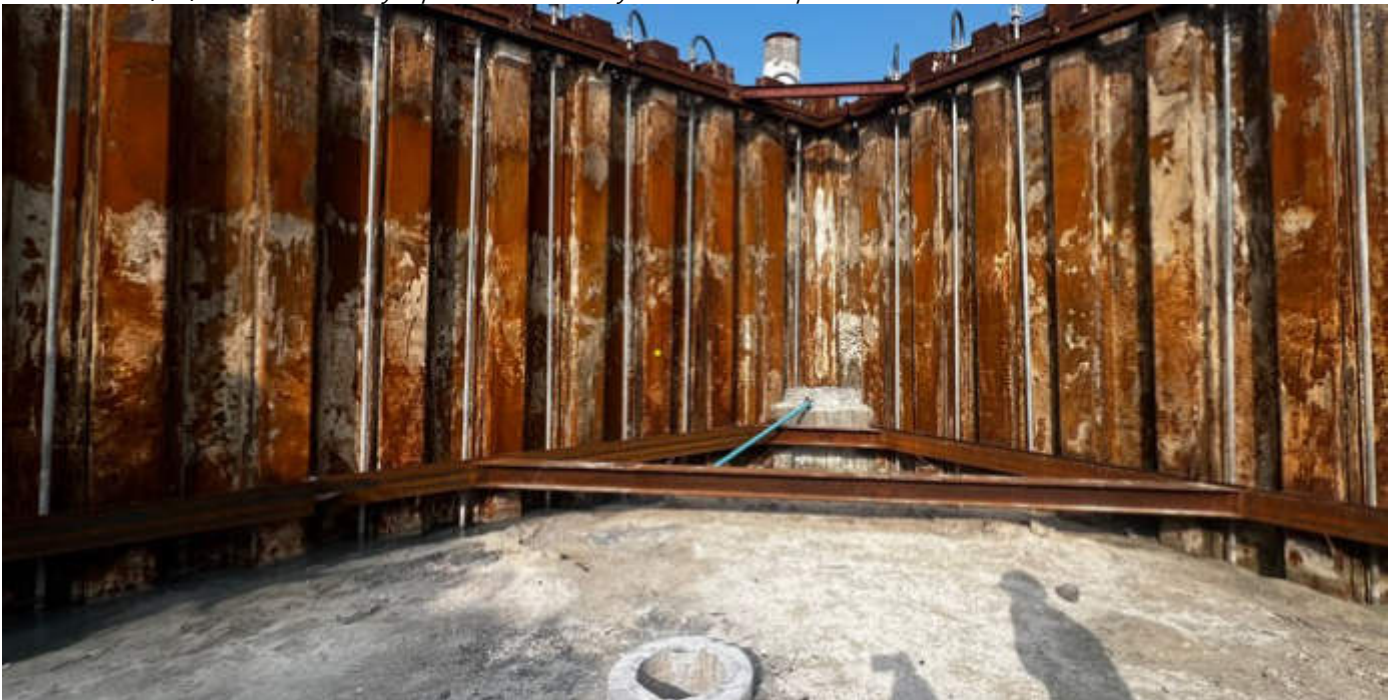
Photo 12 15/01/24 – Leachate pit in the bunker area, needs further excavation work in this area.
