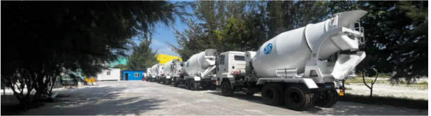
Photo 11 06/03/24 – Concrete mixer vehicles have been delivered to site, but registration process is yet to be completed.
