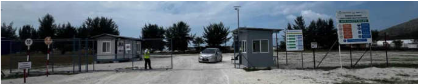
Photo 18 27/03/24 – Main entrance gate to work site, security guard posts in place and manned, CCTV is operational, Signboards are placed around the gate and construction site safety instructions are in place, including vehicle speed limits etc.
