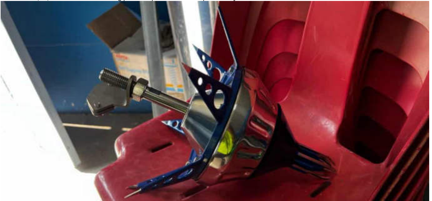
Photo 13 06/03/24 – Lightning conductor is on site and is to be installed on top of the batching plant silos.
