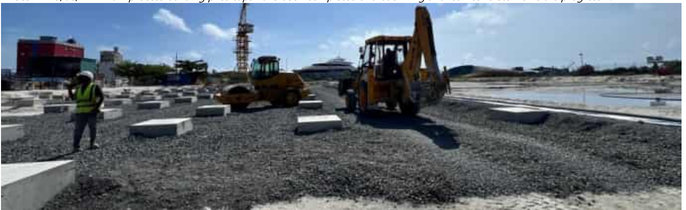
Photo 13 13/06/24 – Main process building piles caps have been completed and backfilling and lean concrete works are progressin.
