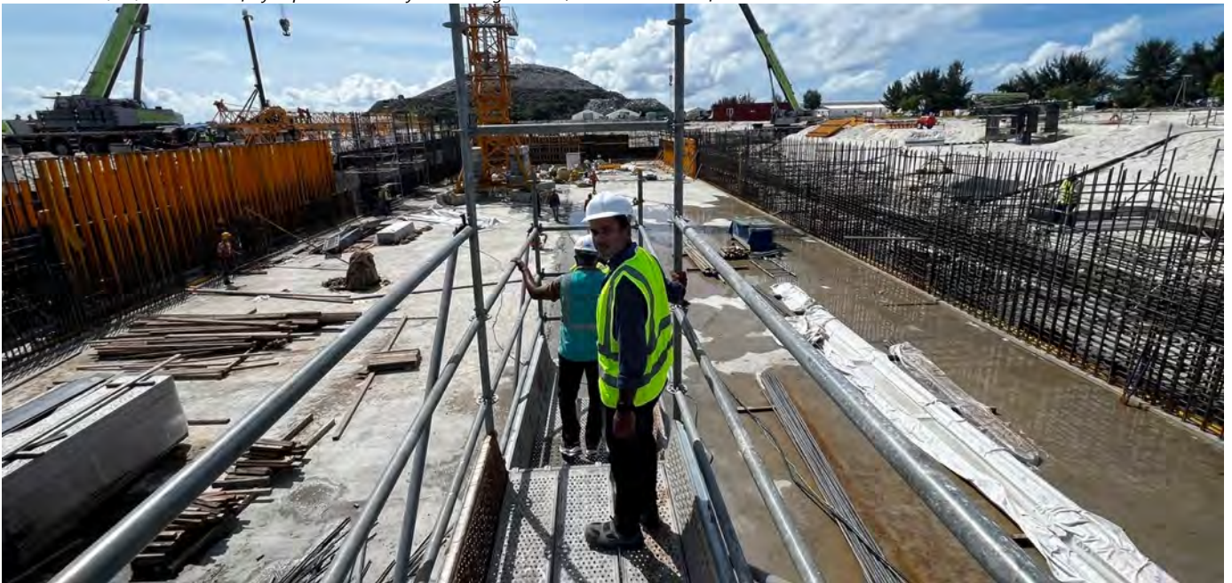
Photo 02 02/05/24 – Mr. Latheef from MOE visiting the site, inspecting the bunker area construction works.
