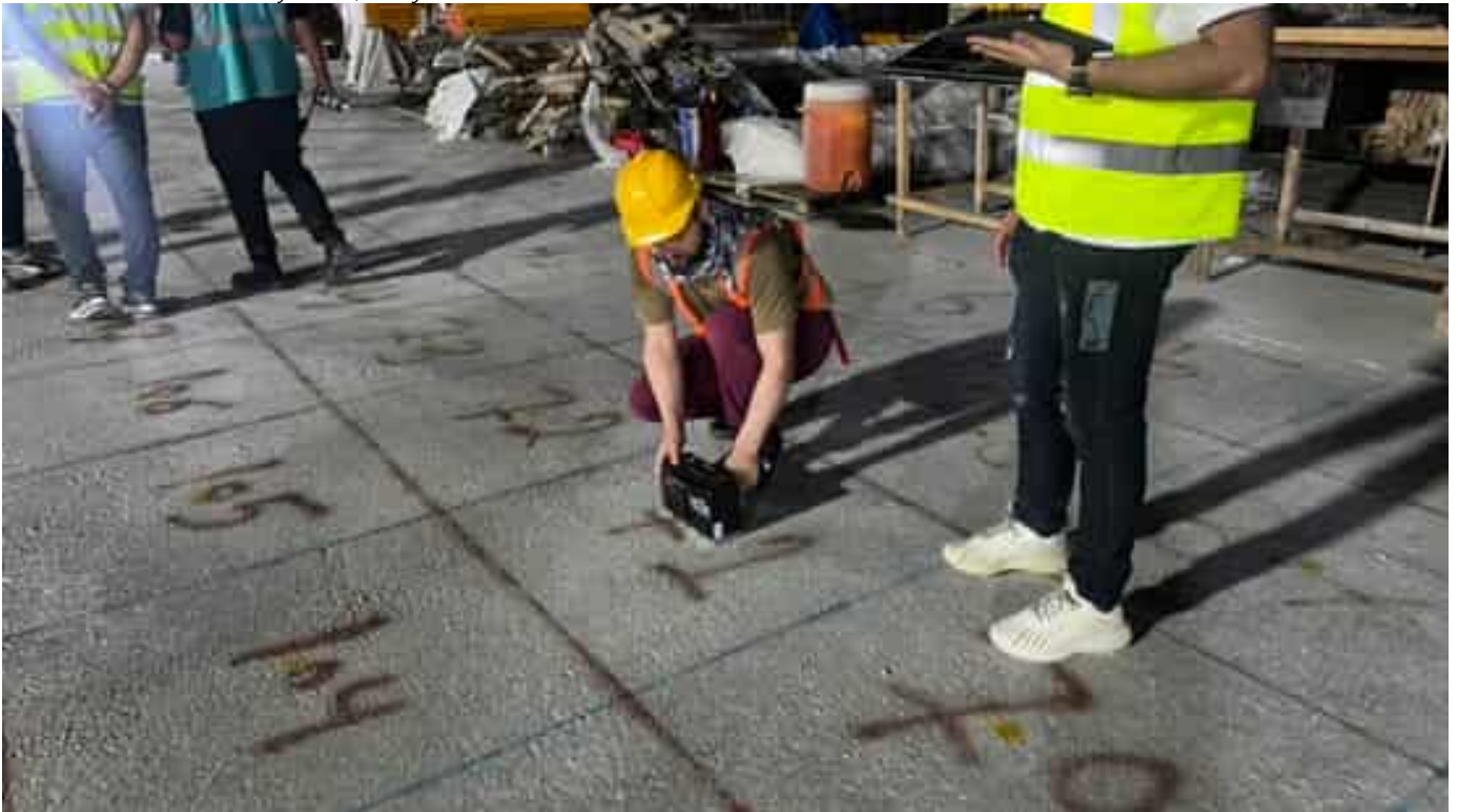
Photo 06 08/04/24 – Non destructive Pulse Echo Ultrasonic test being done on the Bunker slab in Area 1, by third party inspector Falcon Laboratories to check for any cracks, cold joints within the concrete slab.
