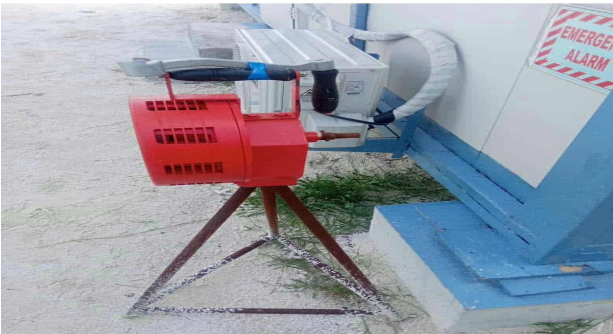
Manual alarm with rusty rod to be used to rotate
