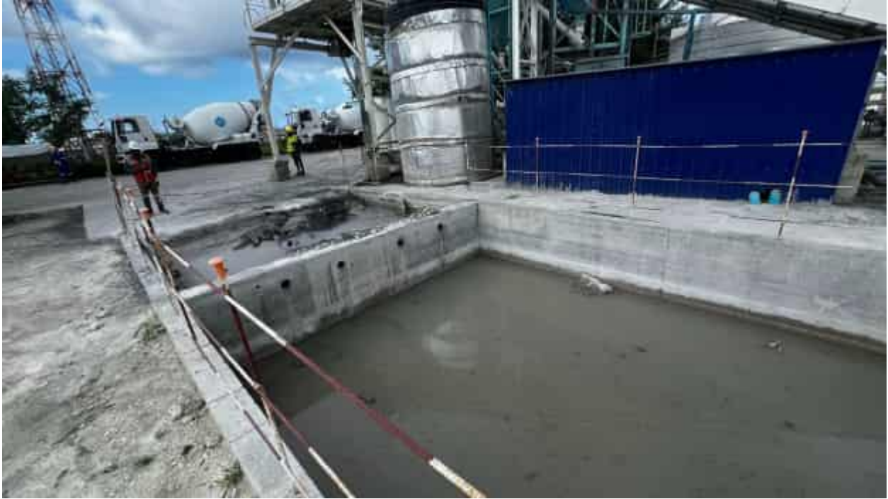
Sedimentation tank to take care of washing effluent in batching plant area
