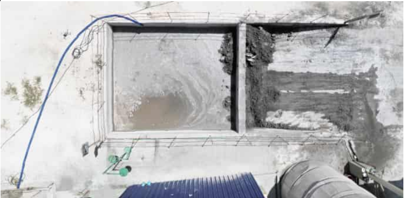
Photo 41 13/06/24 – Concrete truck wash area and waste water evaporation tank used by the batching plant.
