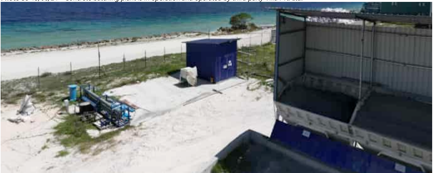
Photo 40 13/06/24 – Genset shed for the batching plant diesel generator and works in progress to install the desalination plant for the batching plant.
