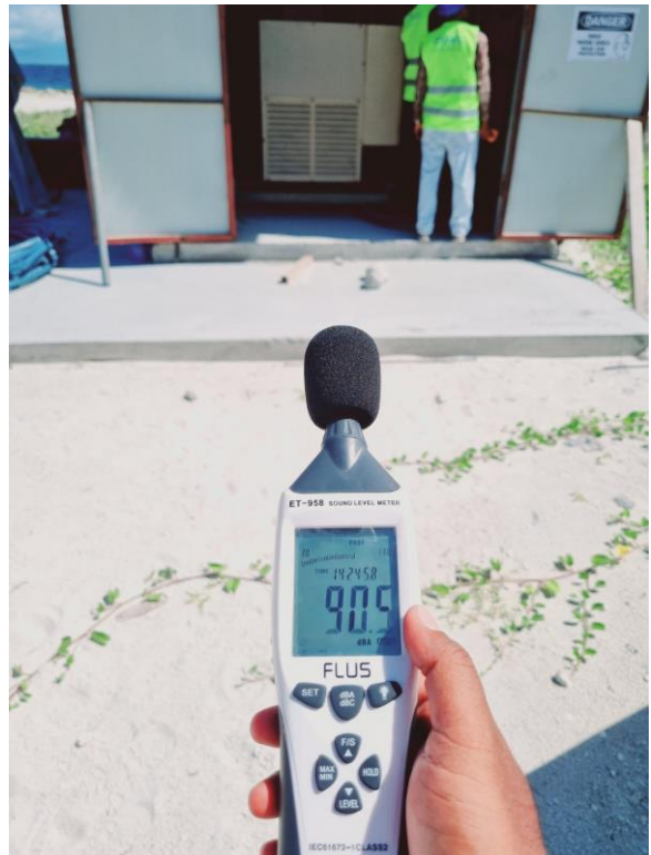
Batching Plant Generator
