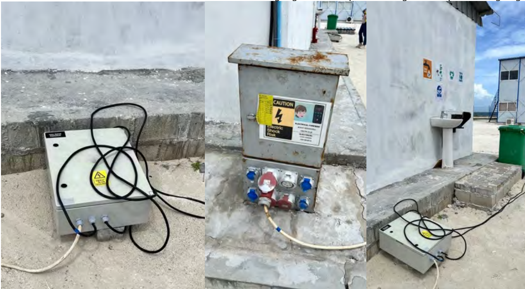
Photo 14 30/05/24 – Adequate measures to be taken for electrical equipment in the camp site..
