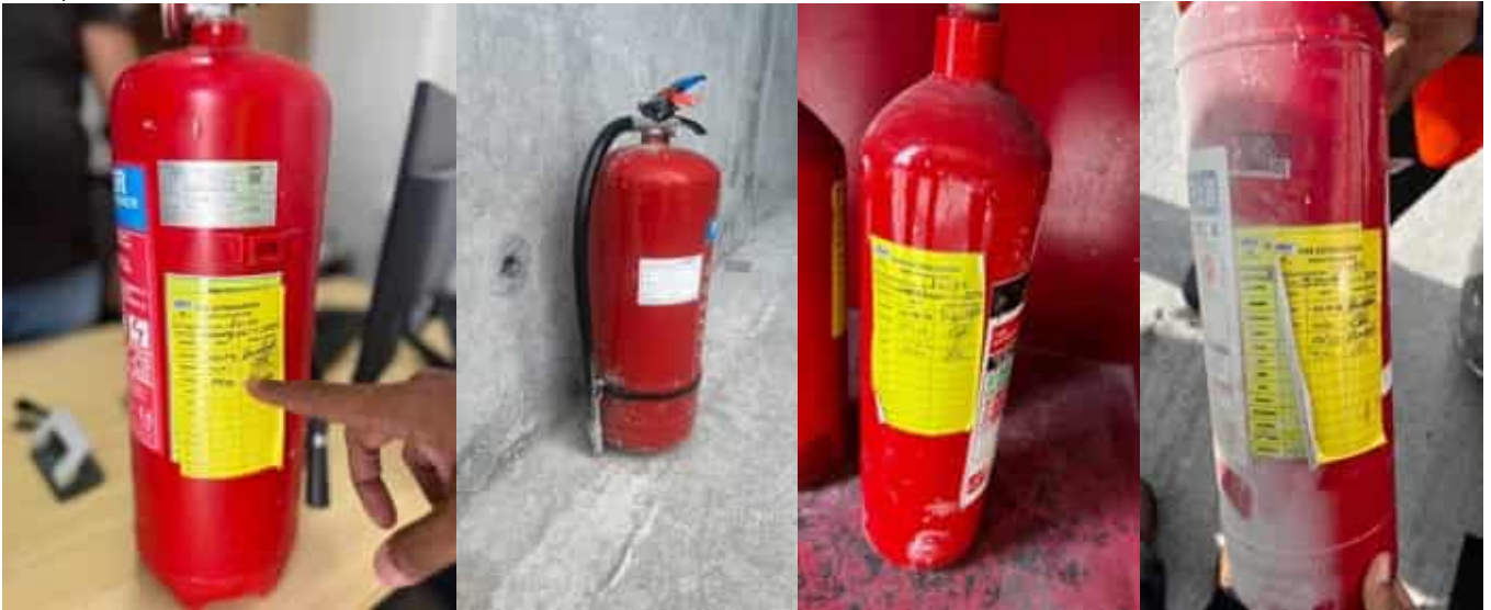
Photo 05 14/04/24 – Expired third party certification, HSE inspections done after and it was not reported/identified.
