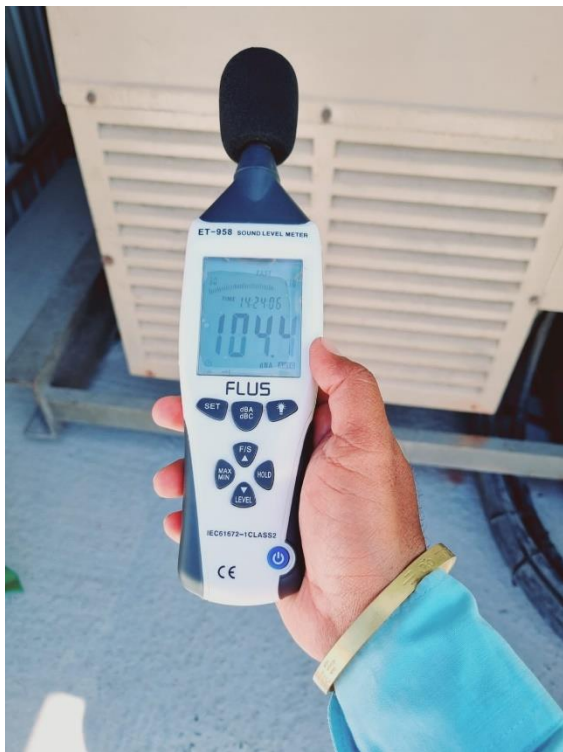
Batching Plant Generator
