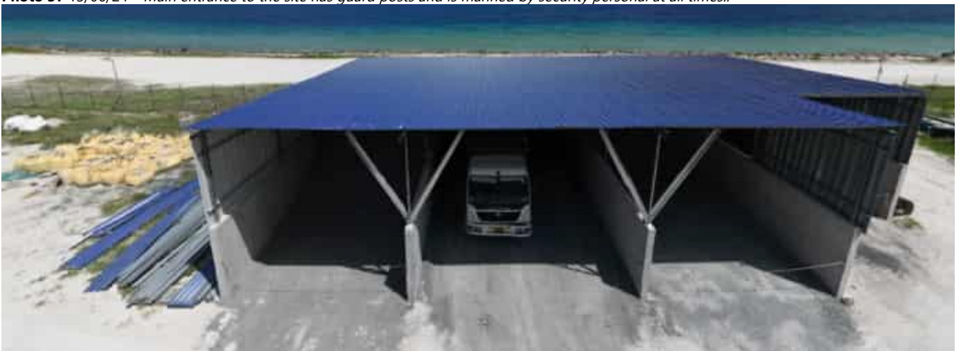
Photo 38 13/06/24 – Material storage area at the concrete batching plant area for aggregates and admixtures.
