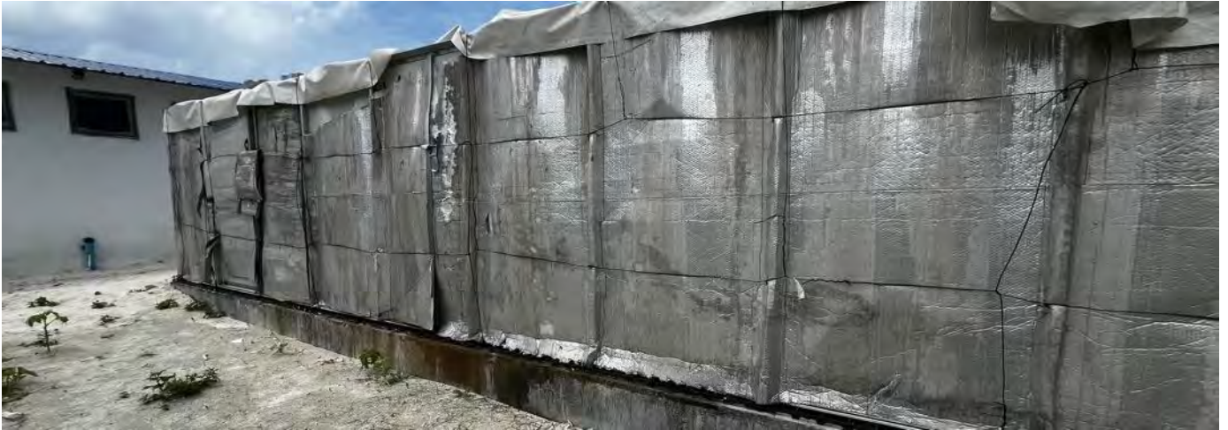
Photo 28 09/05/24 – Emergency water tank on site, has some leaks and this has been raised in several reports, but action taken to rectify..
