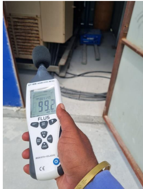
Batching Plant Generator
