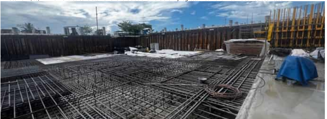
Photo 19 27/03/24 – Bunker area concrete works for the slab and walls are in progress. Area 2 and Area 3 reinforcement is being prepared.
