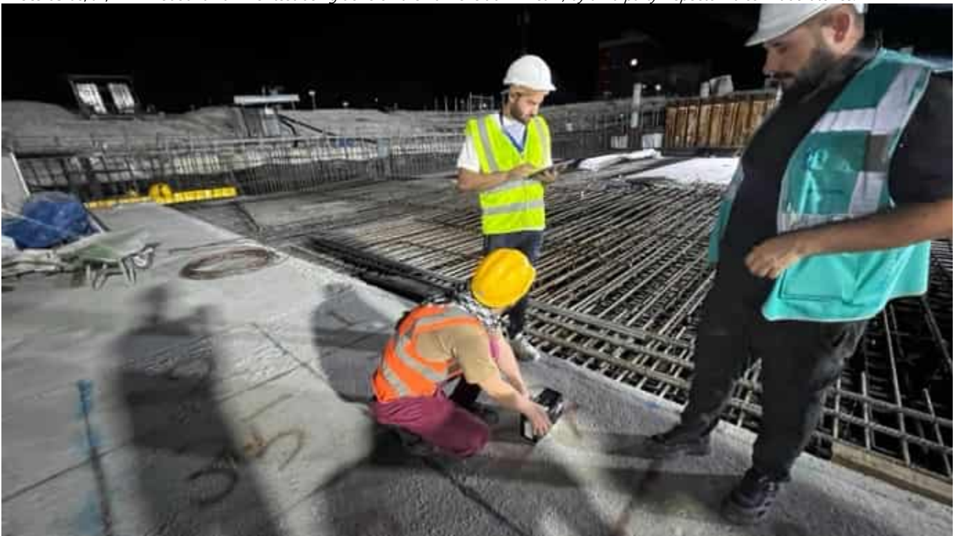
Photo 04 08/04/24 – Non destructive Pulse Echo Ultrasonic test being done on the Bunker slab in Area 1, by third party inspector Falcon Laboratories to check for any cracks, cold joints within the concrete slab.
