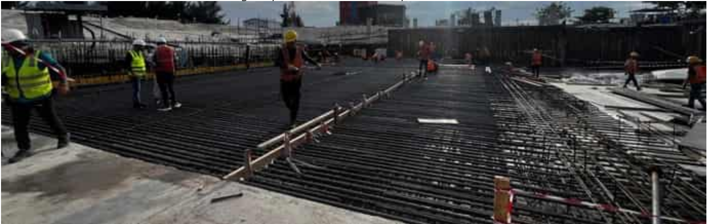
Photo 31 14/04/24 – Reinforcement installation work is ongoing in the Bunker Slab Area 2, and Area 3.
