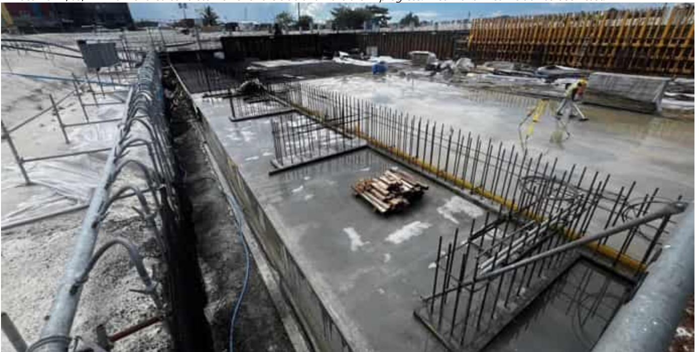
Photo 17 27/03/24 – Bunker area concrete works for the slab and walls are in progress. Area 1 and Area 4 slab has been cast.
