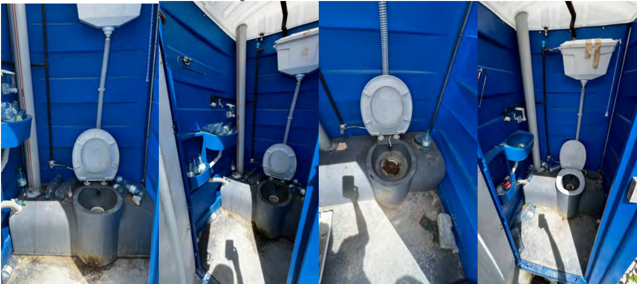
Photo 13 02/05/24 – The portable toilets were not cleaned and in bad condition, EPC HS team has been informed of the issue.
