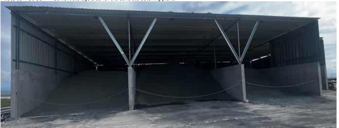
Photo 10 14/04/24 – Sheltered storage area for aggregates and concrete admixture chemicals used by the concrete batching plant.
