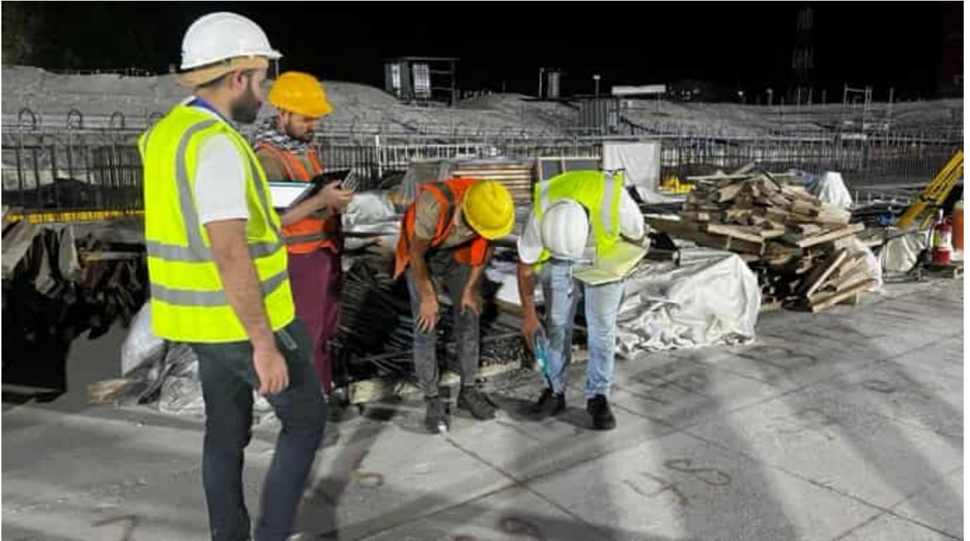
Photo 03 08/04/24 – Rebound hammer test being done on the Bunker slab in Area 1, by third party inspector Falcon Laboratories.
