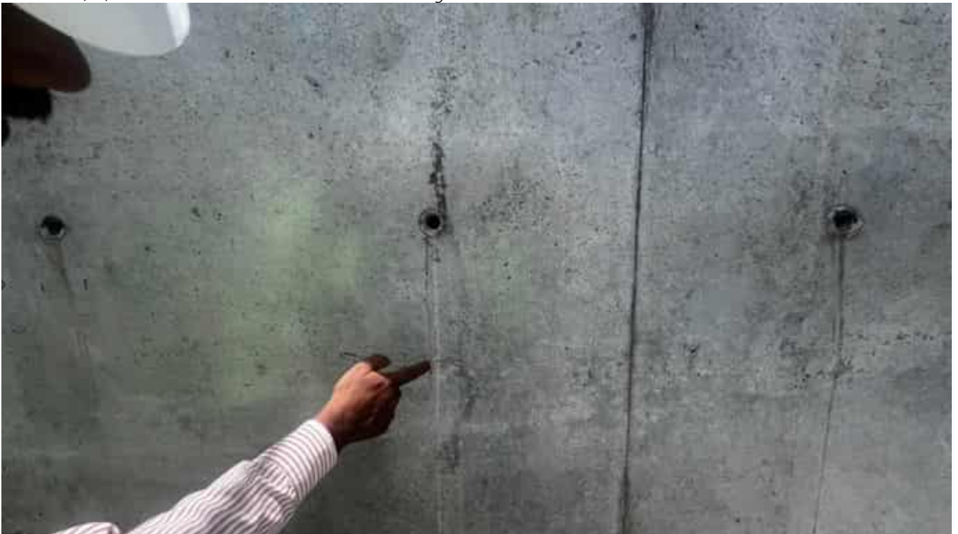
Photo 03 14/04/24 – Several cracks were observed on the Bunker Wall B that has been cast and further investigation has been requested from the contractor. The Echo Pulse Ultrasonic tests were conducted on this part of the wall and the extent of the cracks will be checked once the reports are submitted.
