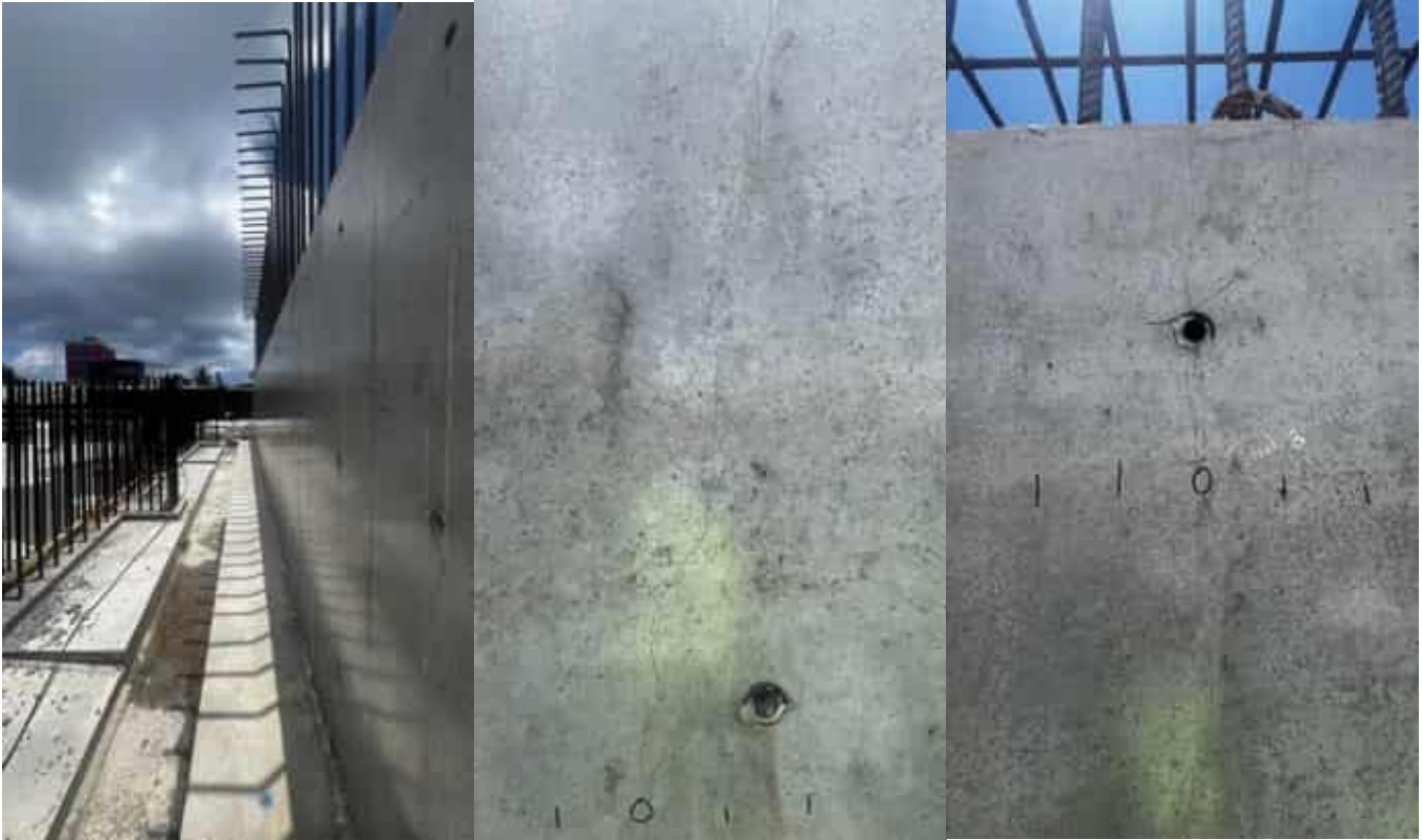
Photo 04 14/04/24 – The Echo Pulse Ultrasonic tests were conducted on this part of the wall and the extent of the cracks will be checked once the reports are submitted.
