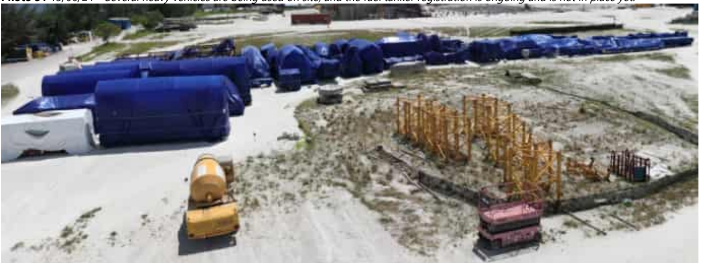
Photo 32 13/06/24 – Parts of the tower crane and the grate is stored on the laydown area.
