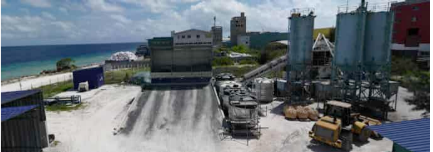
Photo 39 13/06/24 – Concrete batching plant is in operation and operated by third party Villa Pvt. Ltd.
