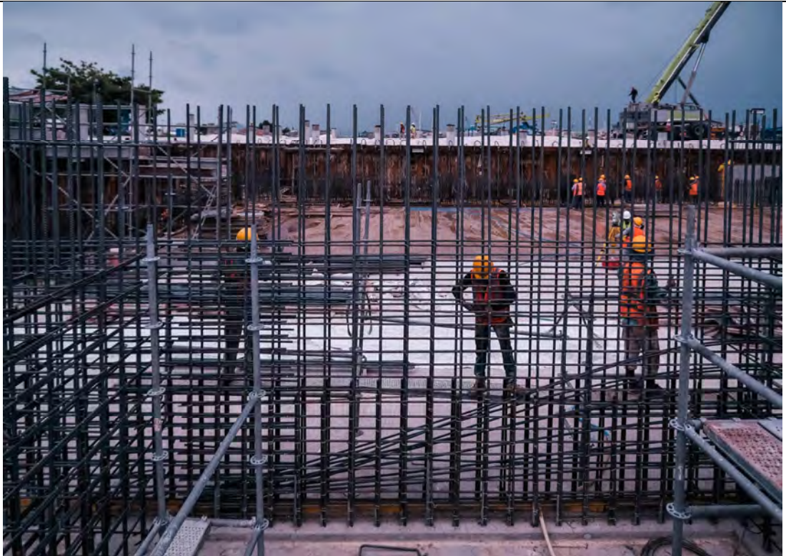
BUNKER - REINFORCEMENT BAR AND FORMWORK IN PROGRESS FOR WALL H, A & J.
