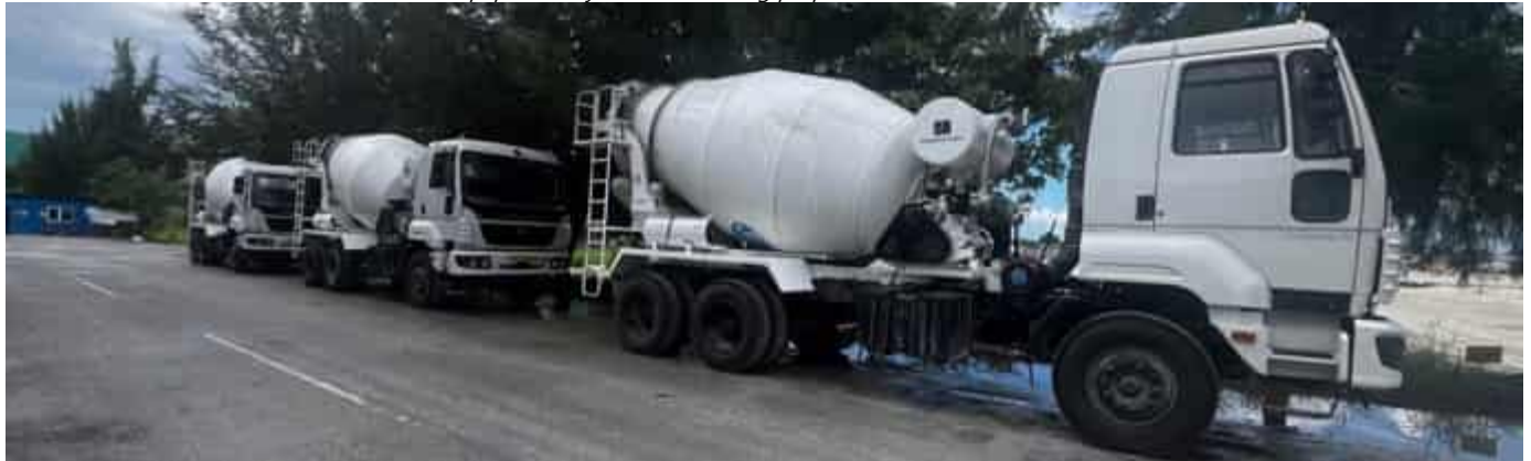
Photo 03 04/04/24 – Concrete mixing trucks on site, however vehicle registration is not in place yet.
