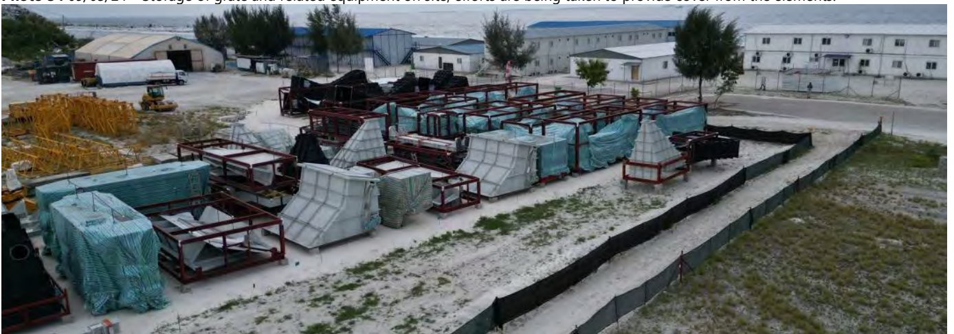
Photo 35 09/05/24 – Storage of grate and related equipment on site, efforts are being taken to provide cover from the elements.
