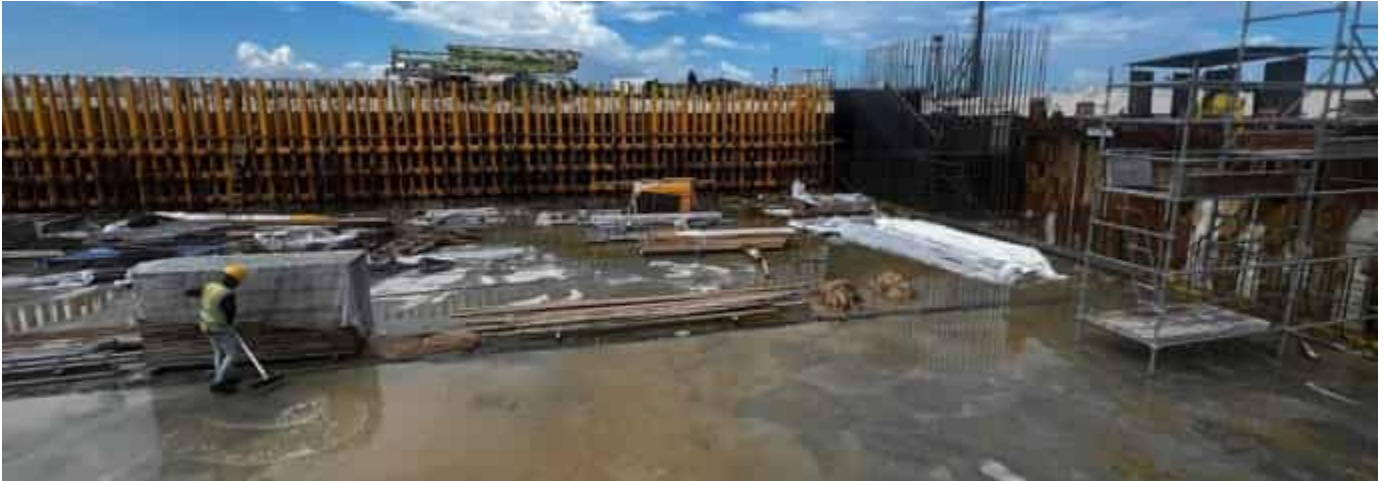
Photo 18 27/03/24 – Bunker area concrete works for the slab and walls are in progress. Area 1 and Area 4 slab has been cast.
