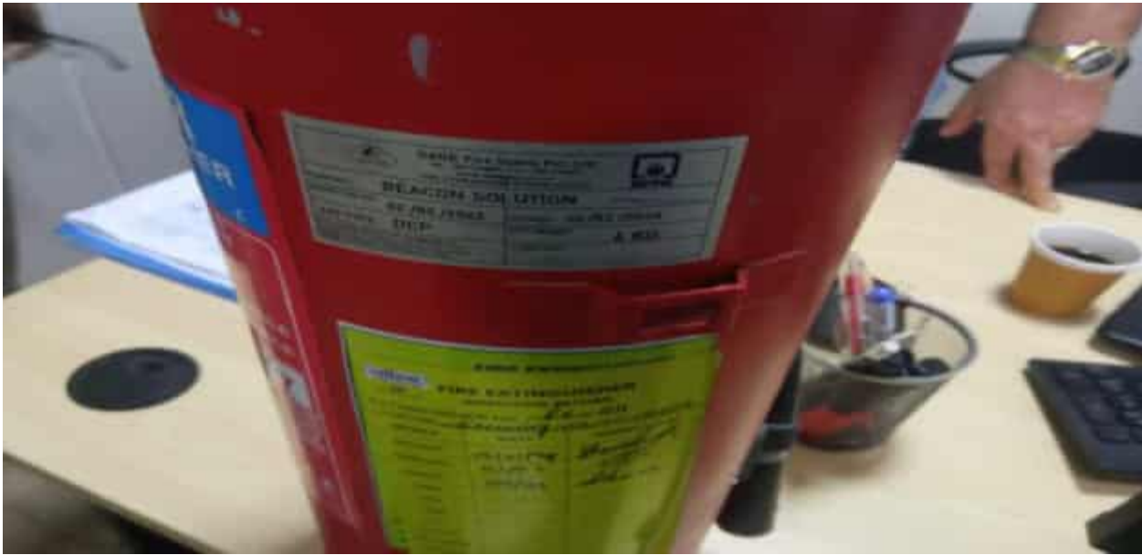
Fire extinguisher without fitness by third party
