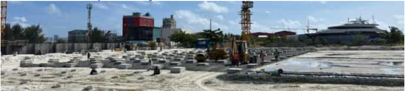
Photo 20 13/06/24 – Main process building area showing part of the lean concrete completed over the backfilled material.
