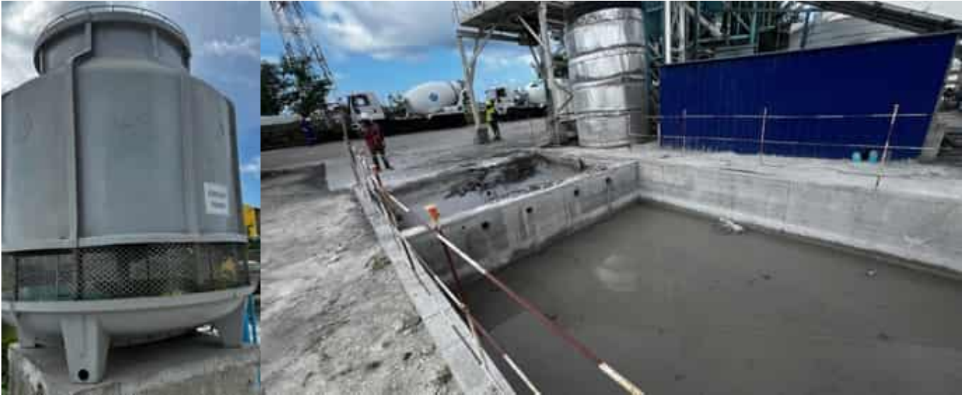
Photo 15 14/04/24 – Water cooling tower used at the batching plant, and the vehicles wash area and sedimentation tank for waste concrete.
