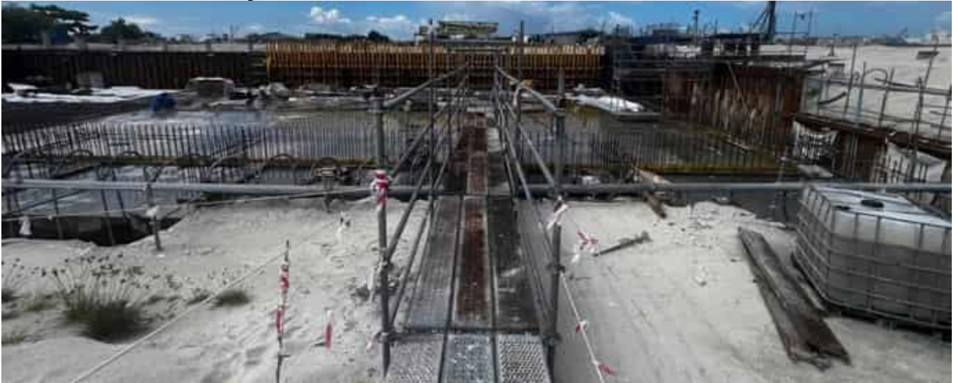
Photo 16 27/03/24 – Bunker area concrete works for the slab and walls are in progress. Area 1 and Area 4 slab has been cast.
