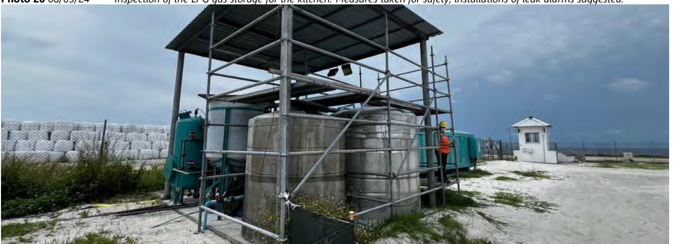
Photo 21 08/05/24 – WTP is operational and being used, monthly outfall tests are done to ensure environmental limits are achieved.
