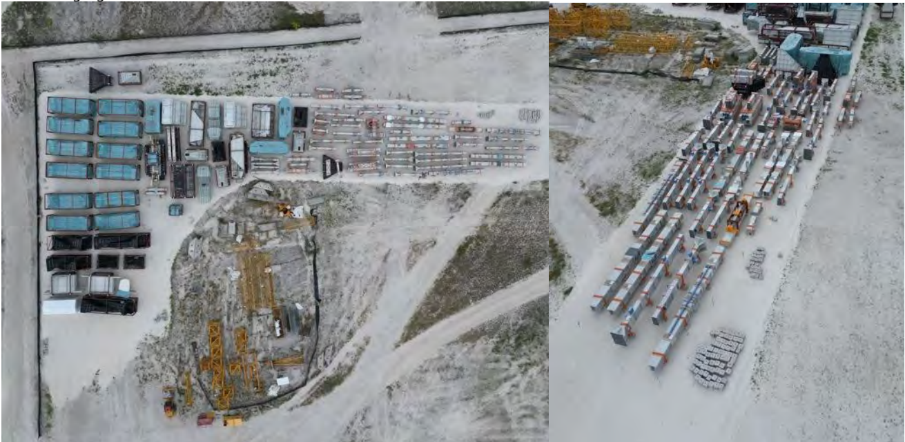
Photo 34 09/05/24 – Storage of grate and related equipment on site, efforts are being taken to provide cover from the elements.
