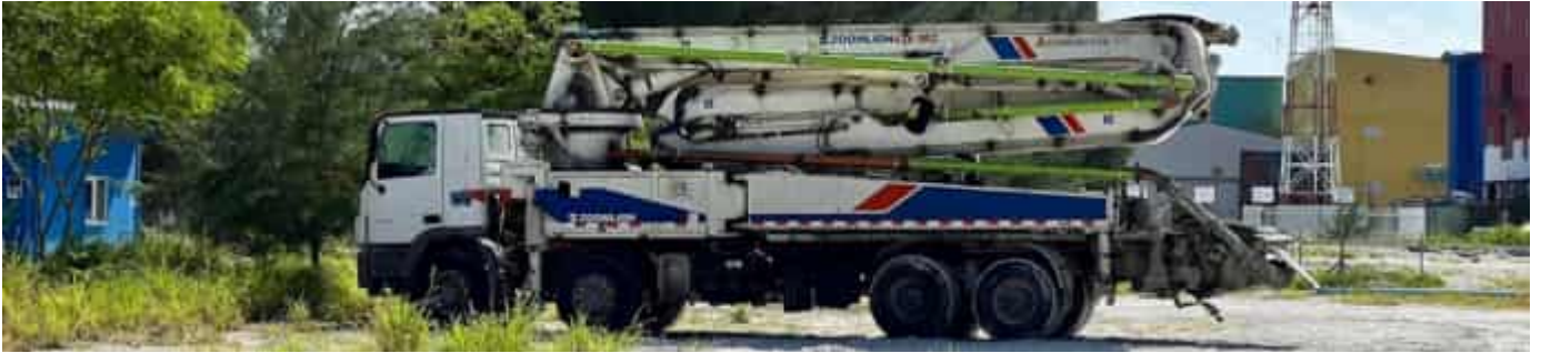
Photo 23 13/06/24 – Concrete pump used by EPC for the concreting works at the bunker area.
