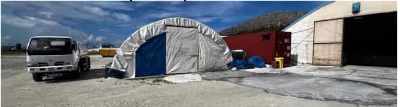
Photo 29 27/03/24 – Storage tents for materials and equipments in place. Fuel tanker is on site.
