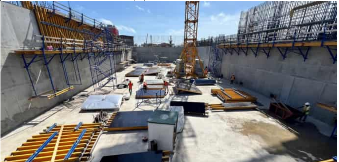
Photo 10 13/06/24 – Bunker construction is ongoing and bunker wall concrete works is progressing as expected.
