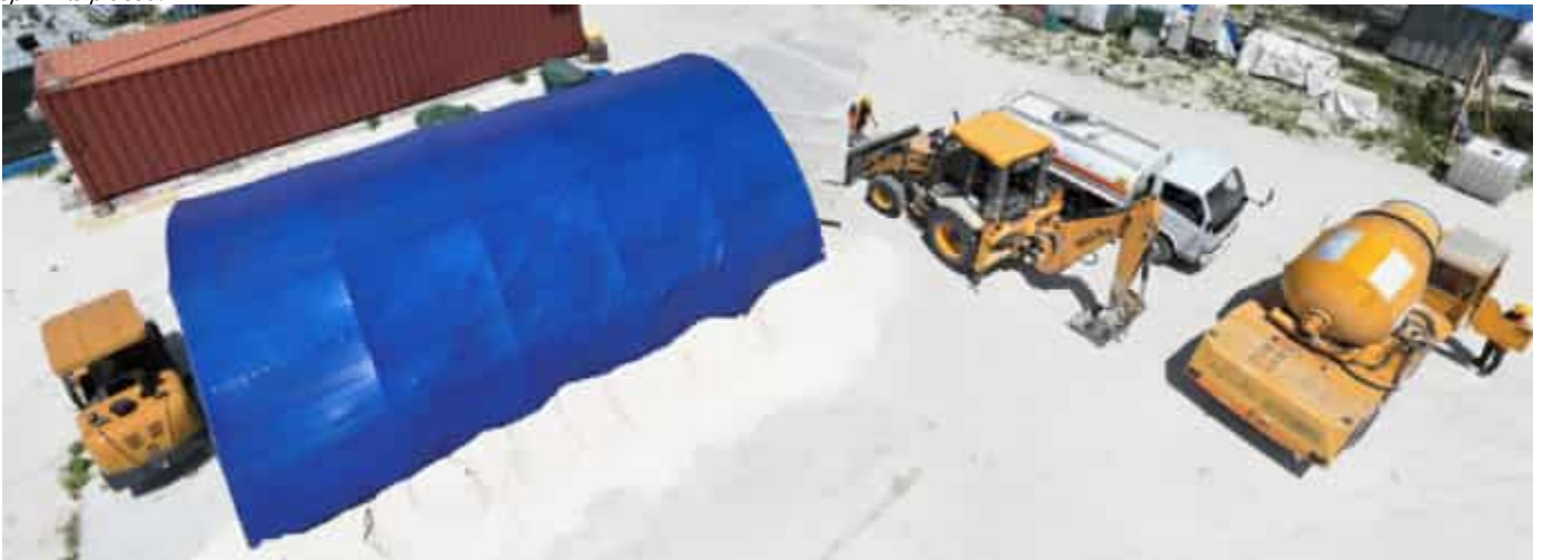
Photo 31 13/06/24 – Several heavy vehicles are being used on site, and the fuel tanker registration is ongoing and is not in place yet.
