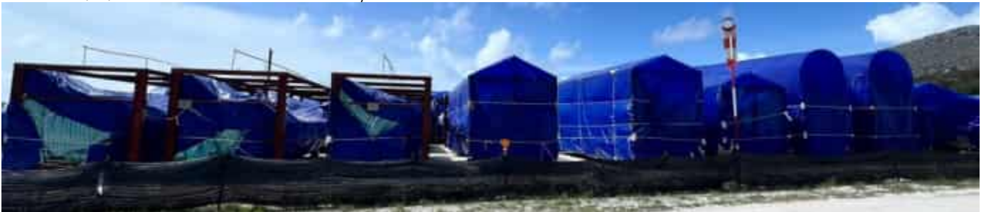
Photo 03 13/06/24 – CNTY delivered the grate parts and are stored on the site laydown area and covered with several sheets of canvas to protect from the elements.
