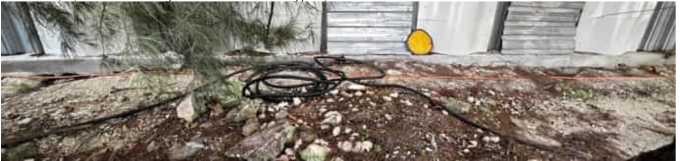
Photo 16 14/04/24 – Redundant loose electrical cable found close to the batching plant area, should be removed.
