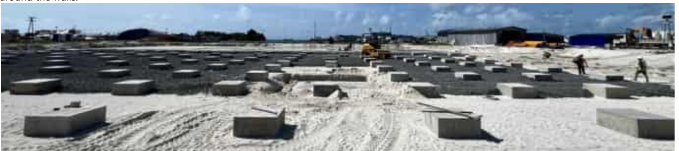
Photo 12 13/06/24 – Main process building piles caps have been completed and backfilling and lean concrete works are progressin.
