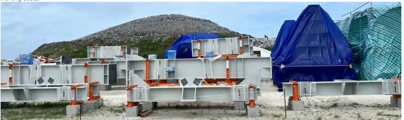
Photo 18 30/05/24 – Equipment delivered to site being covered with canvas material to protect against the elements.
