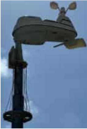
Photo 08 13/06/24 –Weather station is in working condition and real time information is recorded by the EPC HSE team 24/7.
