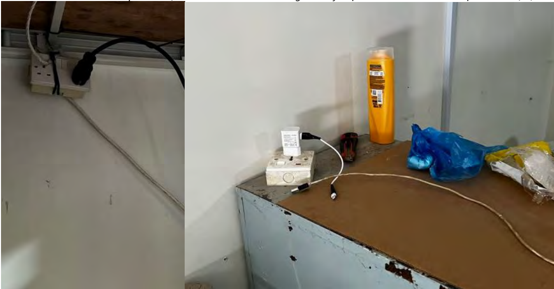
Photo 26 09/05/24 – Inspection of workers accommodation, unsafe use of electrical extension boards was highlighted and mitigation measures were advised.
