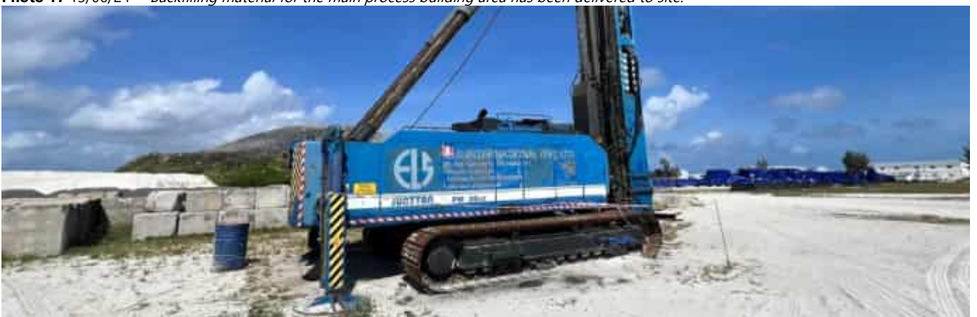
Photo 18 13/06/24 – The pile driving machine from ELS is still parked on site, together with the concrete blocks.
