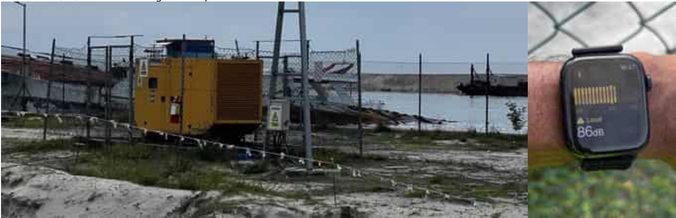
Photo 29 14/04/24 – Genset deemed to be loud and close to the workers area, maintenance check requested.
