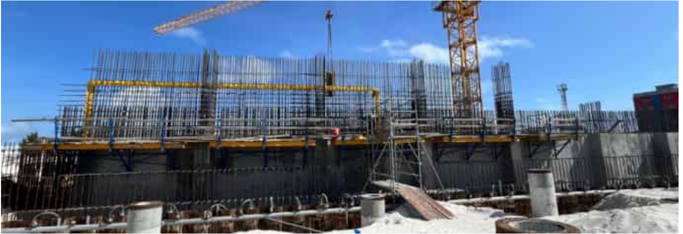
Photo 11 13/06/24 – Continuous dewatering is ongoing and will continue until the bunker walls are completed and backfilling is completed around the walls.
