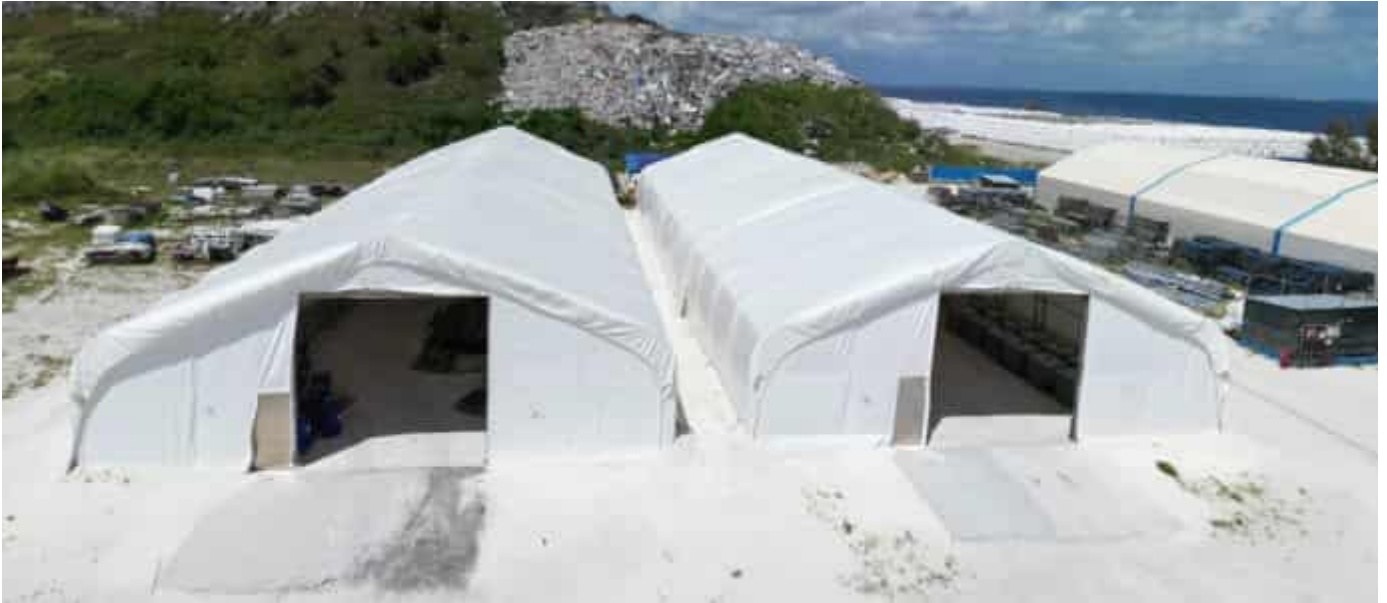
Photo 30 13/06/24 – Storage tents used for concrete admixture chemical storage. Requires measures to be in place for accidental spillage and no spill kits placed.
