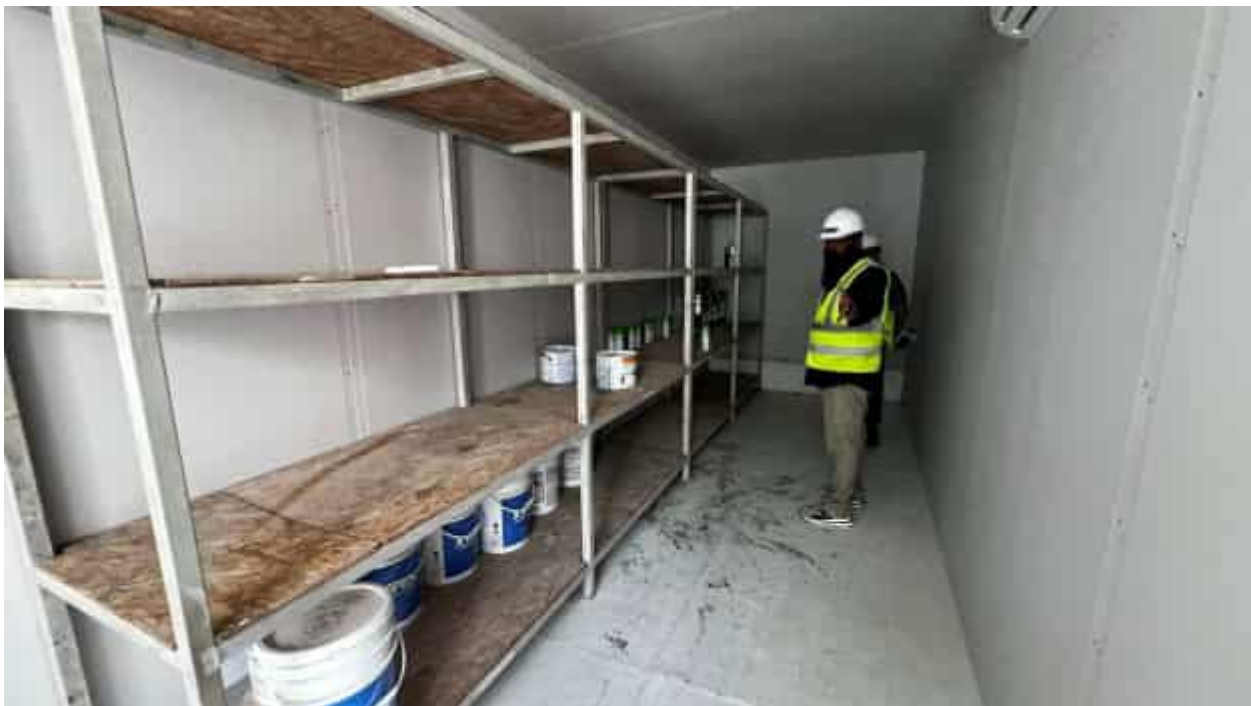
Hazardous chemical storage container from Inside
