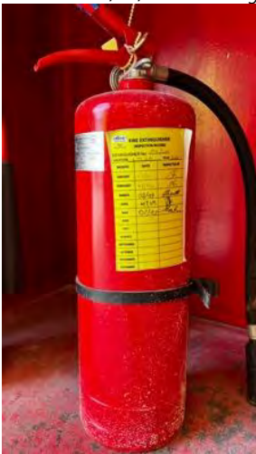
Photo 29 09/05/24 – The fire extinguishers placed around the site has been inspected by site HS team, however several were found with expired third-party inspection certificates.
