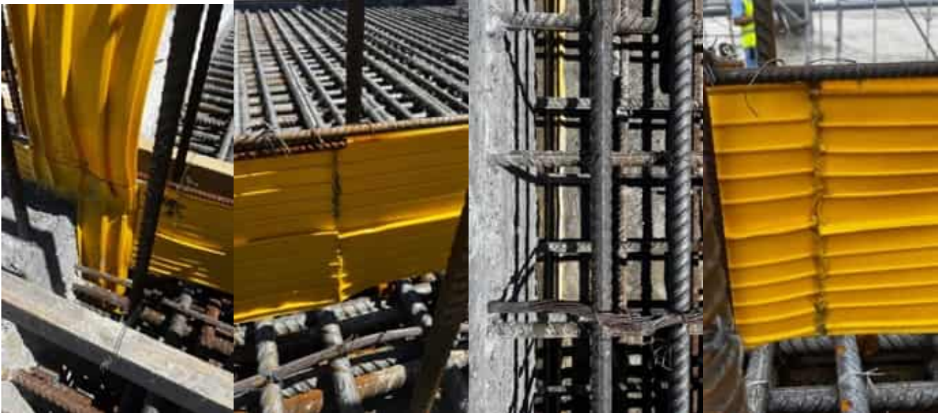
Photo 36 16/04/24 – Waterbars placed in the slab and wall connections and all joints are welded and inspected.
