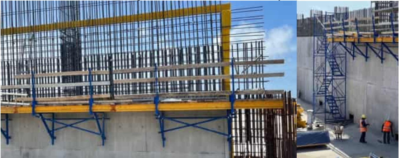
Photo 09 13/06/24 – Scaffolding designer and inspector assigned and mock ups made before being installed and used, and safety measures in place for evacuation from the bunker area in case of emergency.
