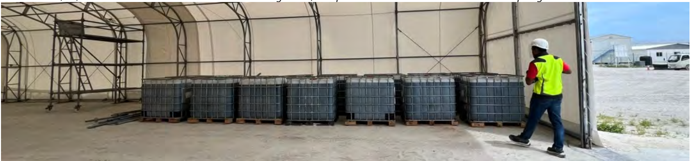
Photo 11 30/05/24 – Conplast X400 Construction chemicals onsite storage area, adequate measures to be taken to address spillage.
