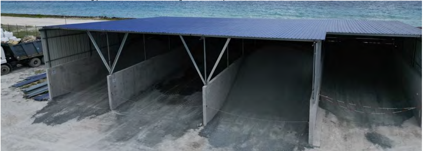
Photo 32 09/05/24 – Aggregates storage area for the batching plant, kept sheltered from the elements.
