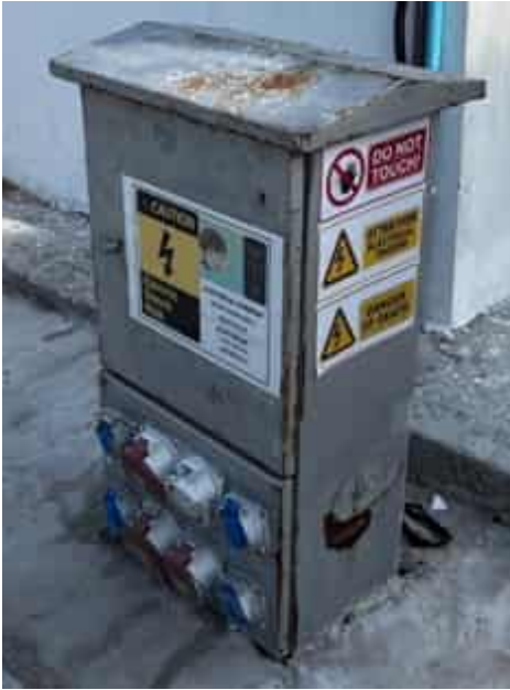
Photo 24 14/04/24 – Outdoor electrical panel with rain cover missing on the outlet, should be rectified immediately.
