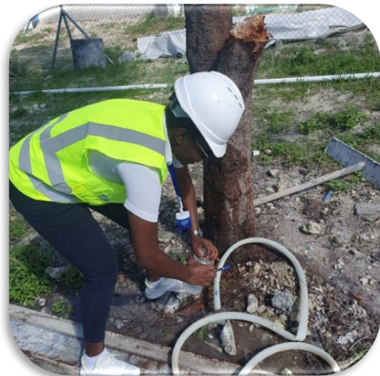
Supply Water for Camp And Construction Sampling
