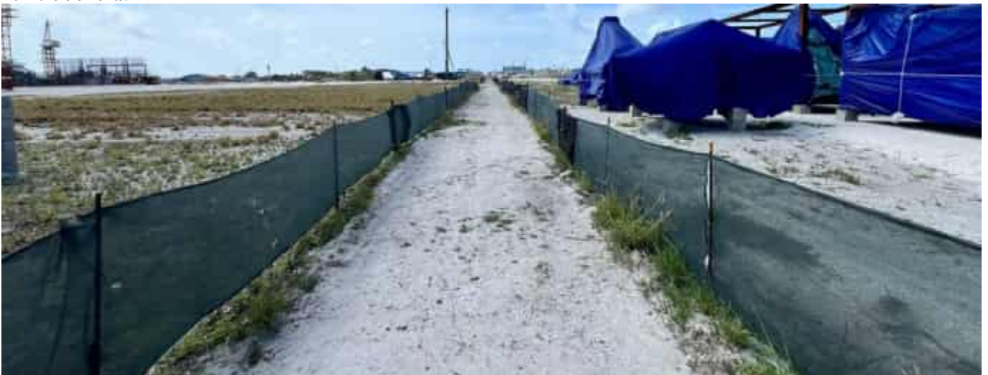
Photo 04 13/06/24 – The walkpath from the construction camp to the construction area is kept clean and free of tripping hazards.
