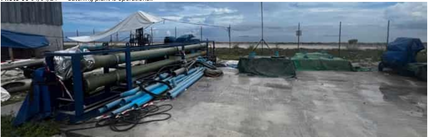
Photo 07 04/04/24 – Desalination plant works for the batching plant is in progress. Needs to check on permits for the bore hole and the plant.
