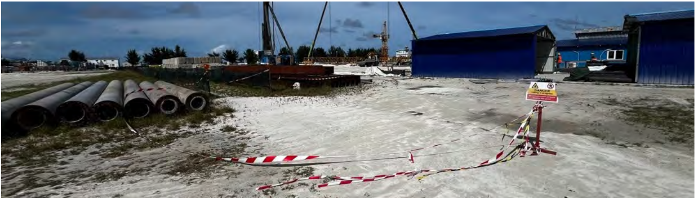
Photo 01 02/05/24 – The safety tape blown away due to high winds, needs to be rectified.
