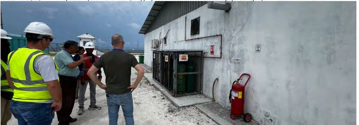
Photo 20 08/05/24 – Inspection of the LPG gas storage for the kitchen. Measures taken for safety; installations of leak alarms suggested.
