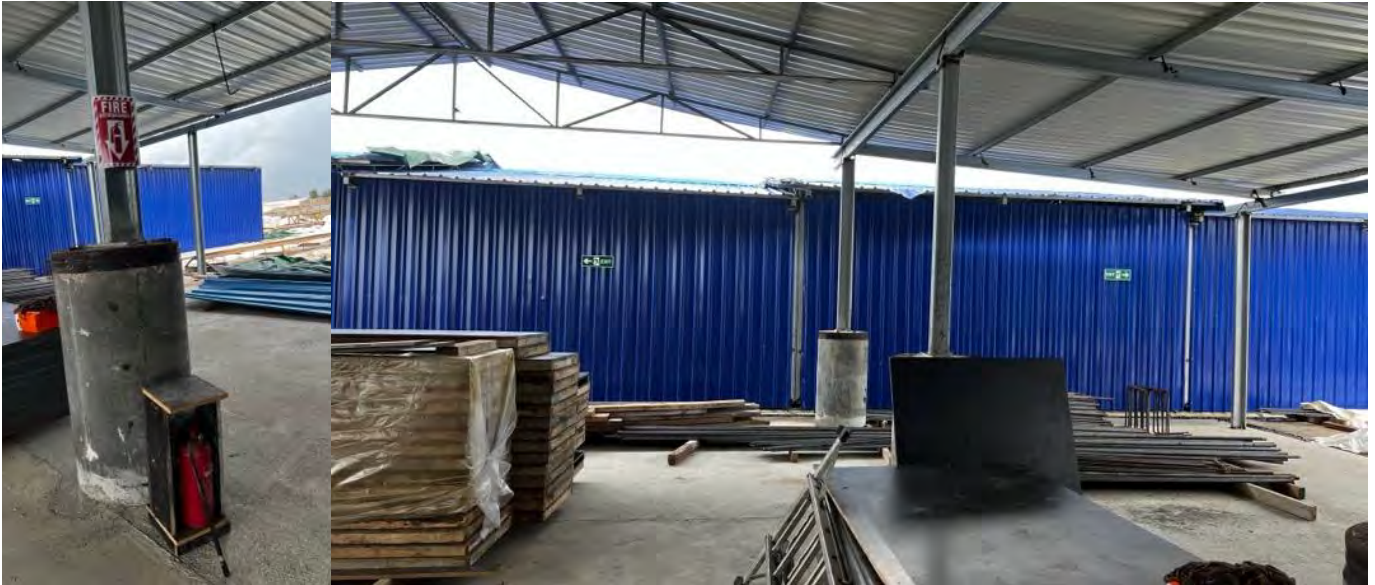
Photo 07 07/05/24 – Fire fighting equipment has been placed in the reinforcement workshop along with signage.
