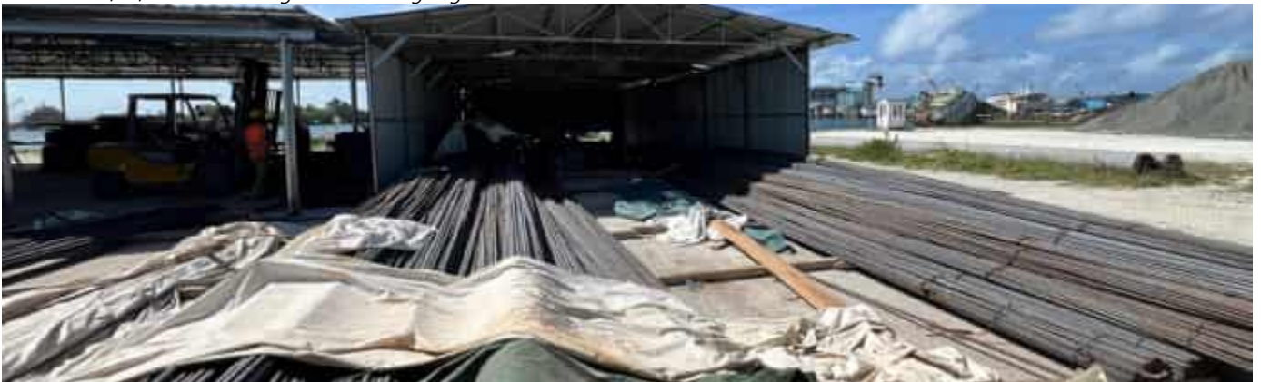
Photo 16 13/06/24 – Reinforcement for the bunker walls and part of the main process building foundation has been delivered to site.
