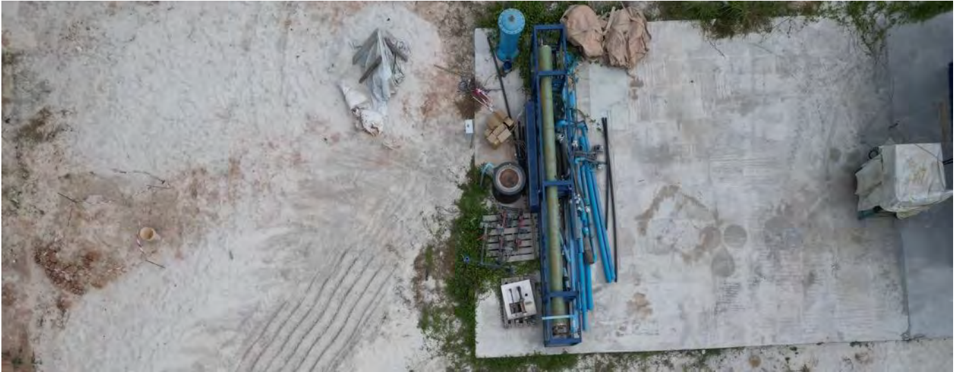
Photo 33 09/05/24 - Area allocated for desalination plant for the batching plant, requirement of permits from government authorities for bore hole was highlighted.
