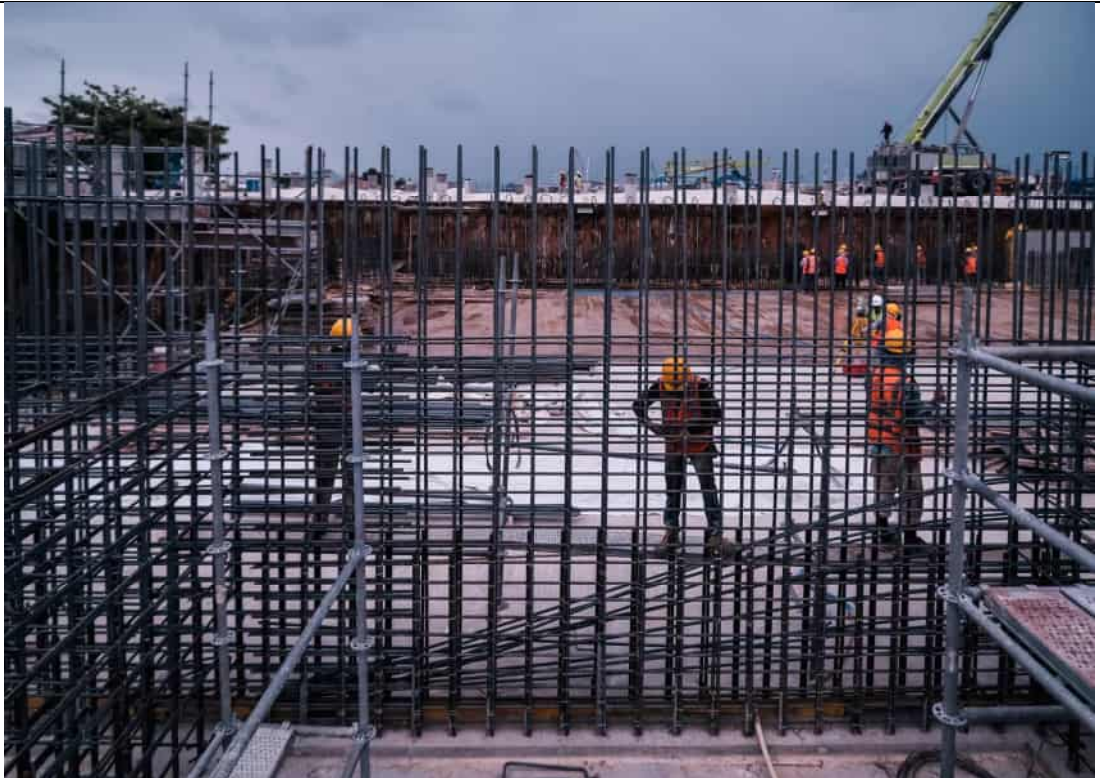
BUNKER - REINFORCEMENT BAR AND FORMWORK IN PROGRESS FOR WALL H, A & J.
