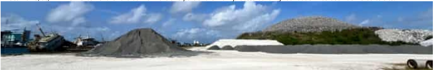
Photo 17 13/06/24 – Backfilling material for the main process building area has been delivered to site.
