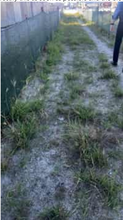
Photo 38 17/04/24 – The pedestrian walk path to the construction camp is overgrown with weeds, and is deemed as a tripping hazard. Needs to be cleared as soon as possible.
