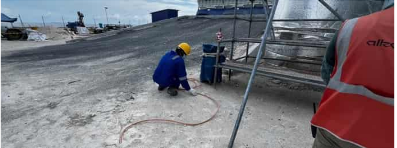
Photo 12 14/04/24 – Electrical cable identified as tripping hazard and asked to rectify.
