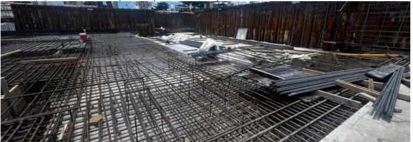
Photo 02 14/04/24 – Reinforcement installation work is continuing in Area 2 and Area 3 of the bunker slab.
