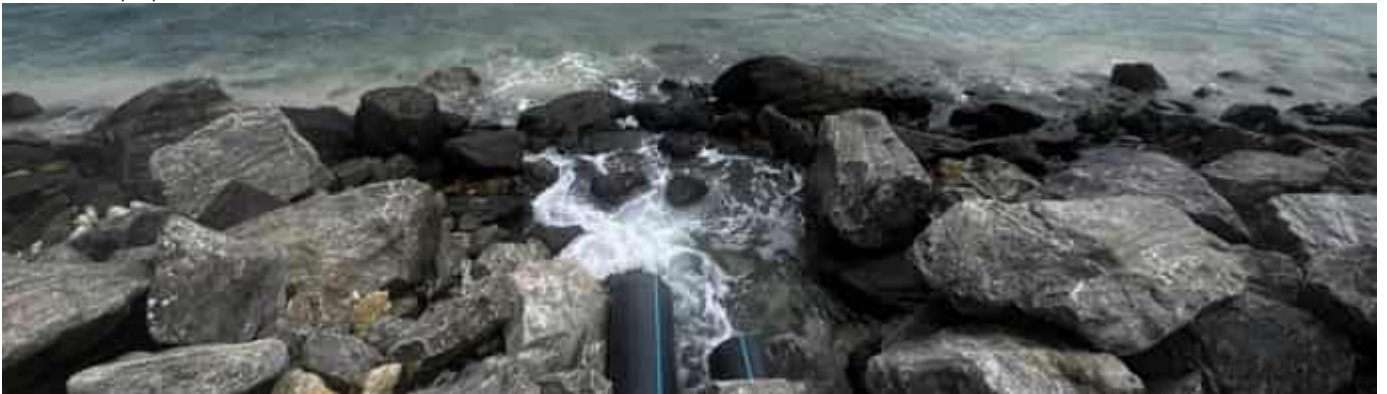
Photo 14 04/04/24 – Dewatering pipe outfall to sea, no sediments or discoloration seen. Monthly quality control checks in place.
