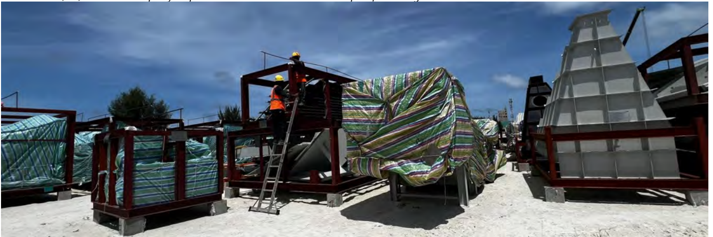
Photo 18 02/05/24 – Equipment delivered to site being covered with canvas material to protect against the elements.
