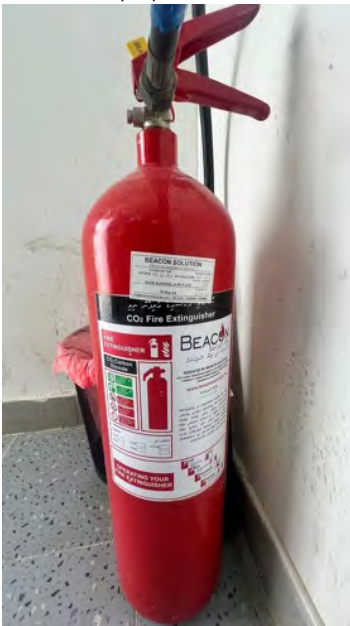
Photo 17 30/05/24 – Third party inspection has expired on many of the fire extinguishers on site, however EPC HS team inspections are done on a monthly basis..
