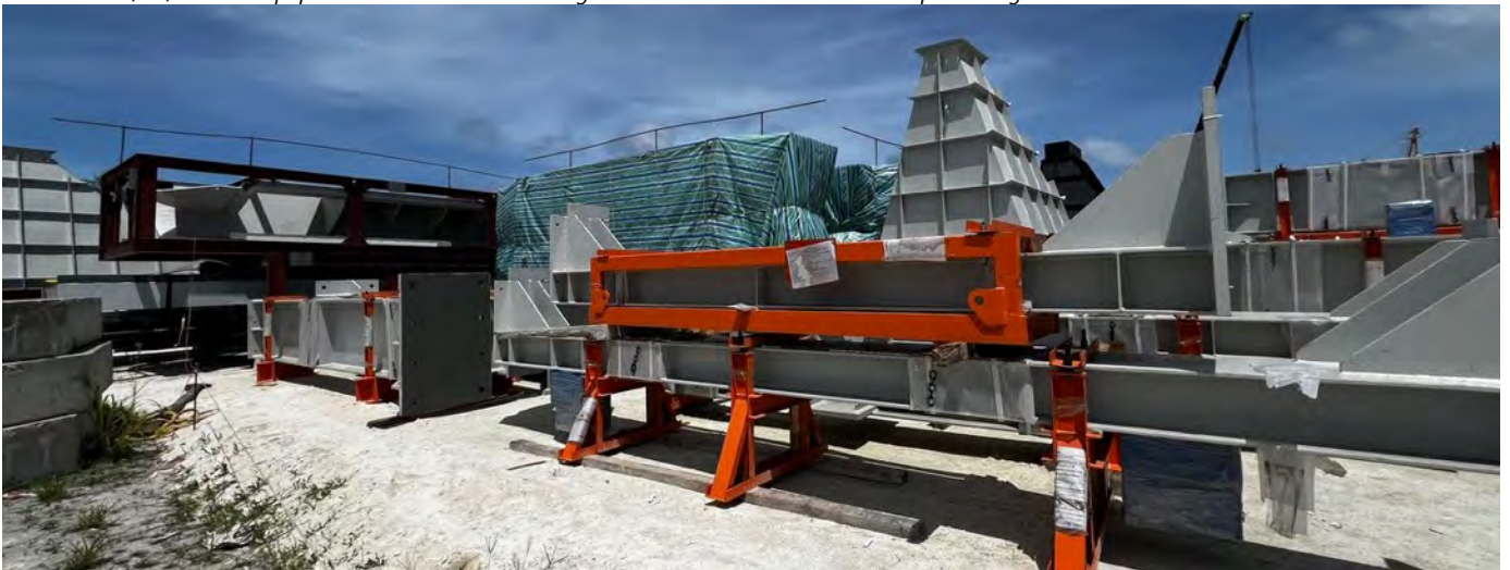
Photo 19 02/05/24 – Steel structure elements delivered to site along with the grate related materials.
