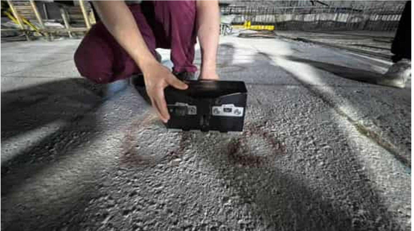
Photo 05 08/04/24 – Non destructive Pulse Echo Ultrasonic test being done on the Bunker slab in Area 1, by third party inspector Falcon Laboratories to check for any cracks, cold joints within the concrete slab.
