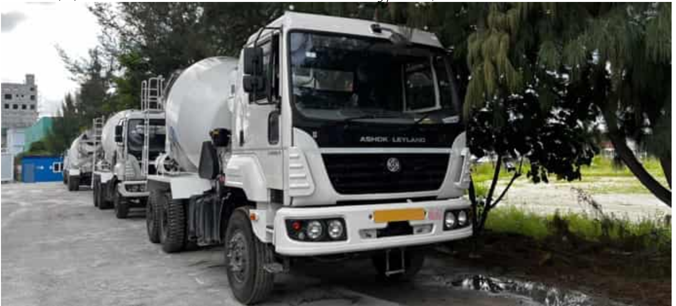
Photo 17 14/04/24 – Concrete mixer vehicles on site, not registered yet however the application made by Villa.
