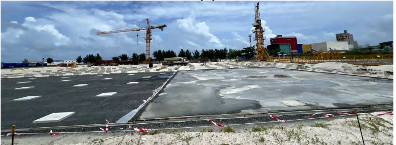
Photo 07 30/05/24 – Main process area construction work is ongoing but slowed down due to material delivery delays..
