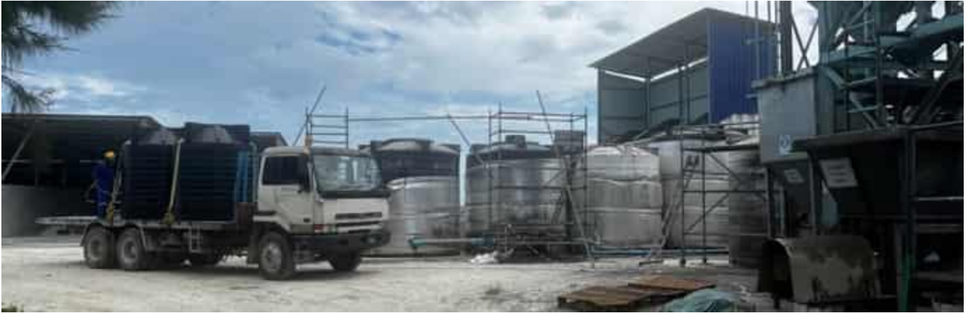
Photo 05 04/04/24 – Batching plant is operational, and water is brought in via truck for the batching plant.
