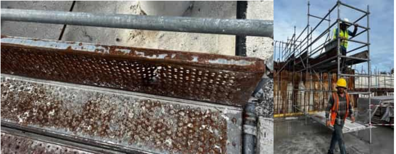
Photo 30 14/04/24 – Rust seen on the scaffolding and panels were asked to be replaced.
