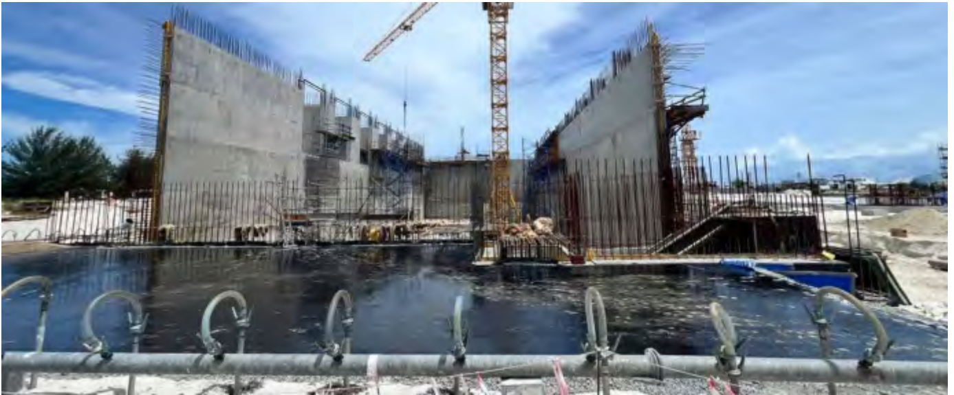
Photo 01 25/07/24– Construction work on the bunker walls continue and additional work as been started adjacent to the bunker area.
