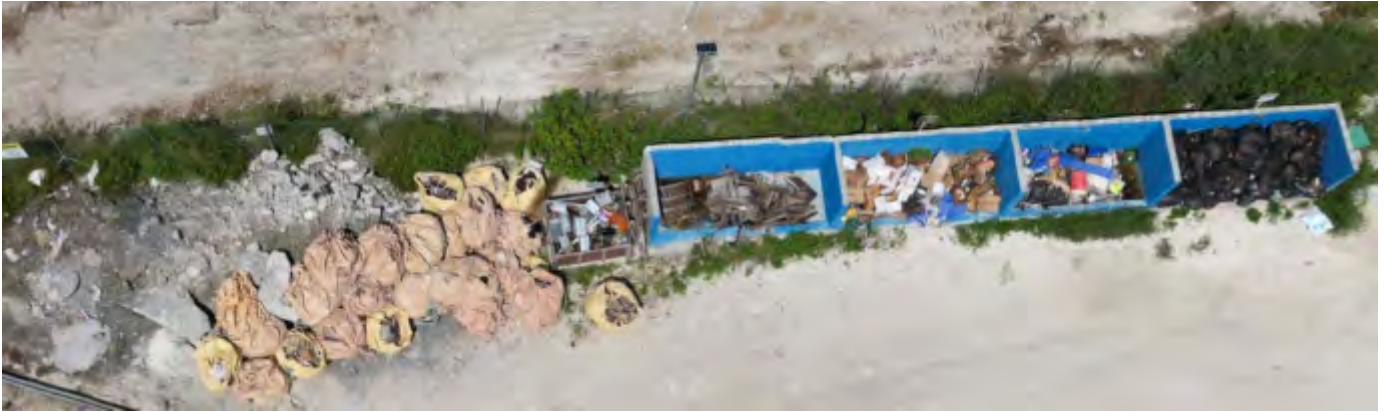
Photo 11 09/07/24 – Waste management area, waste is sorted and removed from site on regular basis.
