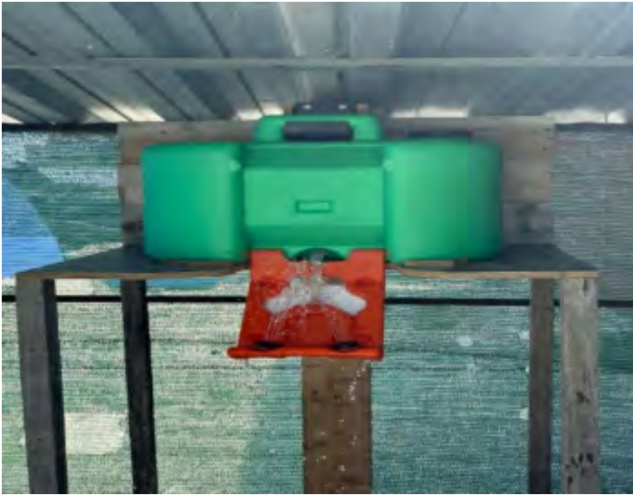
Figure 6: Eye wash station provided near hazardous chemical storage ware house.
