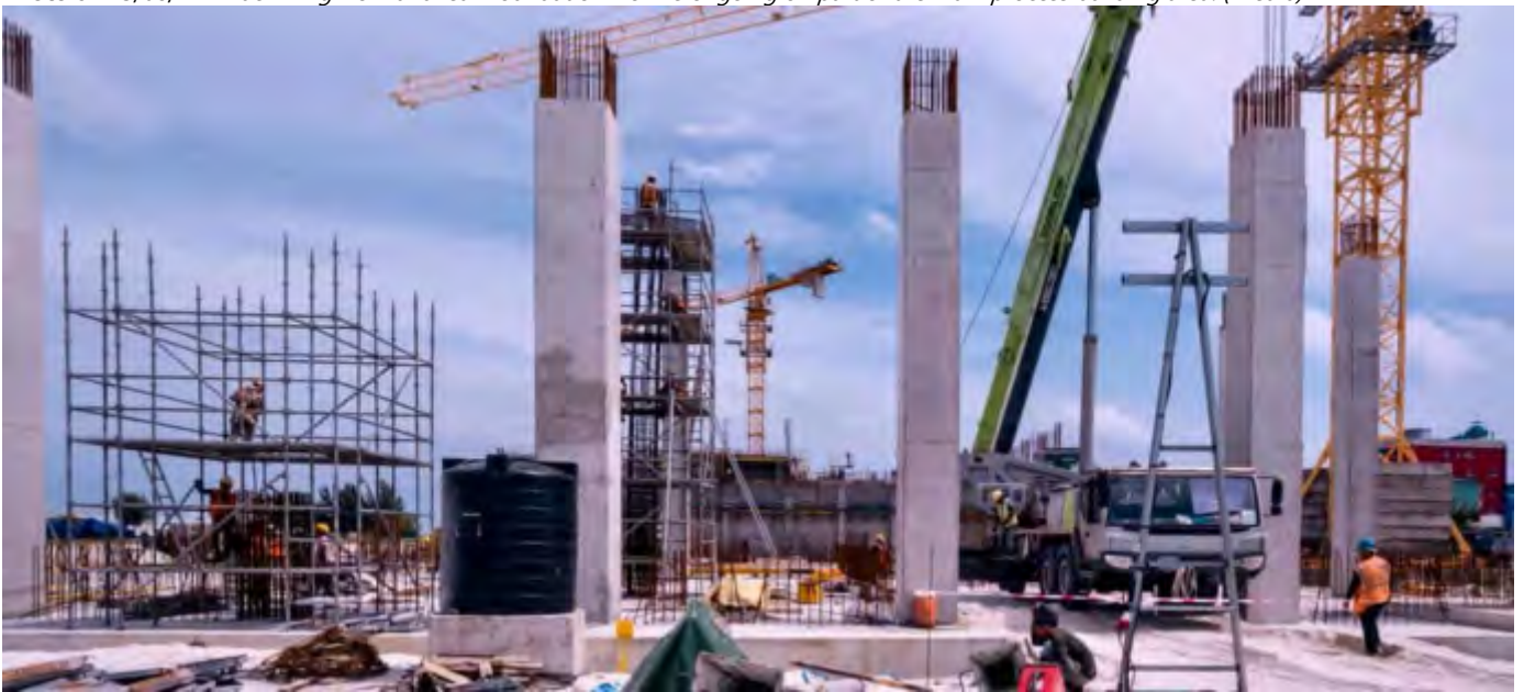
Photo 05 13/08/24 – Ground columns in Area 1 and 2 of Main process building have been cast up to +10.75m height
