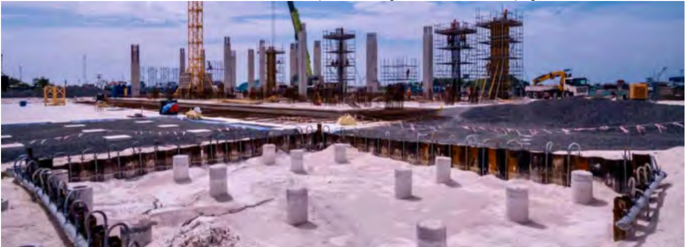
Photo 03 13/08/24 – Turbine Service building area piling and sheet piling works have been completed and ready for excavation, with dewatering system also in place.
