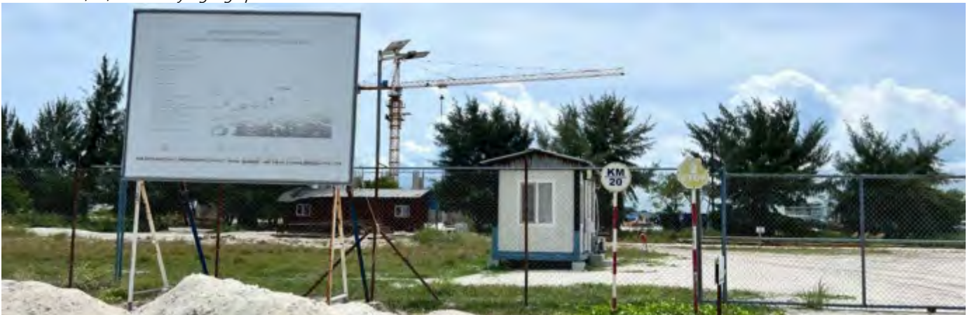
Photo 10 25/07/24– Main project information display board needs to be updated and replaced as soon as possible.
