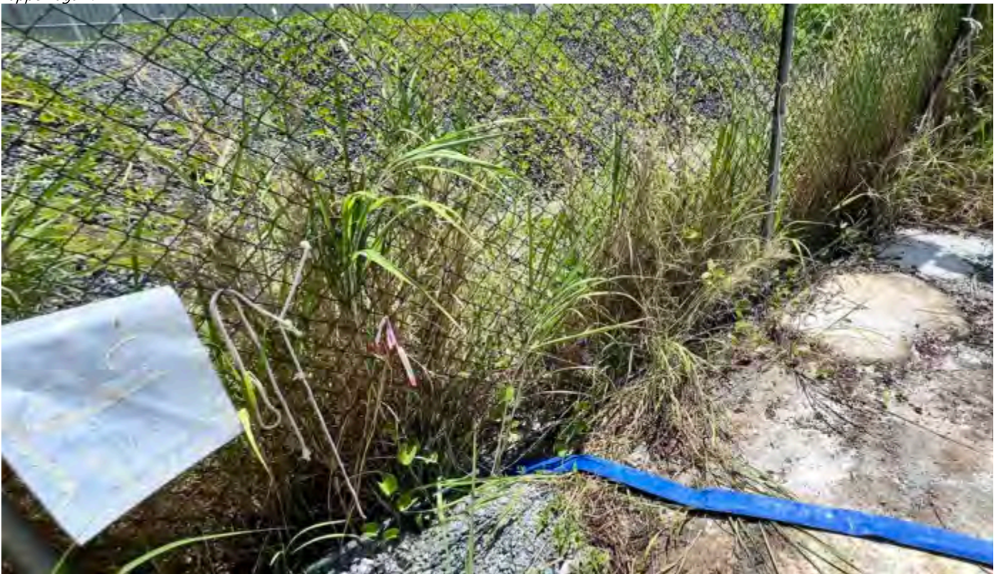
Photo 18 18/07/24– A pump and pipe line was seen from the concrete wash out area retention tank to the adjacent site, this has been brought to immediate attention of the DBO, EPC and Villa subcontractor and instructed to stop this as it is violation of regulations and ensure this doesn't happen again.
