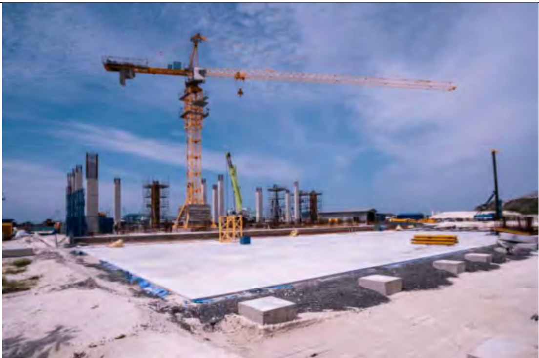
BOILER AREA - NO ACTIVITY
