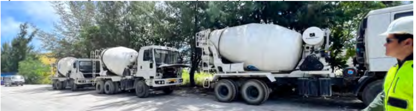
Photo 16 18/07/24– Several concrete mixer vehicles on site, that belongs to the Villa subcontractor are lacking registration, and the process has been started to all vehicle registration in place.
