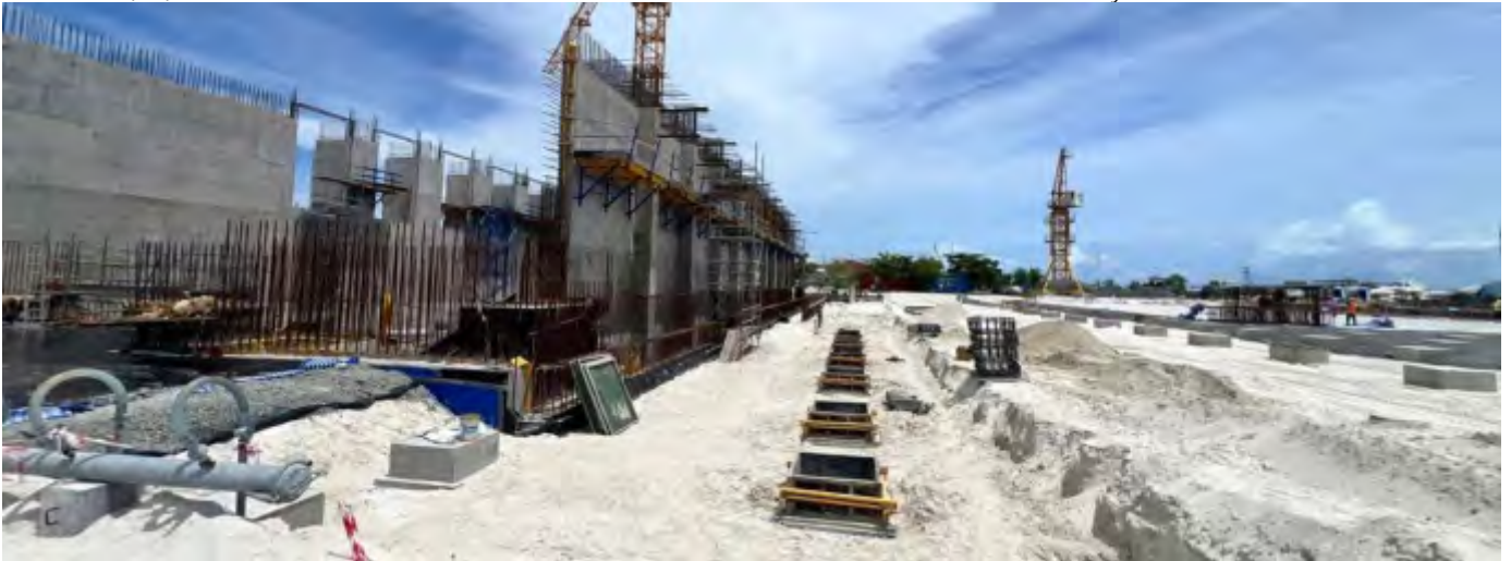
Photo 02 25/07/24 – Pile cap concrete work in progress for the remaining piles caps, after the sheet piles in this area had been removed. (Area 11 & 12)
