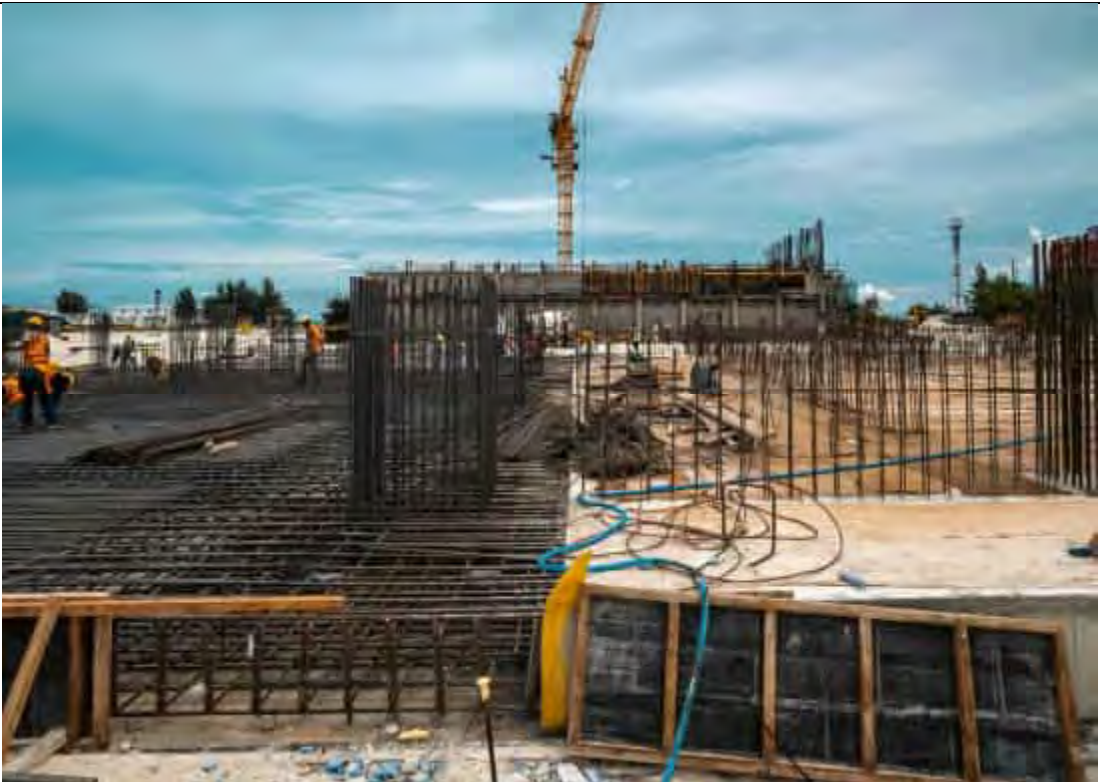
APC AREA - AREA 1 & 3 CONCRETE CASTING FOR FOUNDATION COMPLETED. AREA 2 REINFORCEMENT BAR AND FORMWORK IN PROGRESS.
