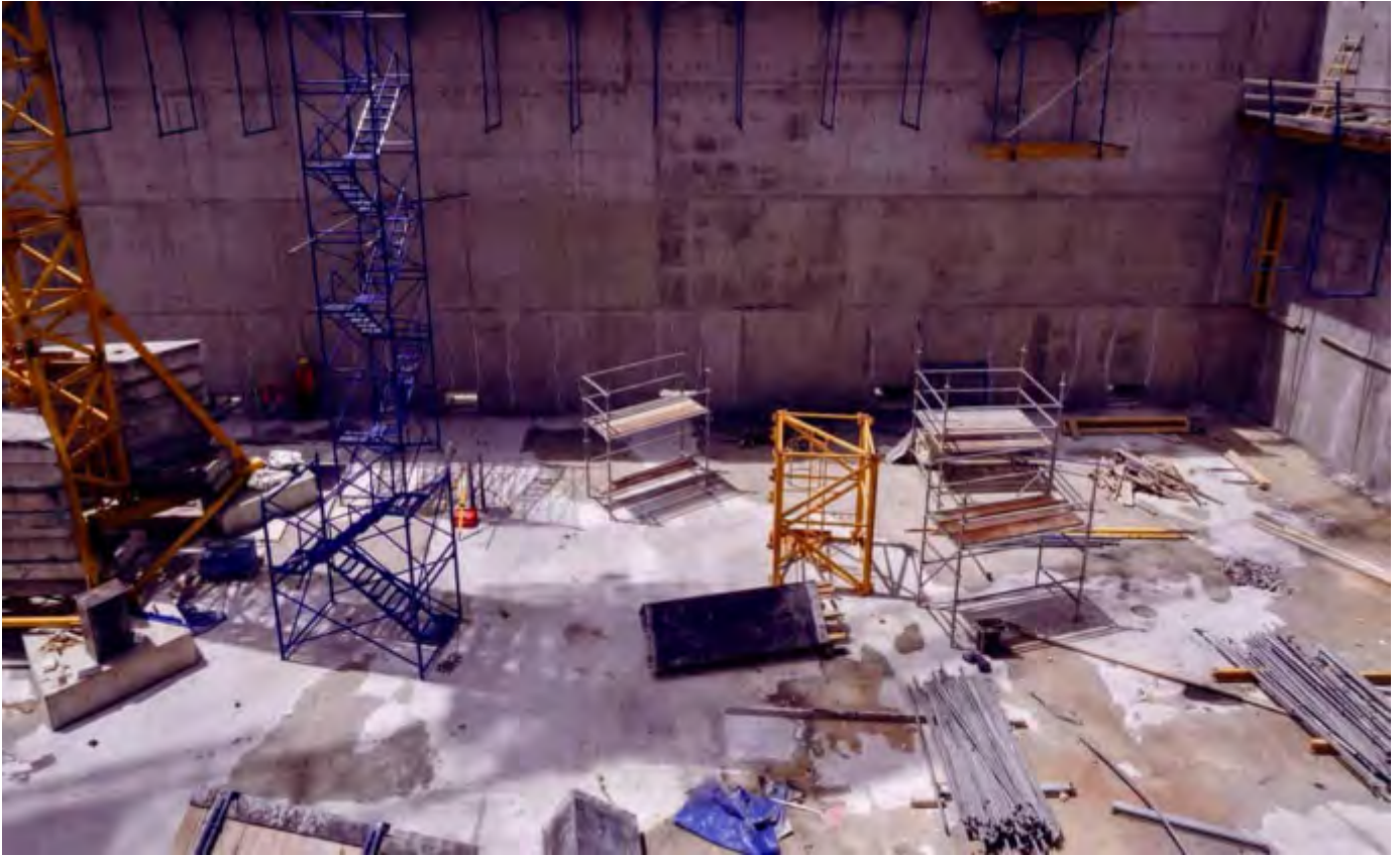
Photo 10 13/08/24 Bunker inside view of Area 1 and 4, crack repair work on Wall D has been completed.
