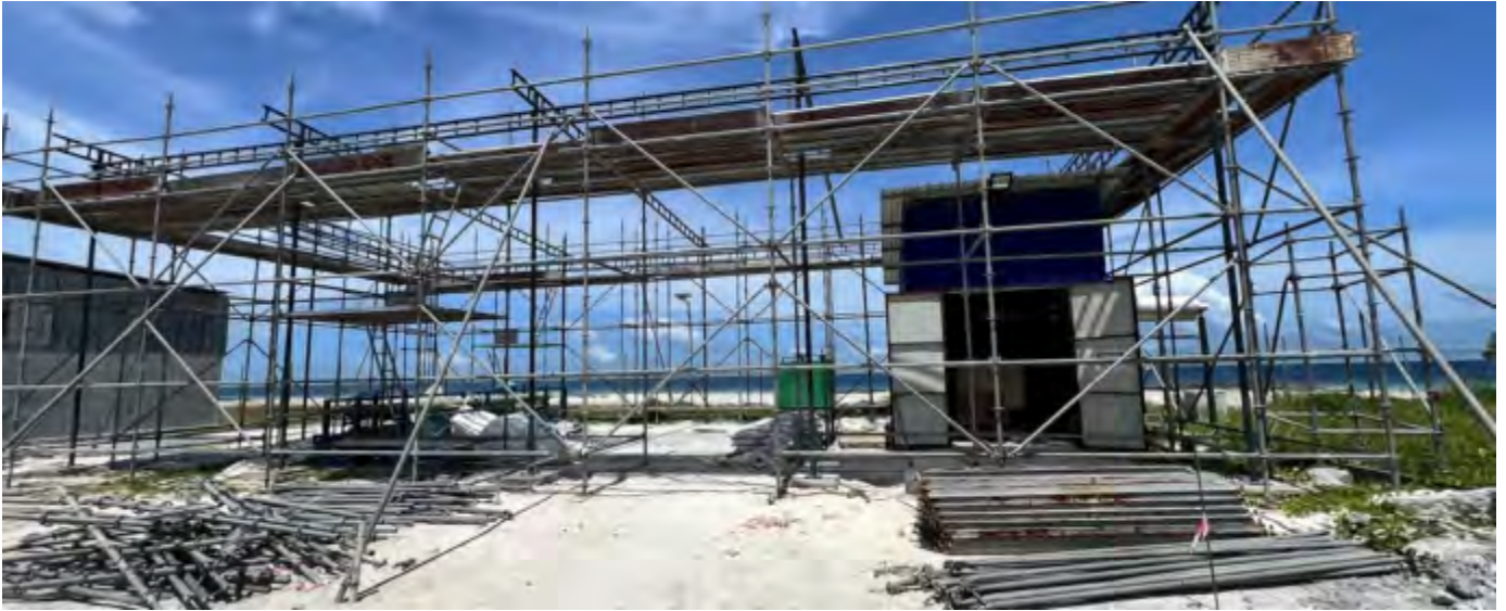
Photo 19 18/07/24– Construction of the desalination plant building is in progress, however permits for borehole, and operation of the plant should be obtained from relevant authorities before operation can begin.
