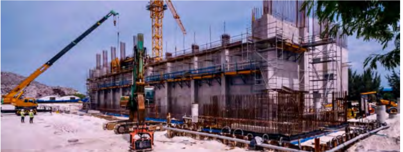
Photo 07 13/08/24 – Bunker walls B,D,C,E,F and G seen on this photo works in progress and expected to finish upto +9.40m this month.
