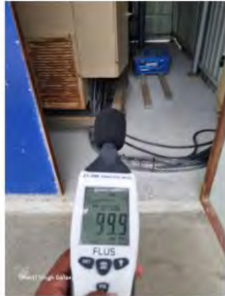
Batching Plant Generator
