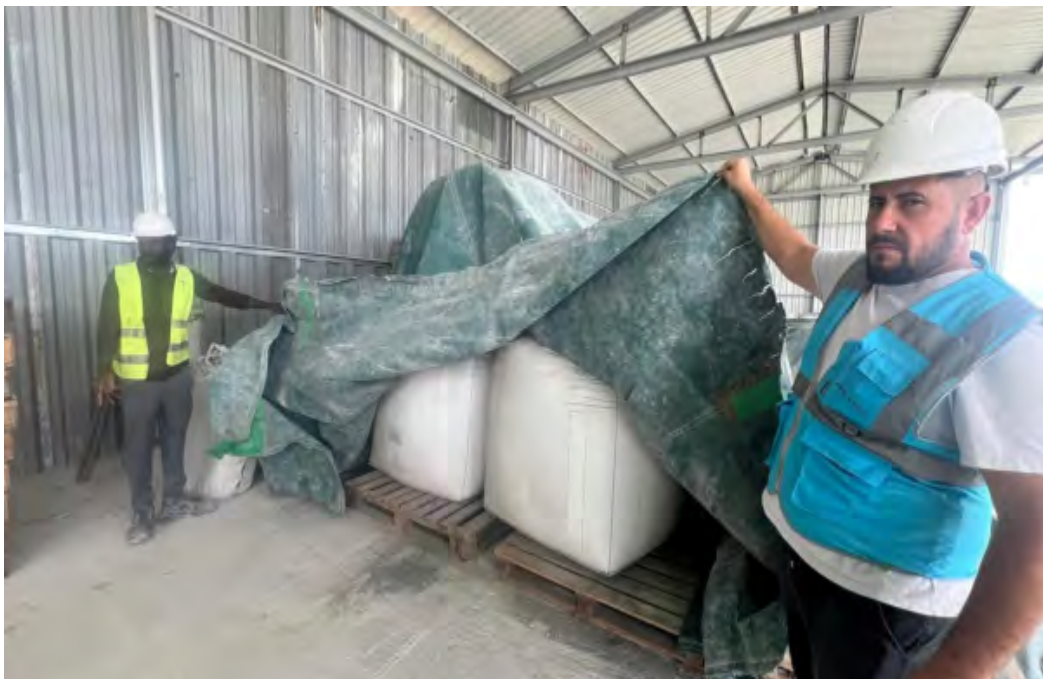
Storage of bags of cement and fly ash to be used in batching plant
