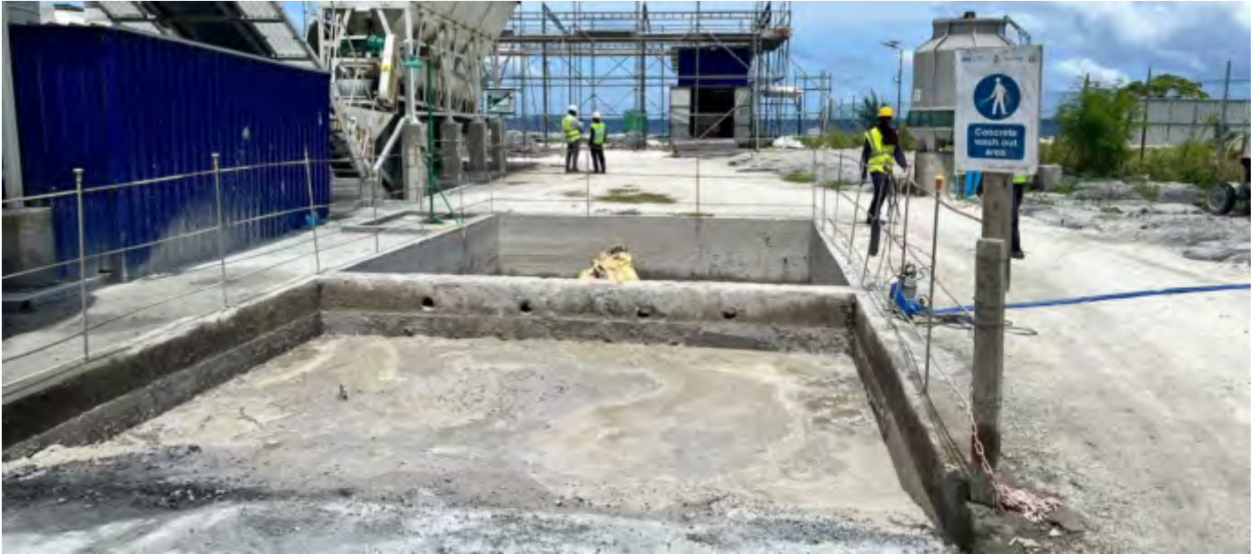
Photo 17 18/07/24– A pump and pipe line was seen from the concrete wash out area retention tank to the adjacent site, this has been brought to immediate attention of the DBO, EPC and Villa subcontractor and instructed to stop this as it is violation of regulations and ensure this doesn't happen again.
