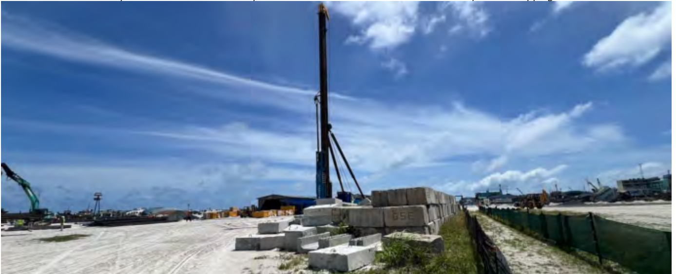
Photo 02 18/07/24 – Some equipment and material remain on site from the spun pile driving work, its advised to remove from site if the material is no longer required.
