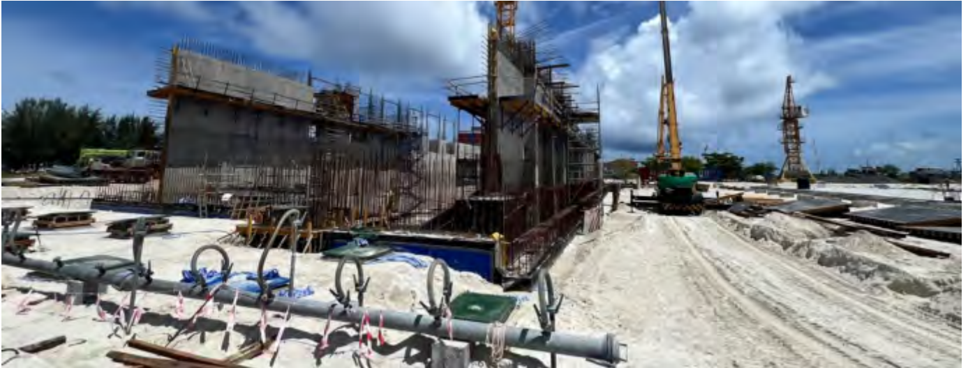
Photo 04 18/07/24 – Sheet pile removal work and backfilling work on going in the area between the main process building and bunker.
