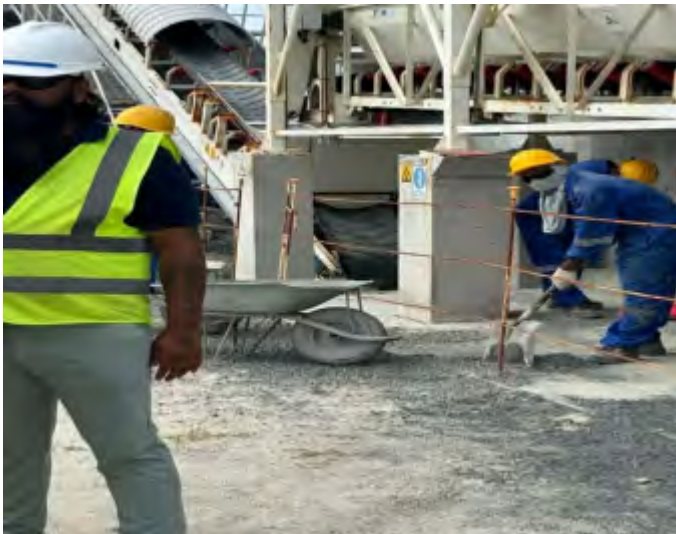
Figure 13: Inadequate Mask found in batching plant area
