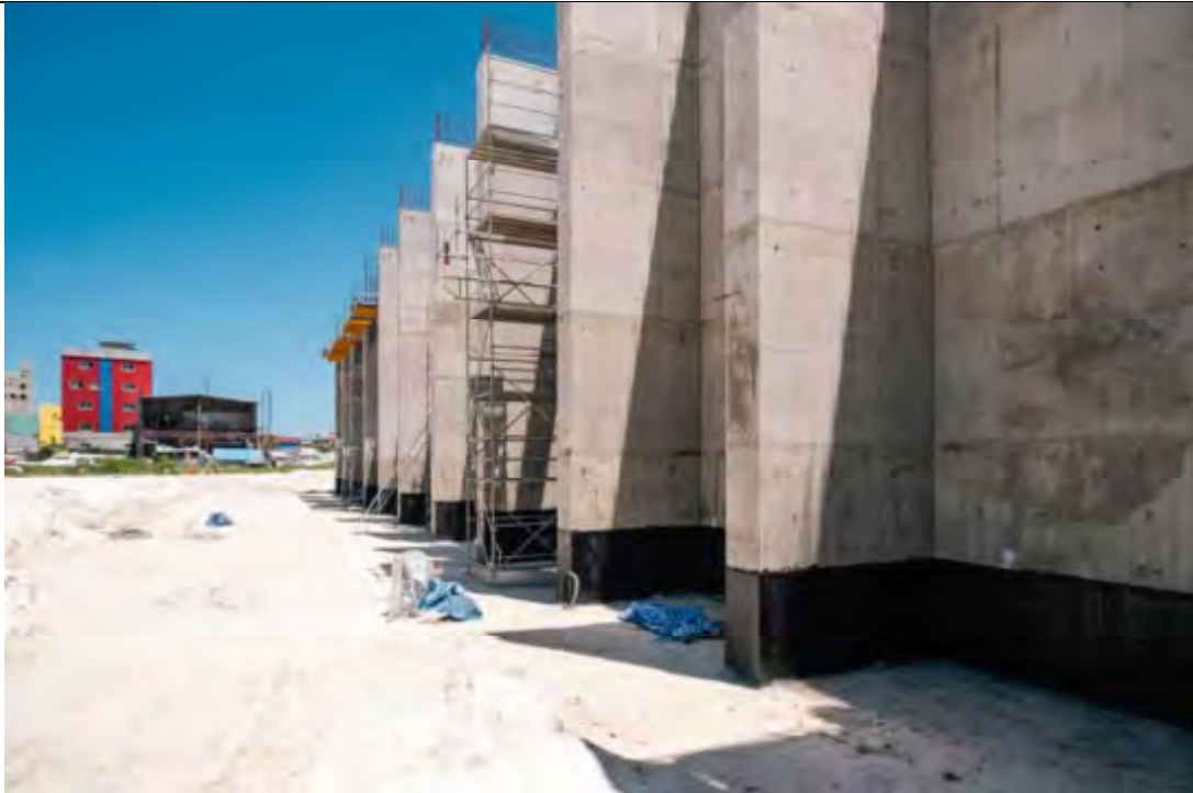
STRUCTURAL BACKFILLING WORK BEHIND BUNKER WALL TO BE RECTIFIED
