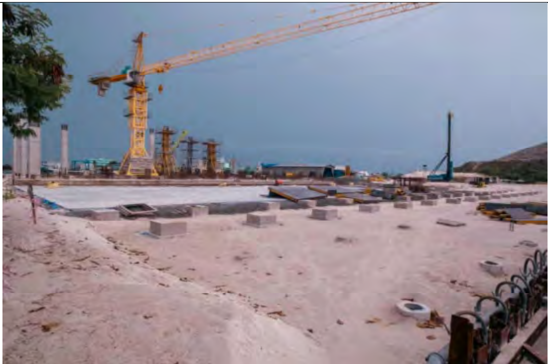
BOILER AREA - NO ACTIVITY
