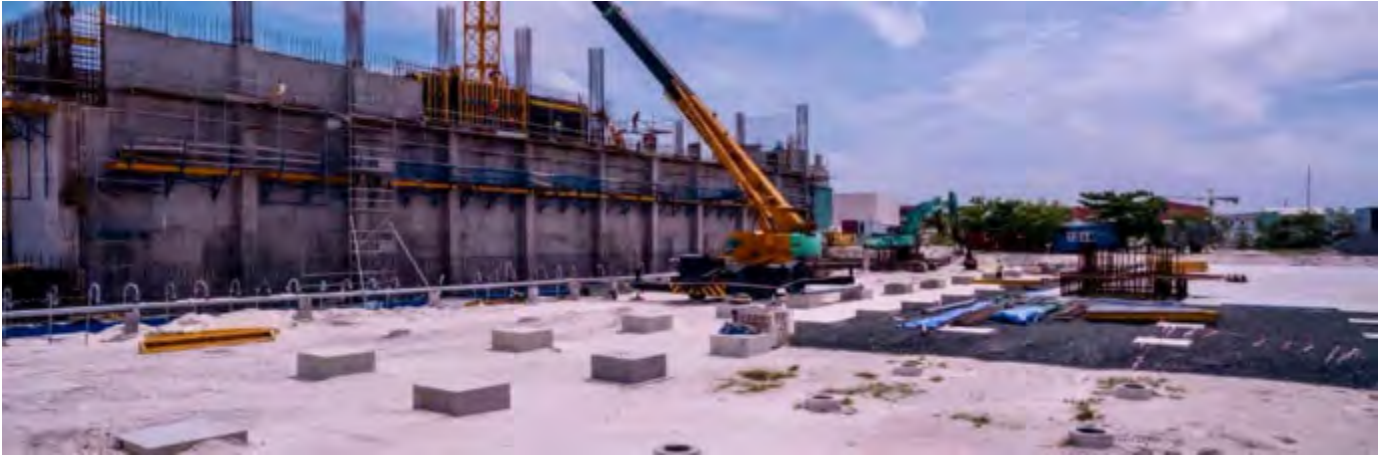
Photo 04 13/08/24 – Backfilling work and lean foundation work is ongoing on part of the main process building area. (Area 6)
