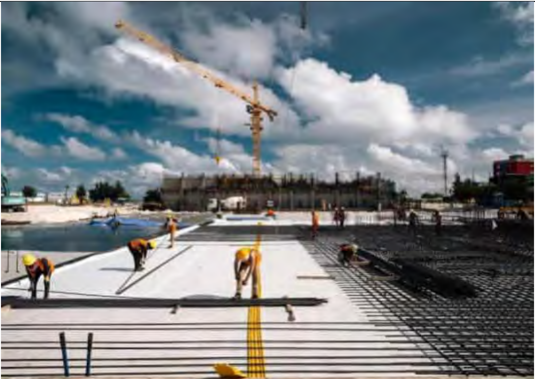
APC AREA - AREA 1 CONCRETE CASTING FOR FOUNDATION COMPLETED. AREA 3 REINFORCEMENT BAR AND FORMWORK IN PROGRESS.
