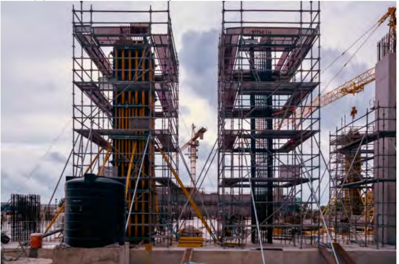
Photo 13 13/08/24– Main process building work Area 2 ground floor columns being made ready for concrete.
