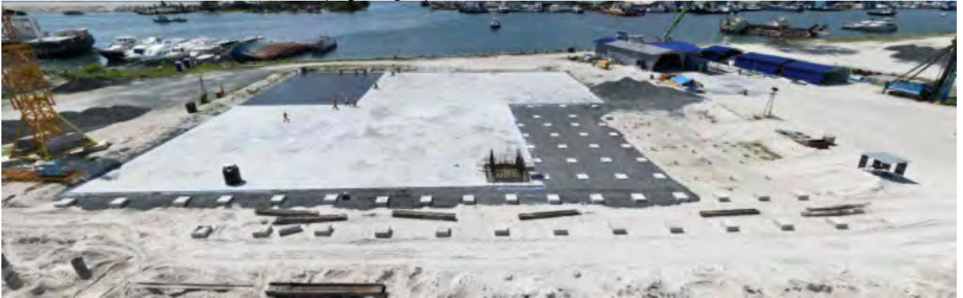
Photo 06 09/07/24 – Backfilling, lean concrete and water proofing work is ongoing in the process building area.
