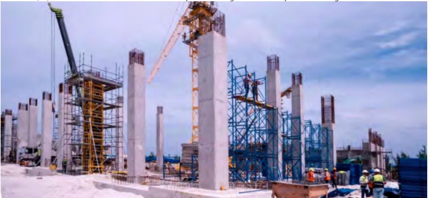
Photo 06 13/08/24 – Ground columns in Area 1 and 2 of Main process building have been cast up to +10.75m height
