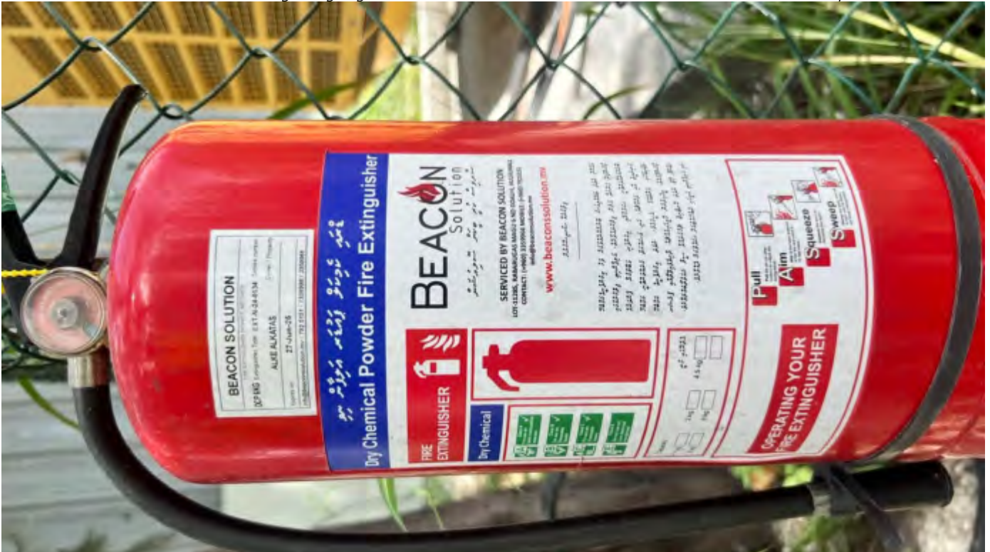
Photo 15 18/07/24– Some of the fire extinguishers still showing expired tests stickers from the third party inspectors, however the EPC assures they have checked and all extinguishers will be checked and verified by the third party inspectors very soon.
