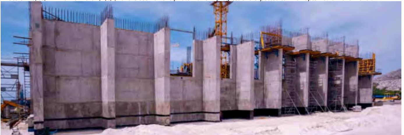
Photo 08 13/08/24 – Bunker walls I and J on this photo works in progress and expected to finish upto +11.35m this month.
