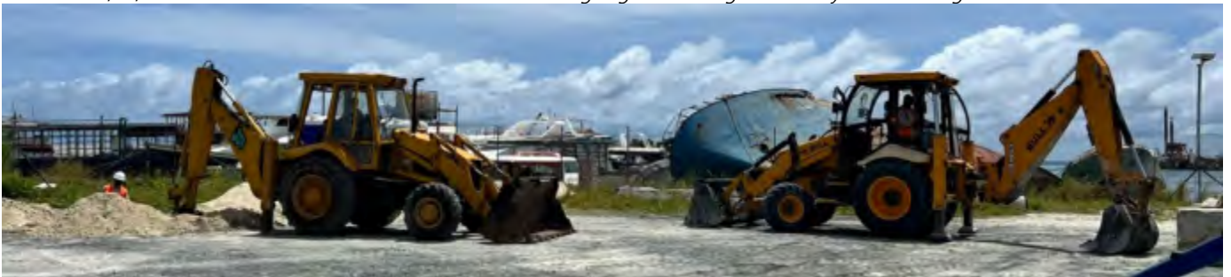
Photo 09 18/07/24– Several heavy machinery in operation doesn't have any visible registration plates, however the EPC assures the vehicles are registered, all registration plates should be installed on vehicles and should be visible as per regulations.
