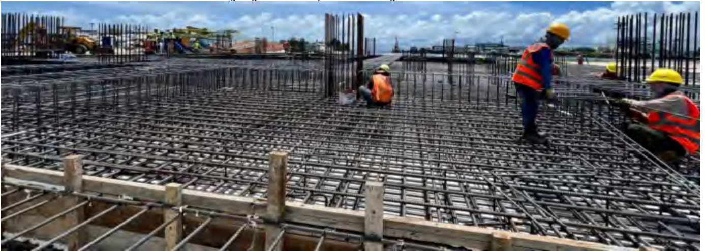
Photo 08 18/07/24 – Foundation slab reinforcement installation is ongoing and is being made ready for concreting.
