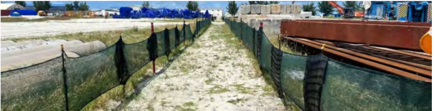
Photo 01 18/07/24– Walkpath to the construction camp to the work area needs to be cleaned and kept free of tripping hazards.
