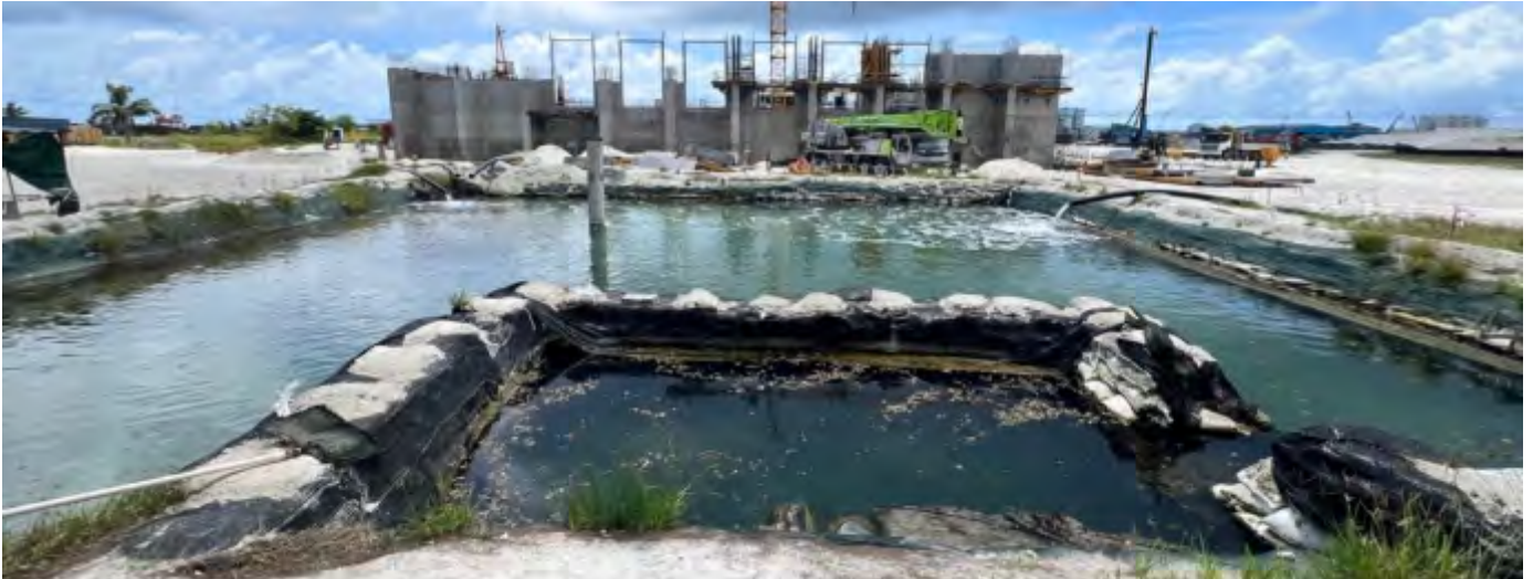
Photo 14 18/07/24– Continous dewatering is ongoing and will continue until all the sides of the bunker walls have been completed.
