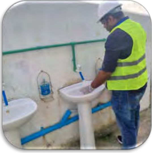
Supply Water for Camp and Construction Sampling
