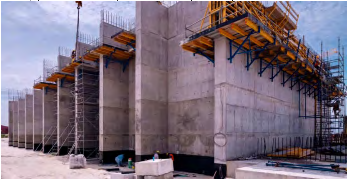
Photo 09 13/08/24 – Bunker walls I and J on this photo works in progress and expected to finish upto +11.35m this month. Walls A and H to be completed up to +14.10m height this month.
