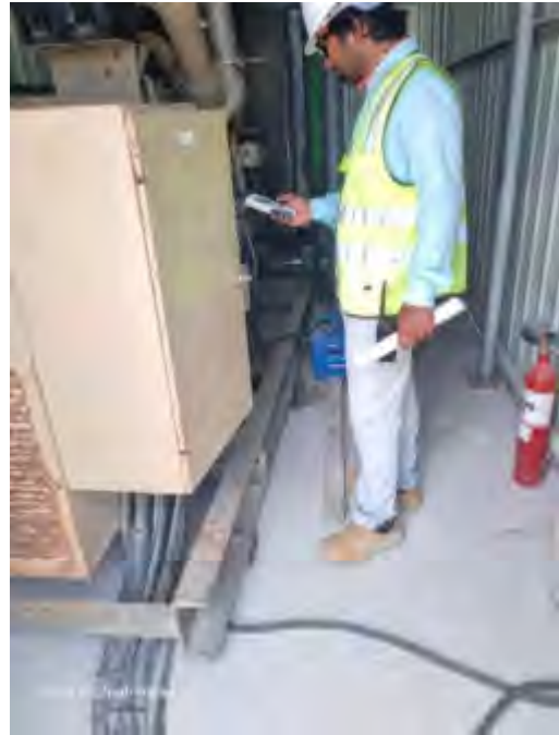
BATCHING PLANT GENERATOR
