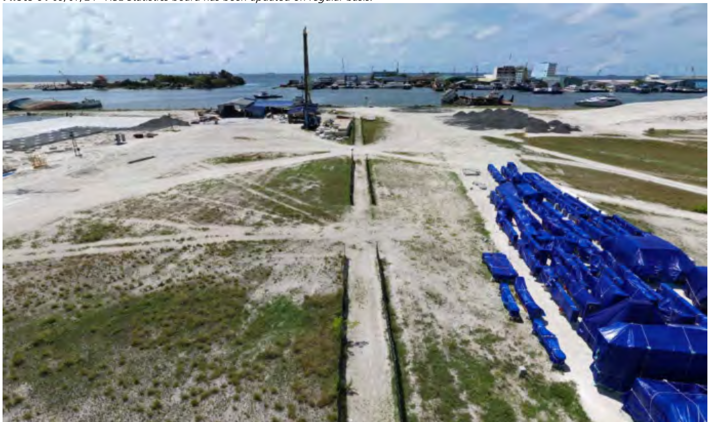
Photo 02 09/07/24 – The walkpath from the construction camp to the construction area is kept clean and free of tripping hazards.
