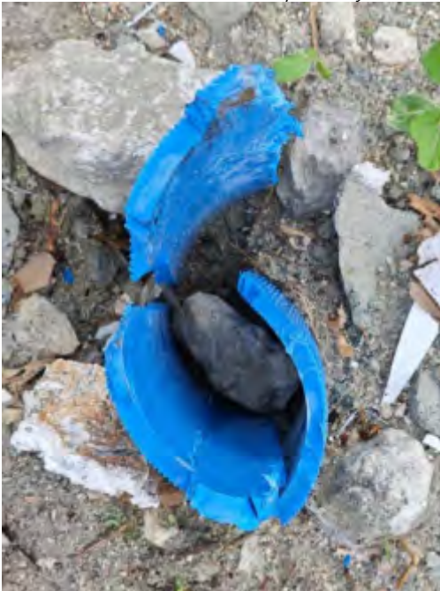
Photo 12 25/07/24– The water sampling well GW6 near the landfill has been damaged and needs to be repaired as soon as possible.
