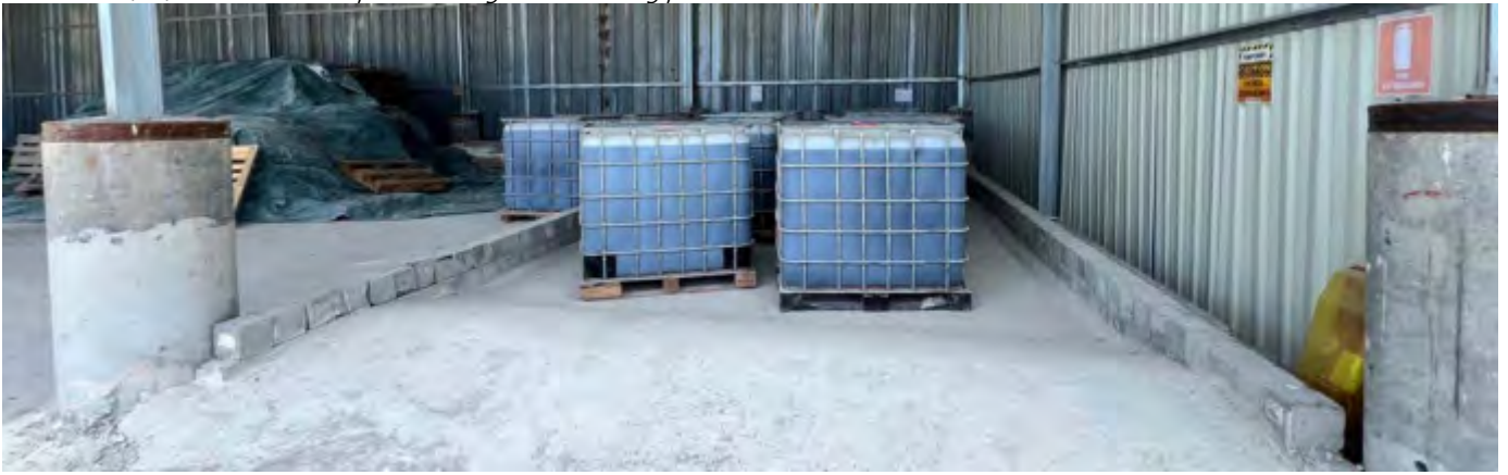
Photo 08 25/07/24 – Chemical storage area in the batching plant area requires proper bund wall for retention in case of accidental spillage.
