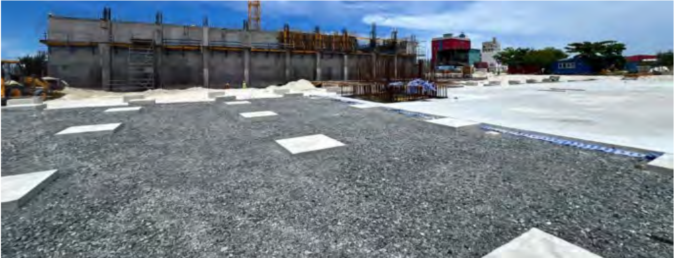
Photo 04 25/07/24 – Backfilling work and lean foundation work is ongoing on part of the main process building area. (Area 8)
