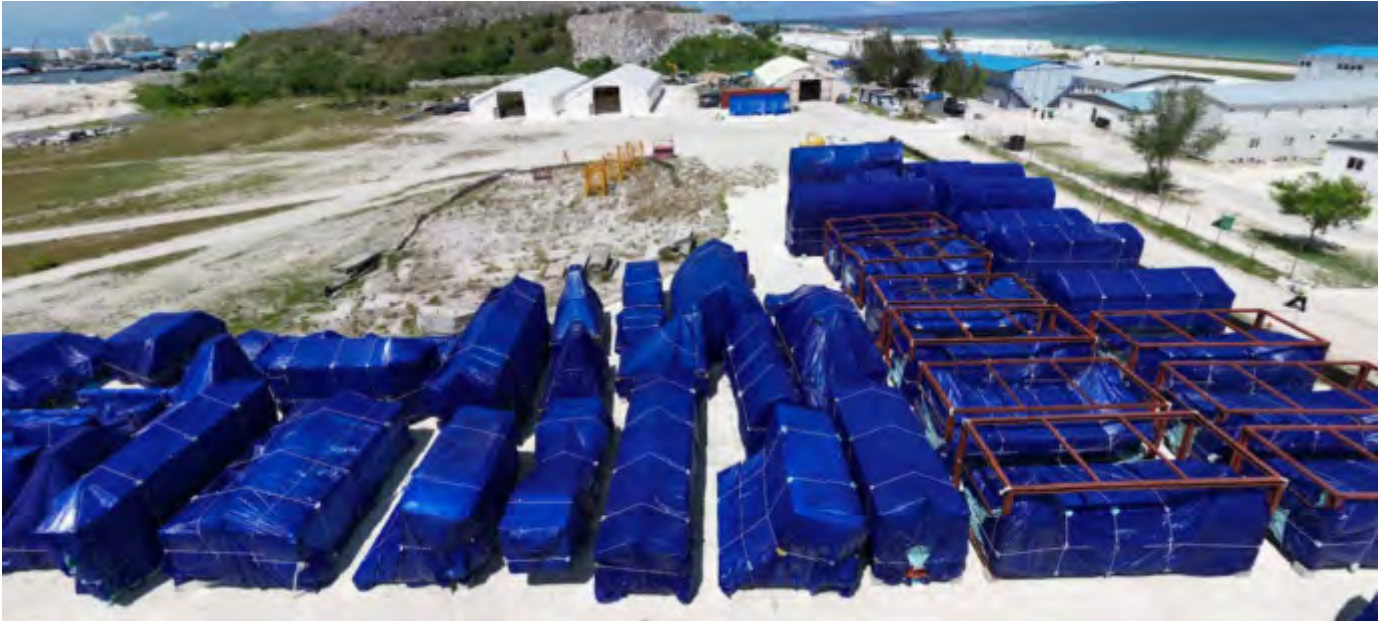
Photo 03 09/07/24 – CNTY delivered the grate parts and are stored on the site laydown area and covered with several sheets of canvas to protect from the elements.
