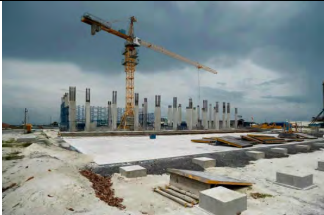
BOILER AREA - NO ACTIVITY
