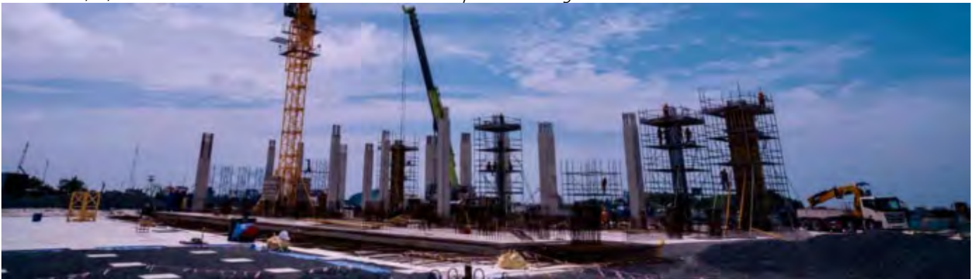
Photo 02 13/08/24 – Ground floor column concretes works in Main process building work area 1,2 and 3 is in progress.
