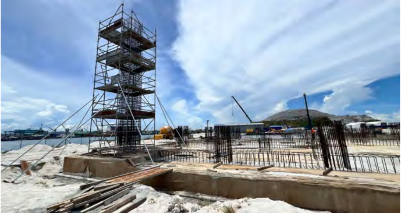
Photo 06 25/07/24 – First column in the main process building area 1 is being made ready for concreting.
