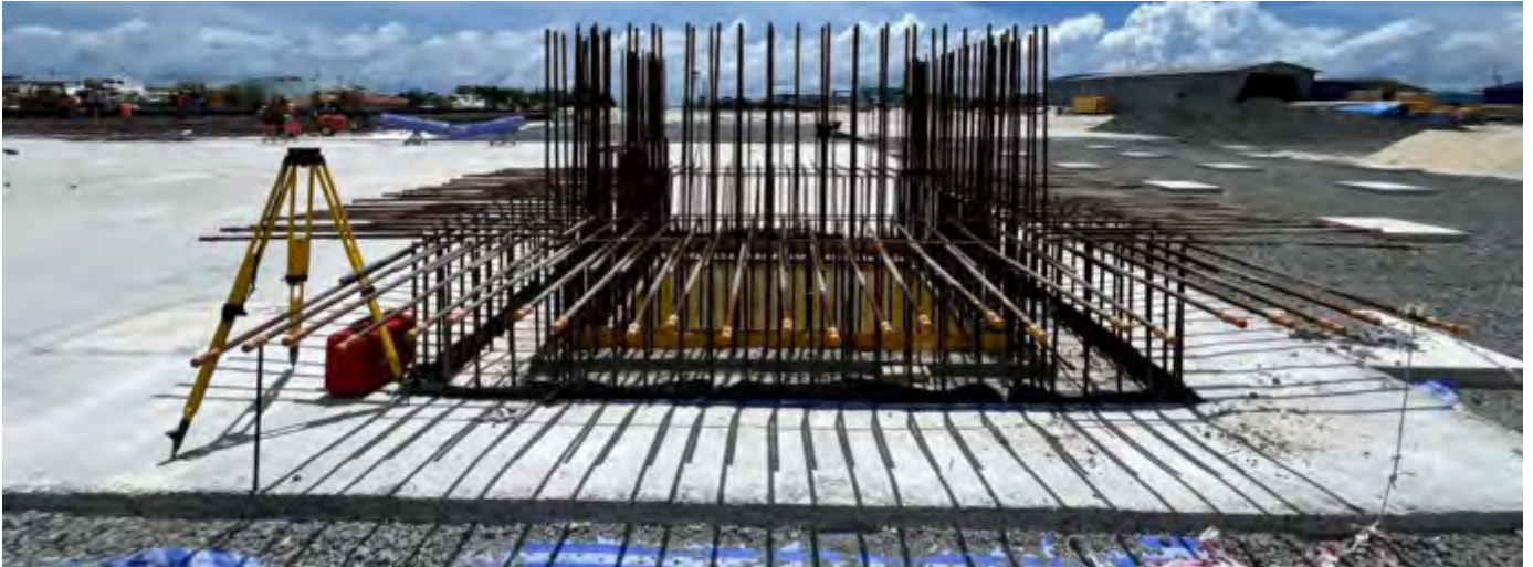
Photo 07 18/07/24 – Lift foundation work is on going in the main process building area.
